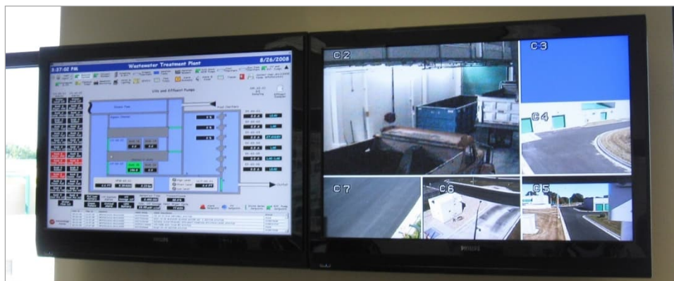
Fond du Lac WPCF SCADA and Security 47-inch LCD monitors.
