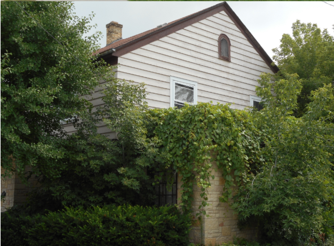
306 Northern Ave (Raze or Repair – walls, floors, ceilings, doors, windows, tuckpoint foundation, Roof, fascia, soffit, plumbing, HVAC, elec, stairs, stoop, gutters, paint, clean, etc)
