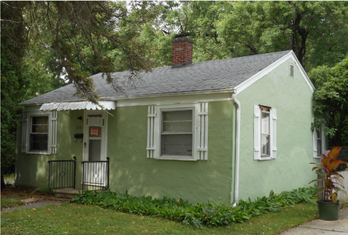
216 Garfield Street (Raze or Repair - deteriorated walls, windows & doors, tuckpoint foundation, plumbing & elec, clean, smoke detectors, & driveway)
