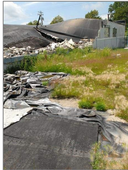
with partially collapsed roof.
