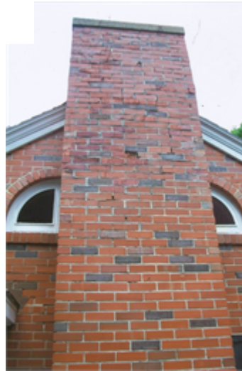
Dane County. The brick on this chimney has experienced severe deterioration - the brick has shifted, cracked and spalled. Source: WHS - Historic Preservation - Public History.
