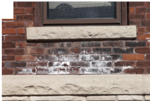
Madison, Wisconsin. Efflorescence can be found on all types of masonry walls - here the efflorescence is evident on the brick surface below the window. Source: Photographer Mark Fay.
