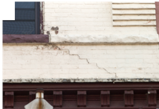
Madison, Wisconsin. Even though this is brick building has been painted, the joint cracking is evident. Source: Photographer Mark Fay.
