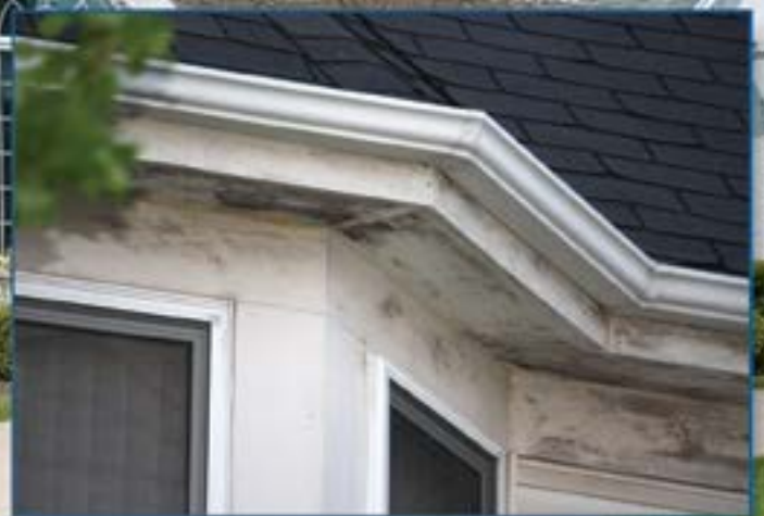
Wood Soffits require cleaning, scraping and painting
