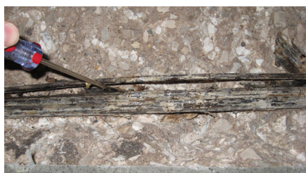
Screwdriver test that identified a loose wire in the button-head tendon bundle
