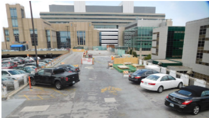
Severe deterioration on roof level
