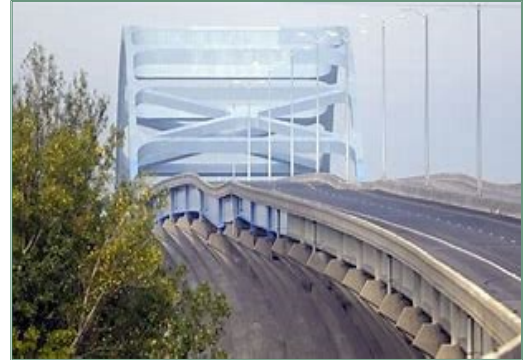
Leo Frigo Bridge Damage
