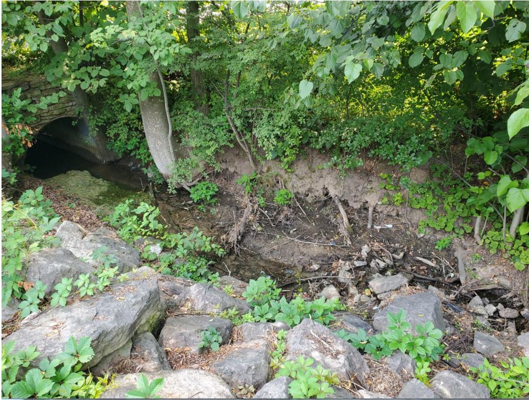
Slight bank erosion north of the driveway culvert servicing 1004 LaCount Road.
