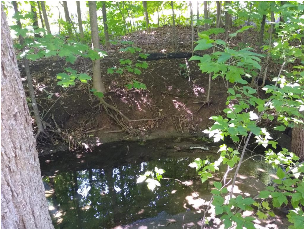
Natural erosion occurring along stream bank within 1024 LaCount Road property.
