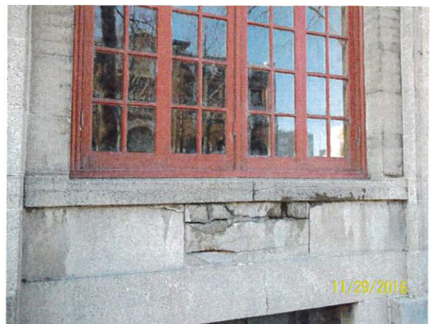
Damaged stone under window sill
