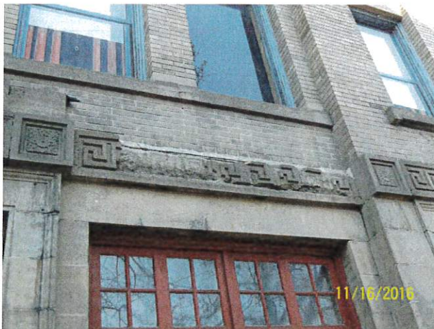
Damaged precast belt course
