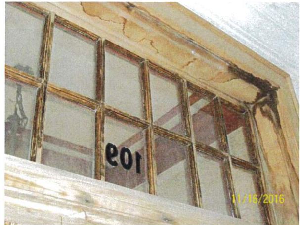
Water damage at entry transom
