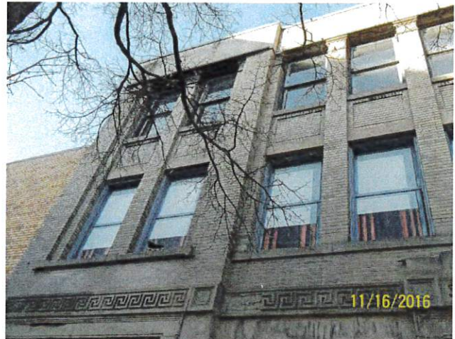
Note damage to window and belt course
