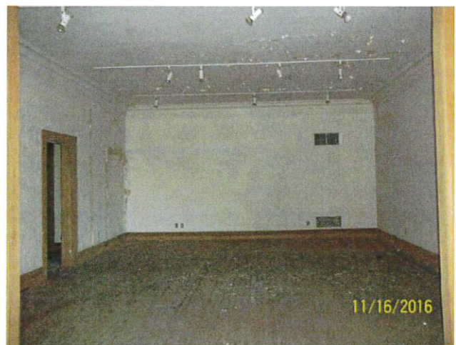
Peeling ceiling paint at chapel
