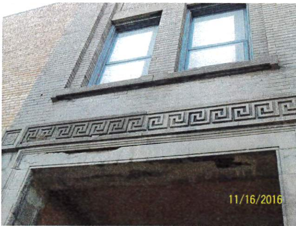
Damaged precast at alley
