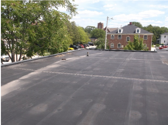
Sanitary vent & roof drain
