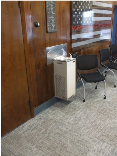
Electric water cooler- meeting room
