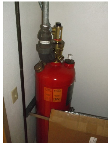
Ansul Halon 1301 – IT room
