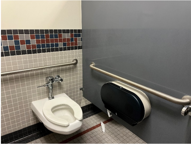
1 st floor Women's – missing vertical grab bar
