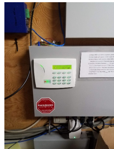
Card access system
