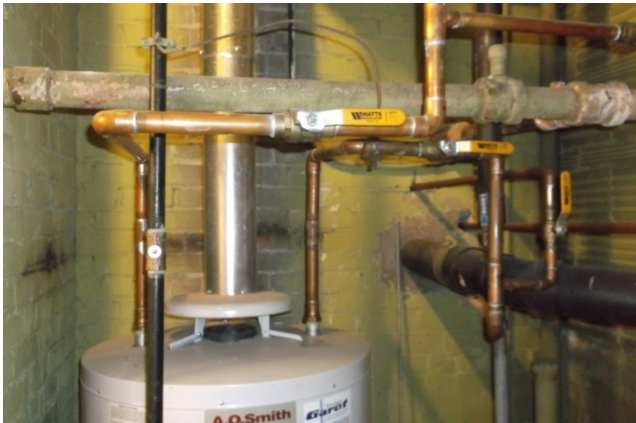
Hot/cold water piping at water heater
