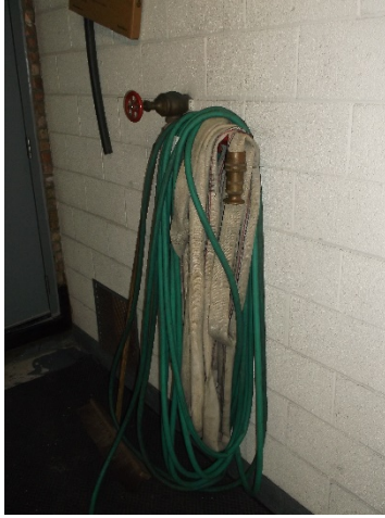
Hose valve – penthouse
