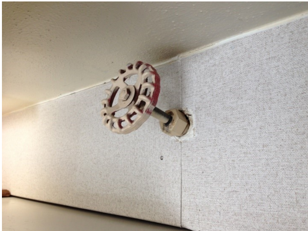
Wall built over valve
