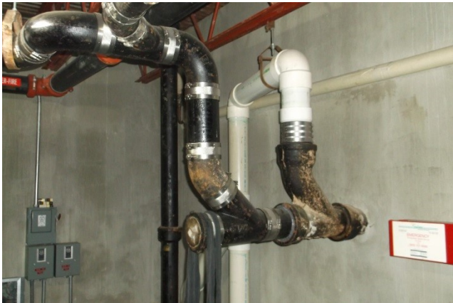
Sanitary piping (cast iron & PVC)
