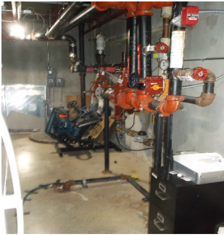
Fire protection riser
