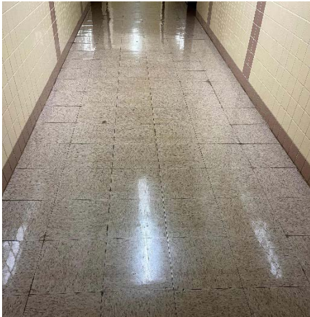
Dirt at center of corridor and edges of tiles
