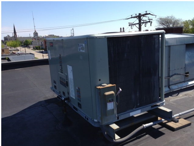
Roof top air unit
