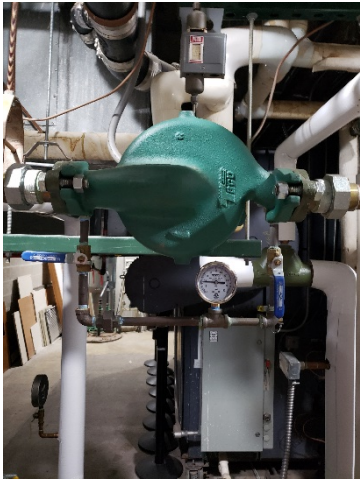
Hot water pumps
