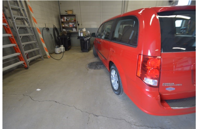
Cracked slab at garage (Note S1)
