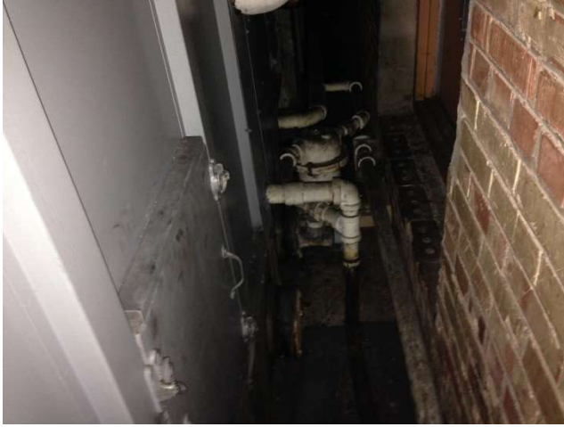
AHU-1 steam coil
