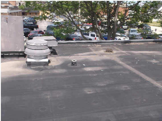
Sanitary vent & roof drain
