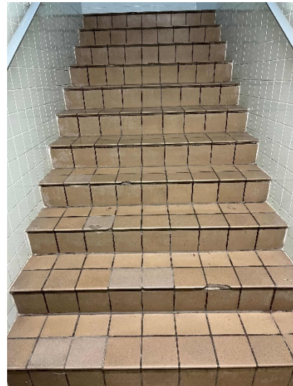
Chipped tiles at south stair
