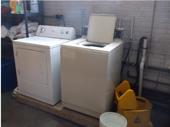
Washer/dryer in garage bay
