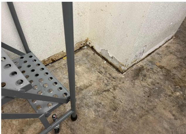
Deteriorated base at high-density storage
