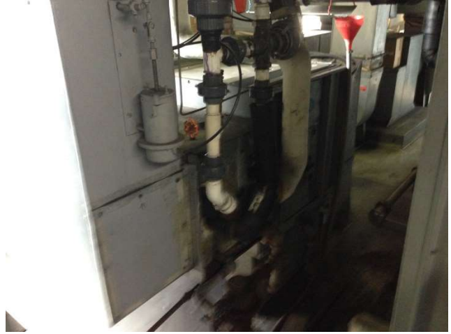
AHU-2 and 3 coils
