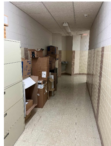
Eliminate combustible storage in corridor
