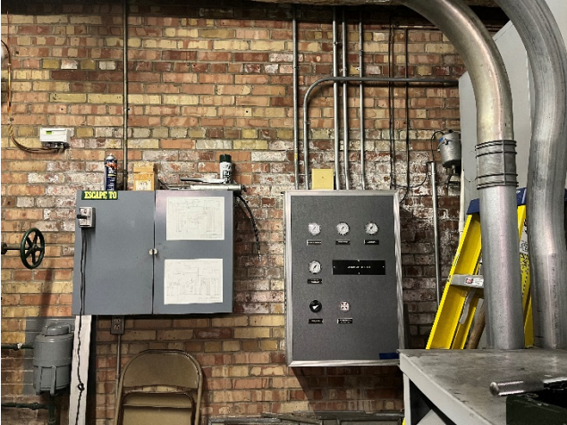
Effervescence on west wall
