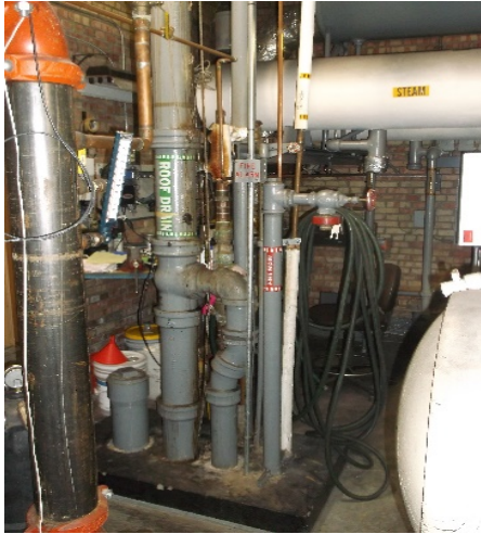
Vent, water piping in penthouse
