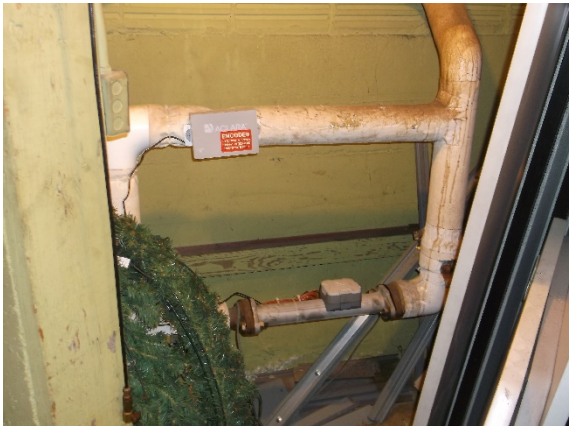
Water service, water meter with by-pass
