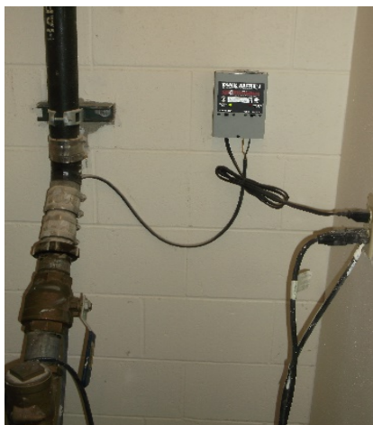
Elevator – high water alarm
