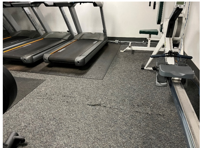
Ripped carpet at cardio room
