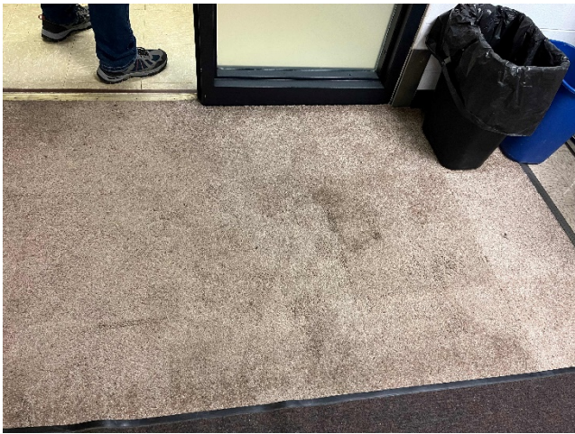
Worn, stained cut-pile carpet
