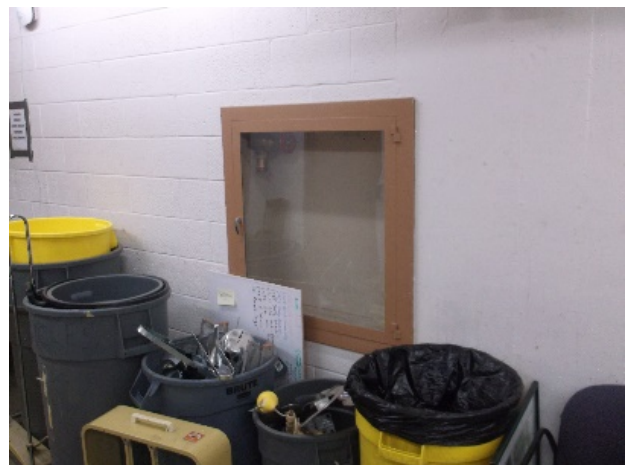
Valve cabinet - basement
