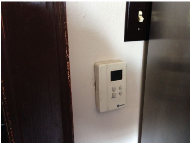
Typical thermostat (This one too close to fridge)
