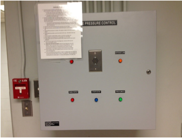
Firing range control panel
