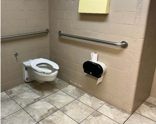
Peeling paint from glazed block
