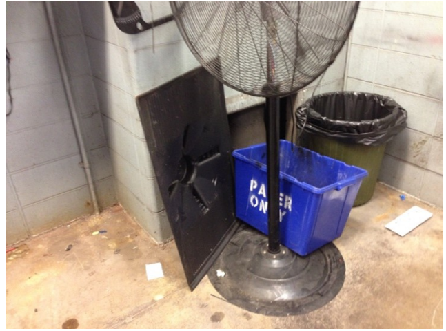
Garage exhaust vent (behind storage)
