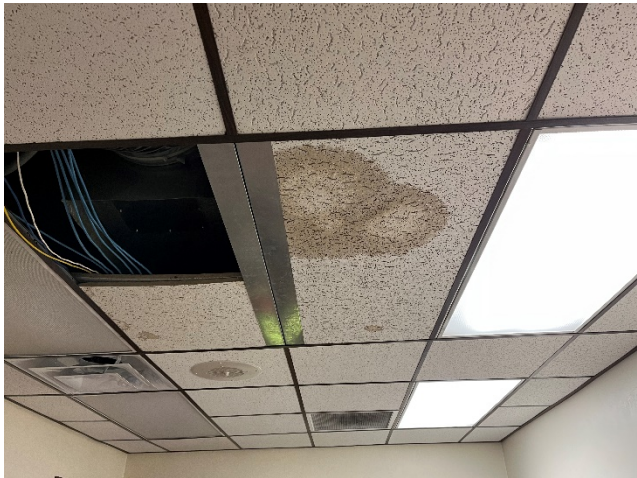
Missing and stained ceiling tile
