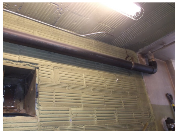
Sanitary piping – boiler room
