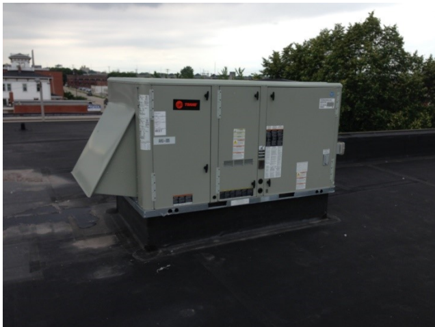
Training room air unit
