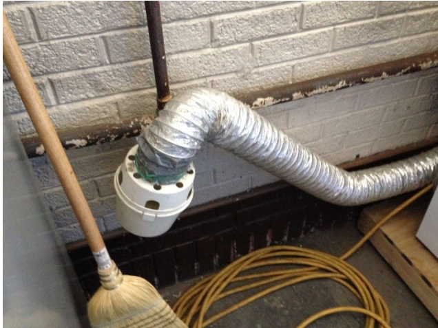
Dryer vent (indoors)
