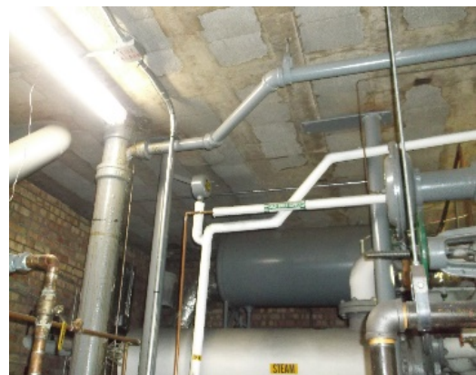
Cast iron vent piping
