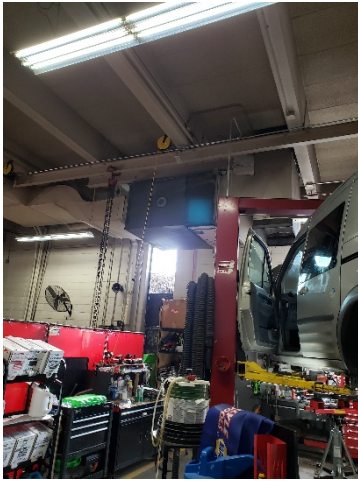
Garage make-up air unit
