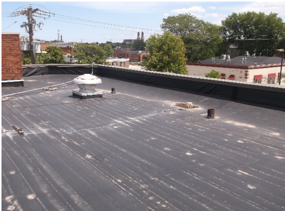
Sanitary vent & roof drain
