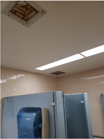
Exhaust grille (degraded)
