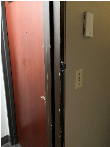
Chipped paint at basement door frames
