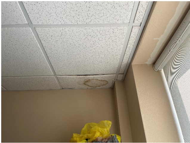
Damaged ceiling tile – adjacent to IT room
