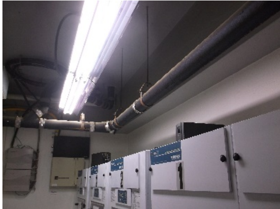
Sanitary piping over evidence dryers
