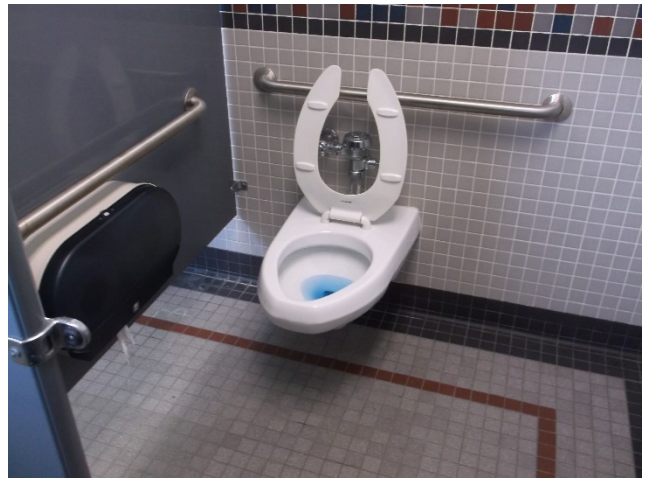
1 st floor Men's – missing vertical grab bar
