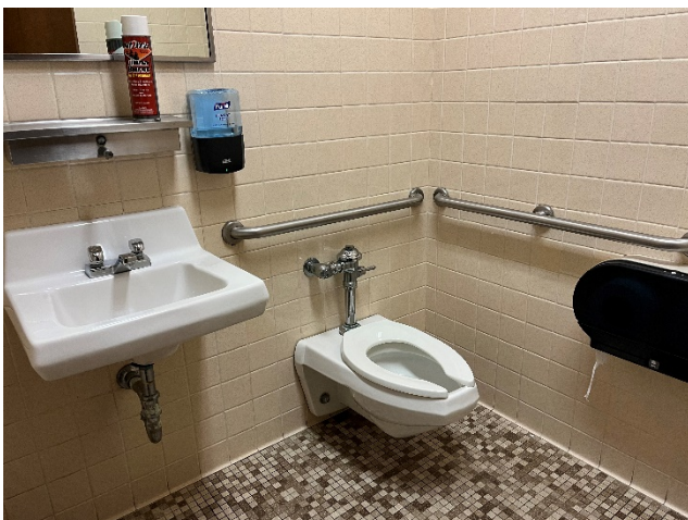
1st floor unisex toilet room – missing vertical grab bar
