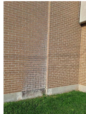
Efflorescence on brick
