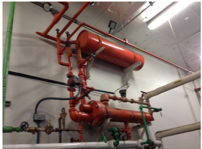
Basement hot water system
