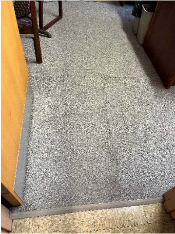
Bubbled carpet at NE office
