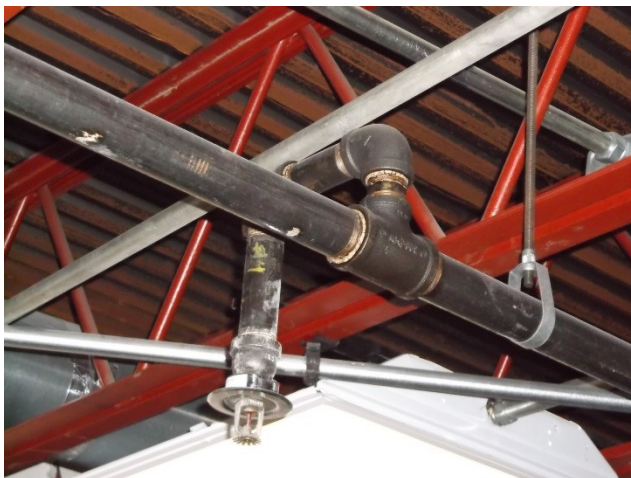
Pendent sprinkler head too far from ceiling
