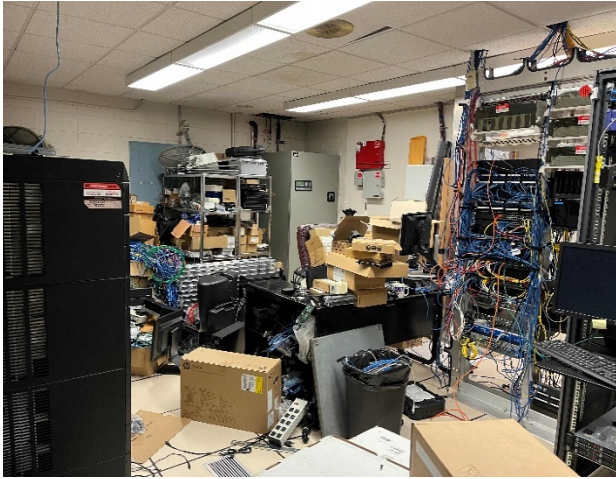
Basement IT room – needs egress route
