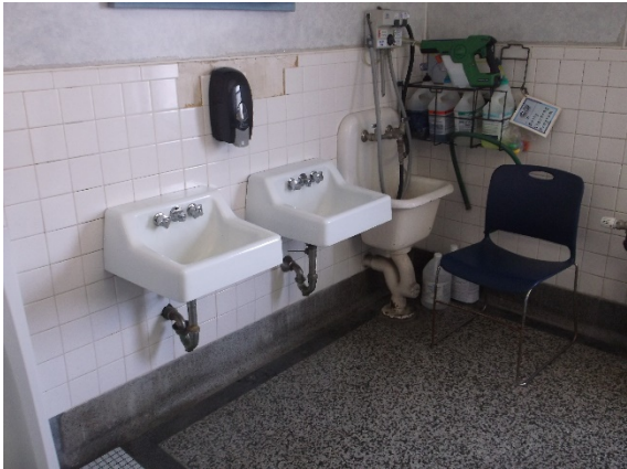
Lavatory sink – men's
