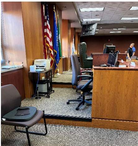
Council platform not accessible
