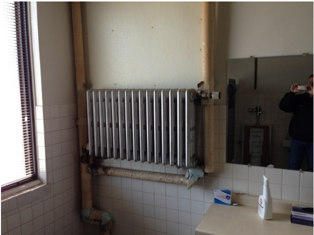
Radiator at women's toilet
