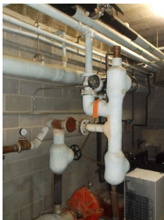
Storm and water piping
