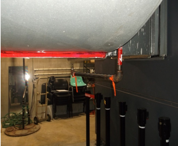
Sprinkler head under duct
