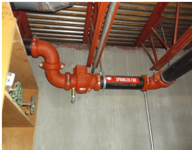
Flow direction points the wrong direction
