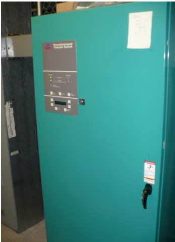
Automatic transfer switch
