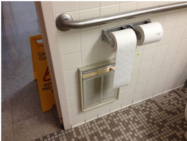
Electric heat at stairs and toilets
