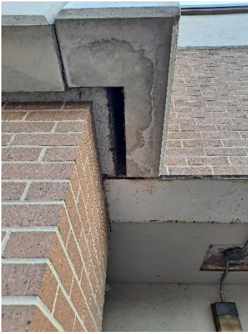
Gaps under precast concrete panels
