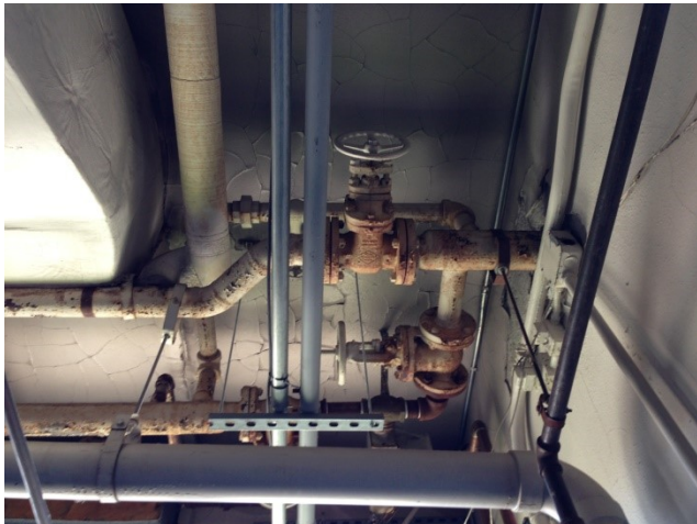
Uninsulated pipe (typical)
