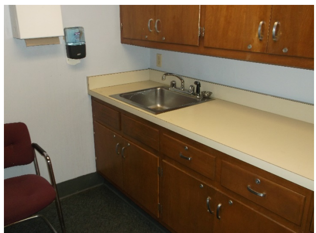
Break room counter/sink at 36"
