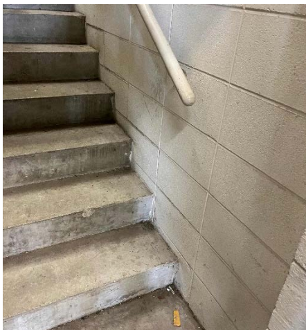
Lack of handrail extension
