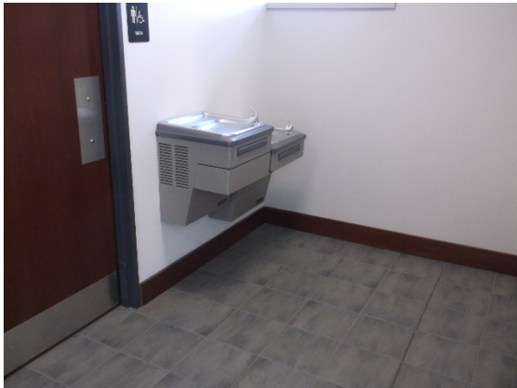
Electric water coolers – lobby
