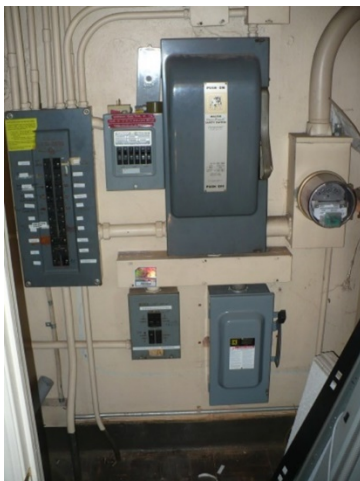
200A service meter and disconnect
