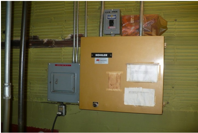
50A transfer switch
