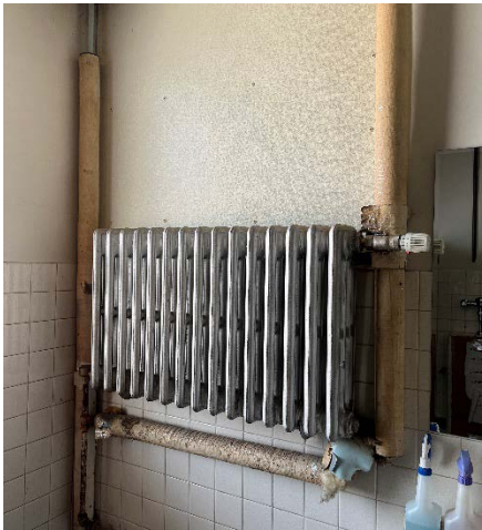
Friable insulation on piping
