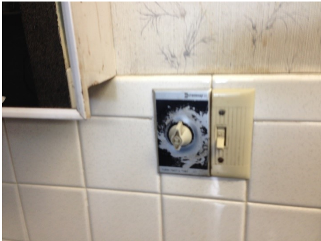
Exhaust fan manual switch (typical)
