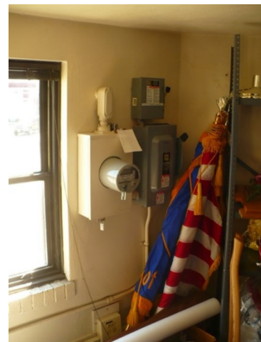
100A service meter and disconnect
