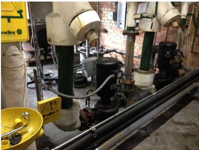
Induction unit water pumps
