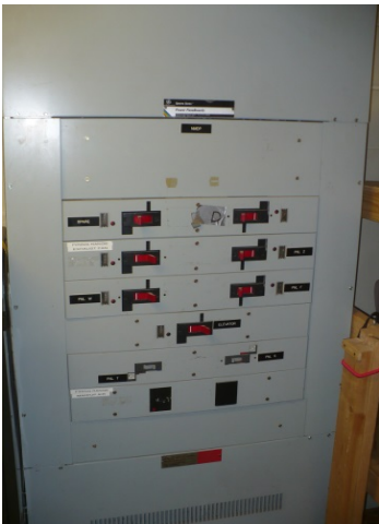
Normal main distribution panel
