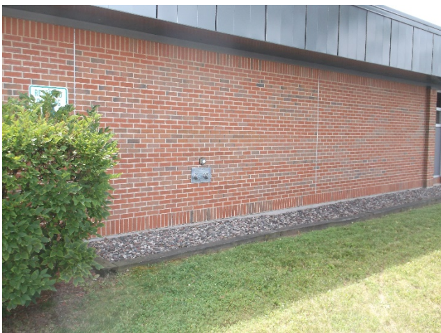
Fire department connection
