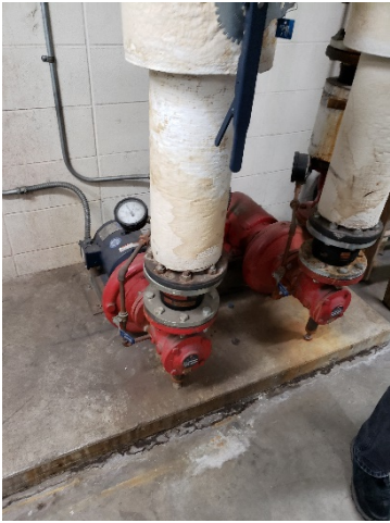
Hot water pumps
