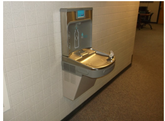
Electric water cooler
