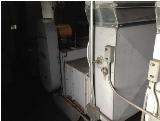
AHU-2 and AHU-3
