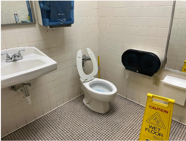
1 st Floor: not accessible toilet room
