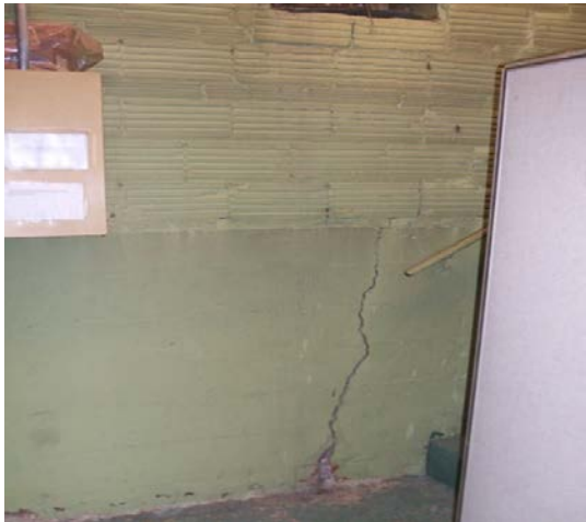
Cracked foundation wall in generator room (Note S1)
