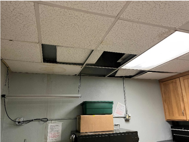
Missing and misplaced ceiling tiles
