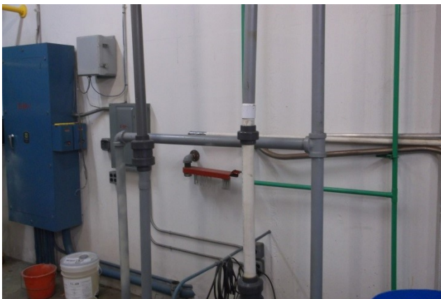
Pump discharge piping
