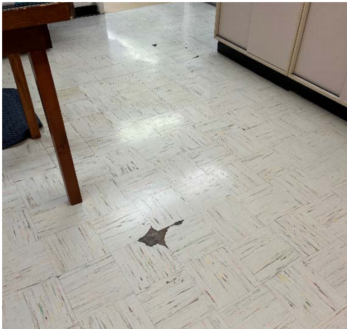
Chipped floor tile
