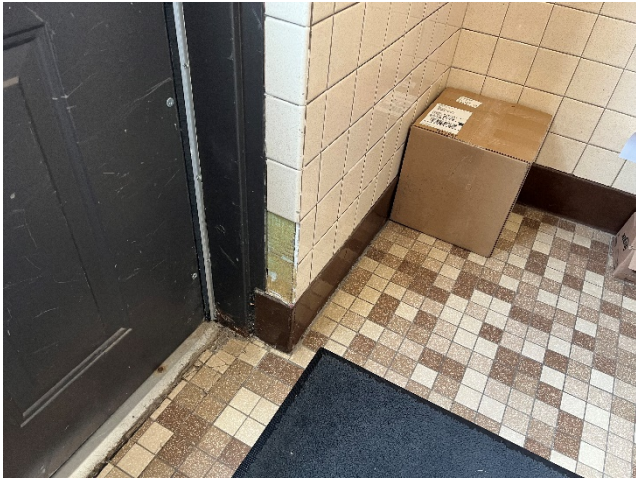
Missing wall tile
