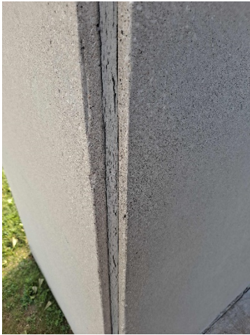
Caulking dried and brittle
