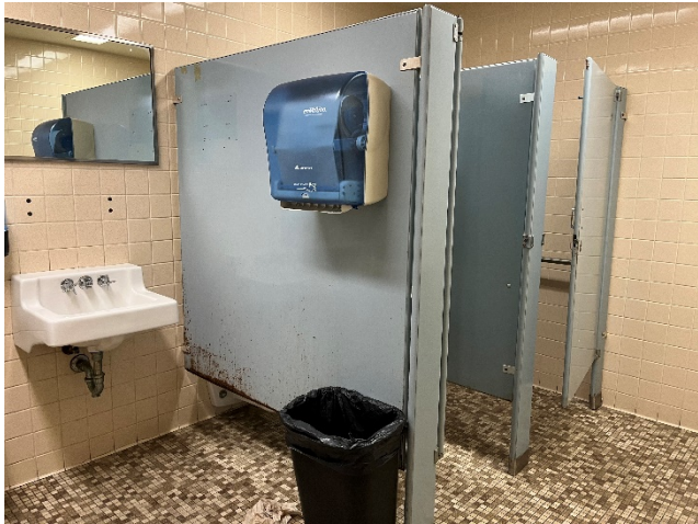
Rusted bottom of men's toilet partitions
