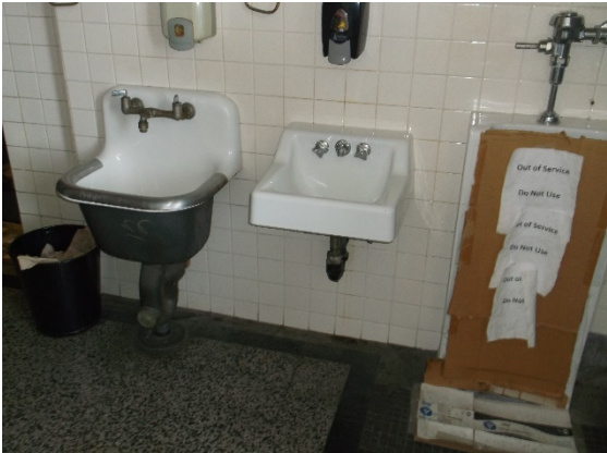
Sink, lavatory, urinal – women's
