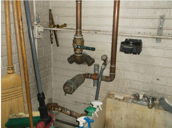
Fill connection(s) in garage
