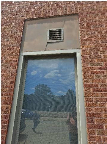
Transom faded and broken
