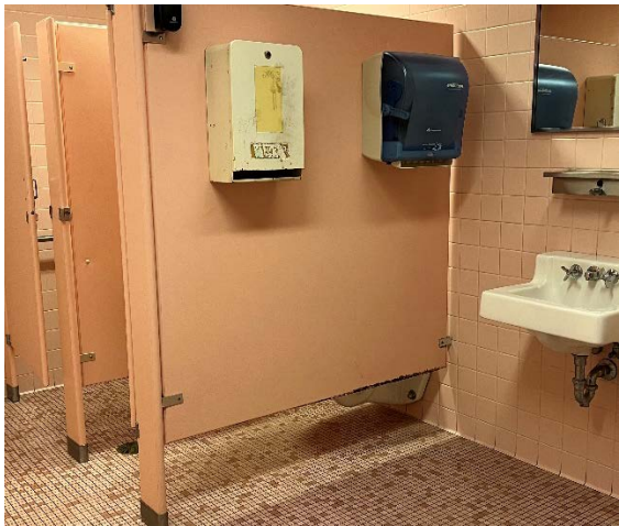
Rusted bottom of women's toilet partitions
