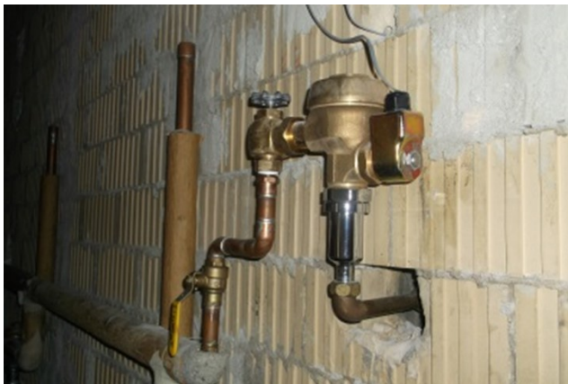
Flush valve in toilet chase
