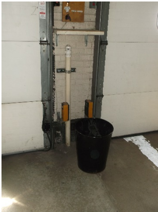
Studor vent - garage
