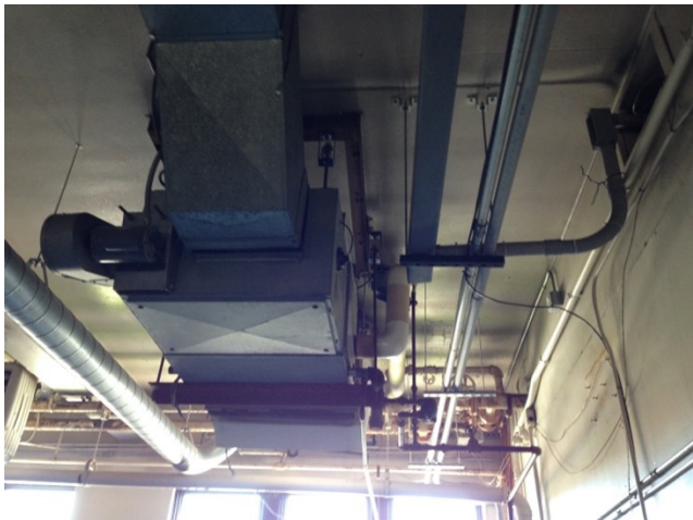
Make-up air unit
