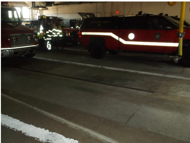
Garage trench drain
