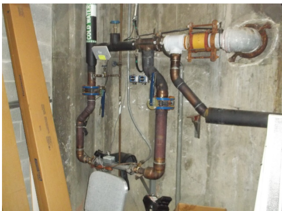
2" water meter, 4" water main
