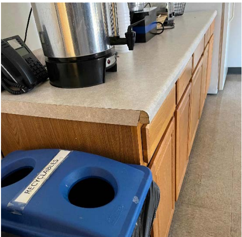
Chipped plastic laminate
