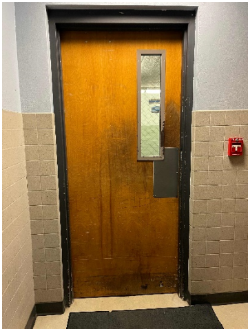
Chipped paint at lite and damaged wood finish Missing kick plate
