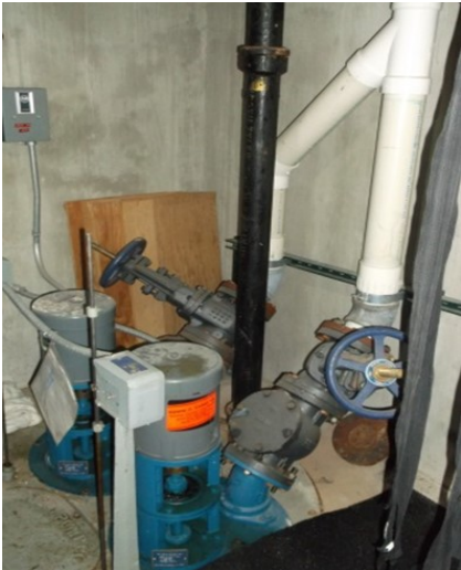
Sanitary ejector – duplex pumps
