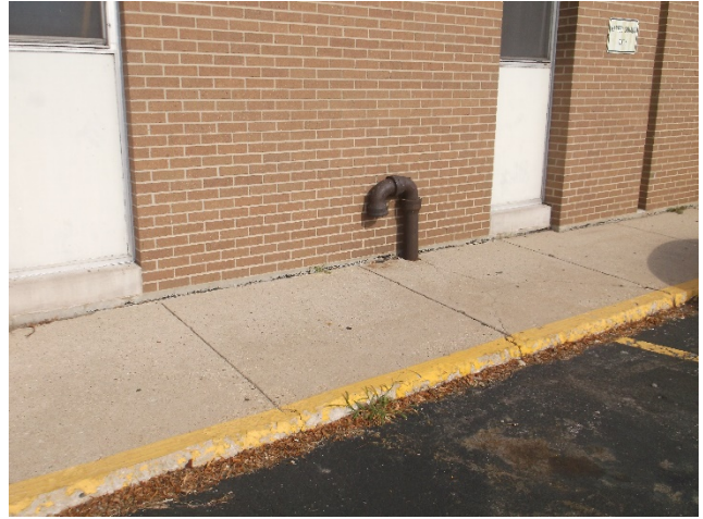
Garage catch basin vent
