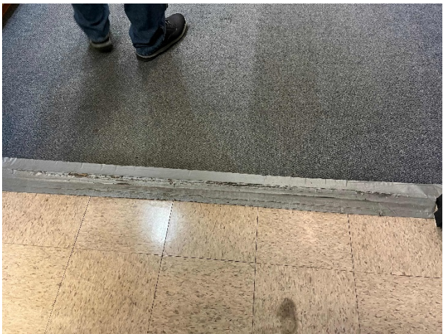
Duct tape at transition from carpet to VCT
