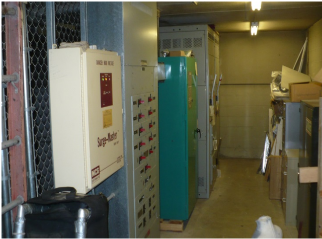
Main electrical equipment
