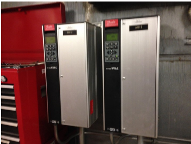
Air unit VFD's (boiler units similar)
