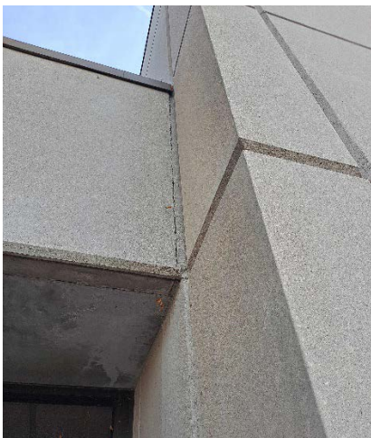
Caulking dried and brittle
