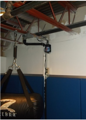
Drain tile sump/pump, alarm
