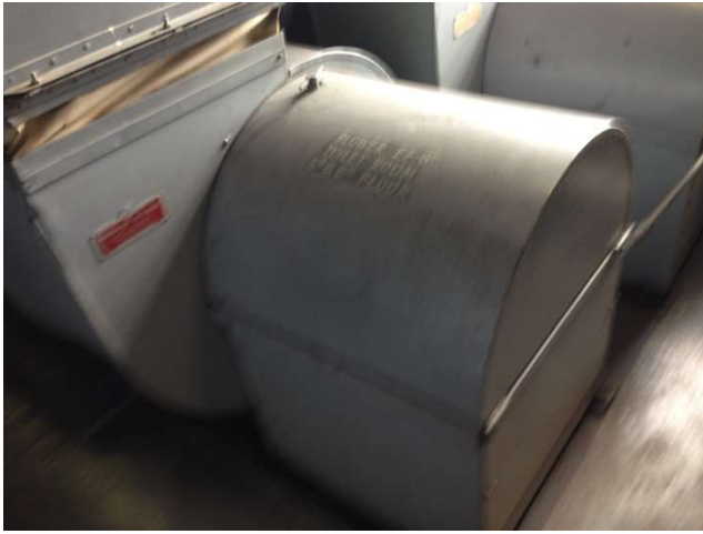
Typical exhaust fan
