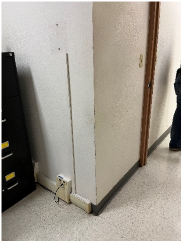
2 nd & 3 rd floors: typical chipped paint at exterior corner
