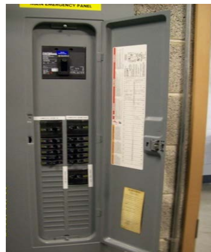
Main emergency panel
