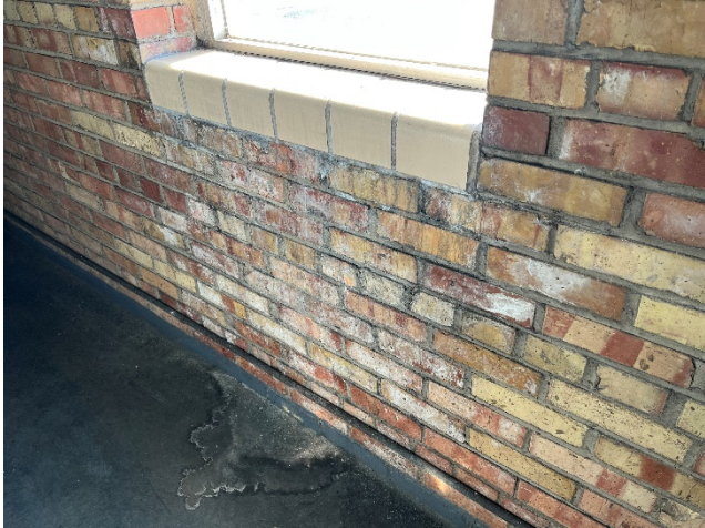
Effervescence on east wall
