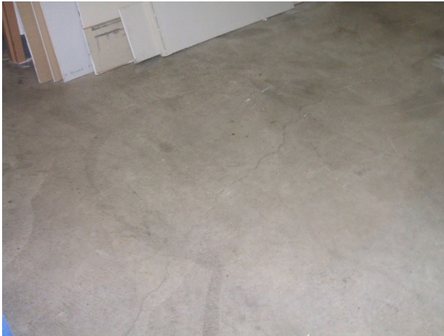
Shrinkage cracks in basement slab (Note S1)
