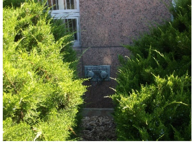
Fire dept. connection
