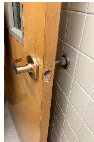
Missing latch at north stair door
