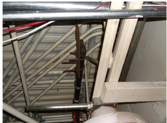
Sprinkler head with baffle in electrical room
