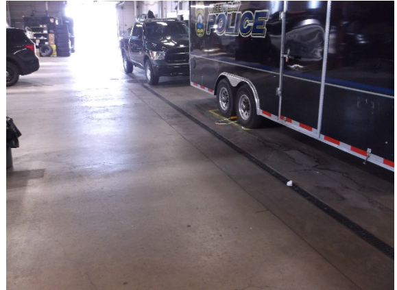
Garage trench drain
