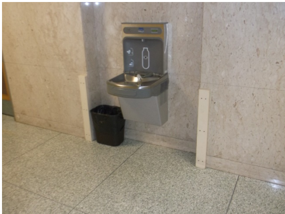
Electric water cooler – typical corridor
