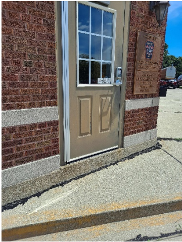
Door not egressing to grade
