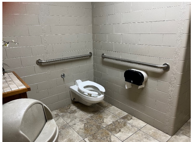
5 th floor: Typical missing vertical grab bar
