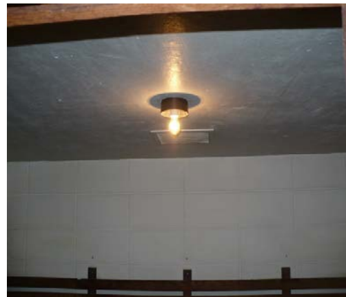
Sauna light missing lens
