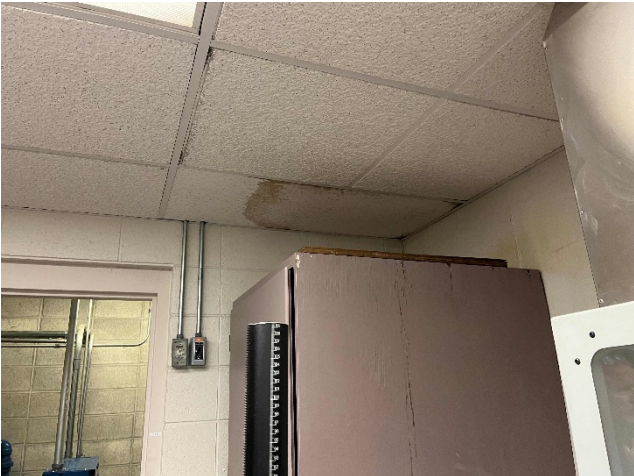
Typical stained ceiling tile
