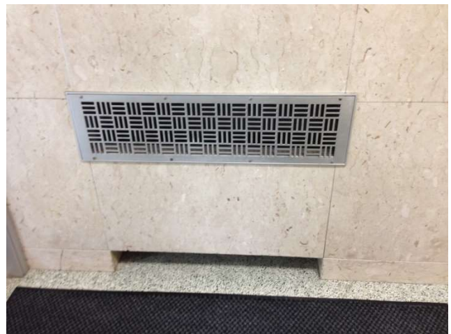
Vestibule heater (typical)
