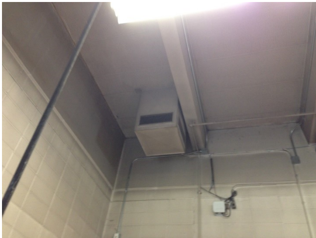
Garage exhaust (near ceiling)
