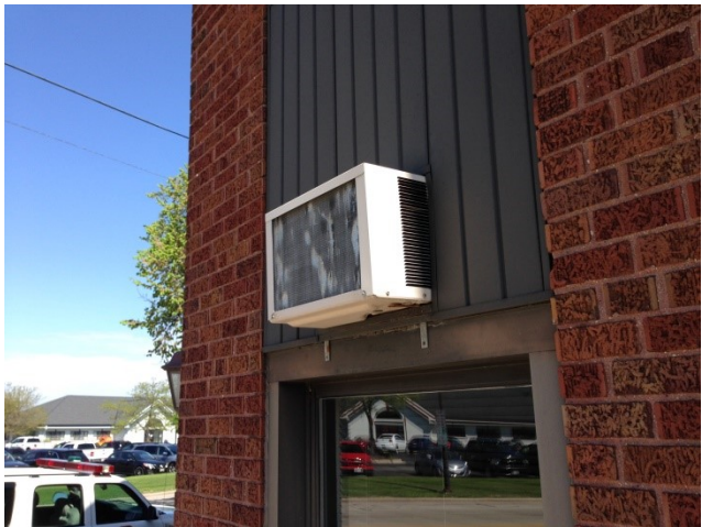
Through wall air conditioner
