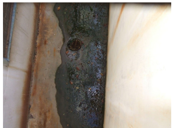
Area well drain
