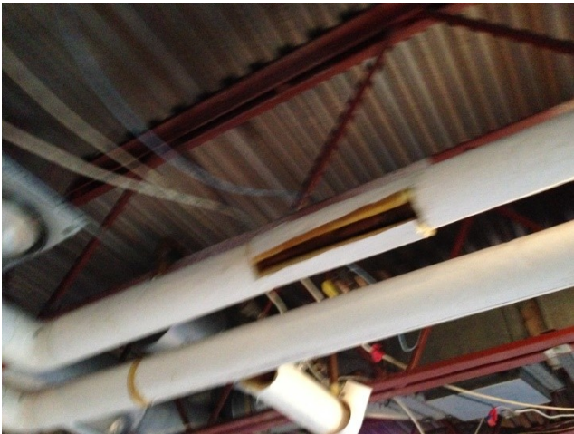
Poor insulation (typical)
