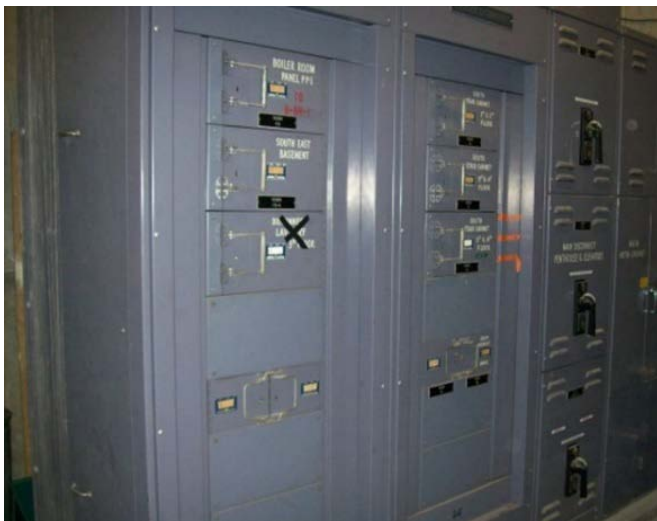
MSB main switchboard
