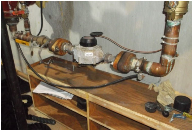
Water meter with by-pass
