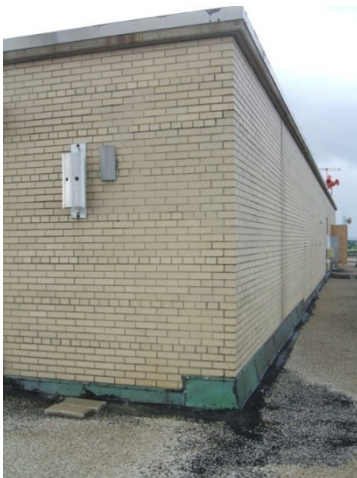
Expansion cracking of brick penthouse (Note S3)
