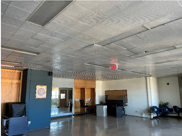
Typical spline ceiling issues
