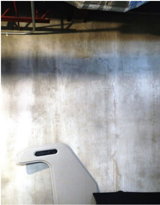
Concrete shrinkage crack in basement storage room (Note S1)
