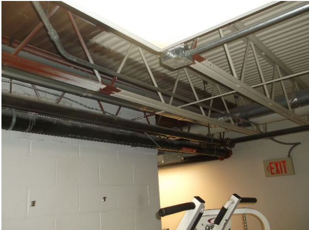
Fire protection main
