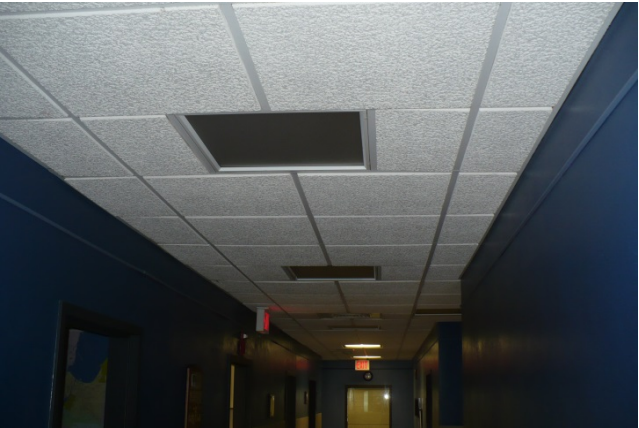
1 st floor corridor lighting
