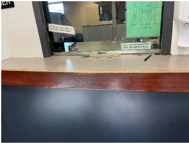
Worn finish at reception counter
