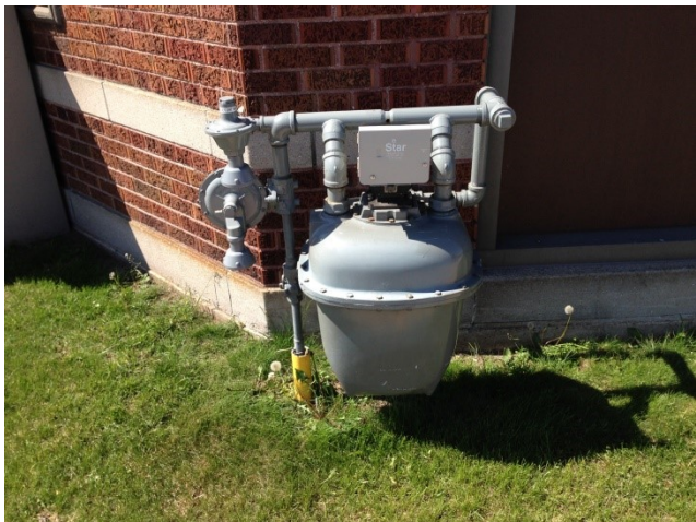
Gas meter (intake louver out of frame)
