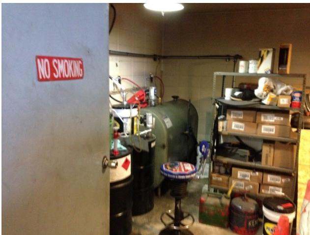
Hazardous storage room (vented tanks)
