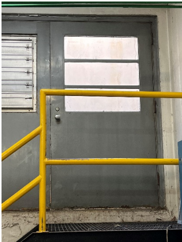
Missing weatherstripping at rusted door
