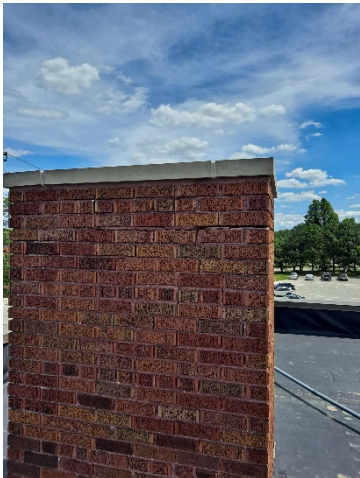
Tuck pointing needed at chimney
