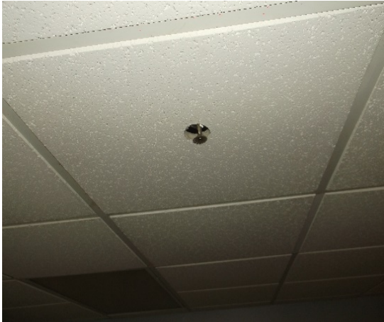
Sprinkler head – missing escutcheon
