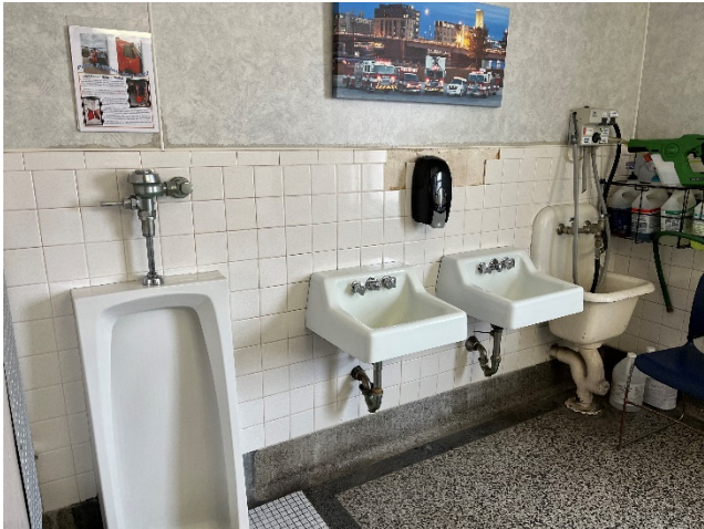
Missing wall tile at plumbing wall
