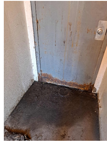
Rusted door to window well
