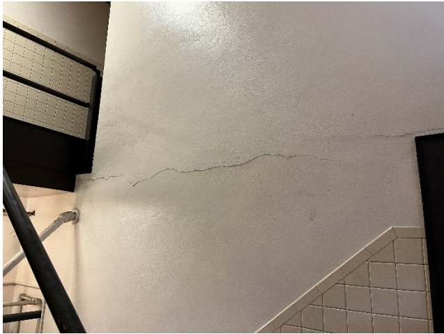
Cracked plaster at stair
