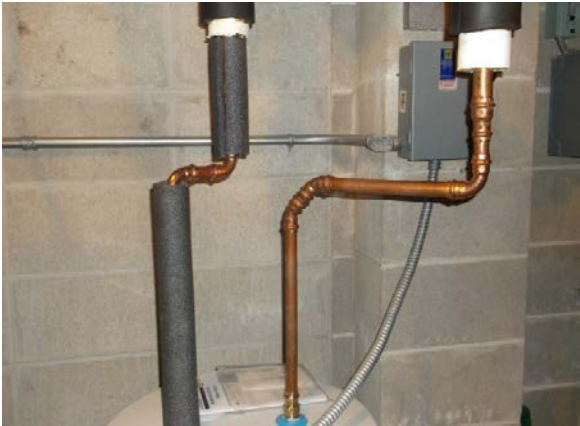
Water piping at water heater, pro-press piping
