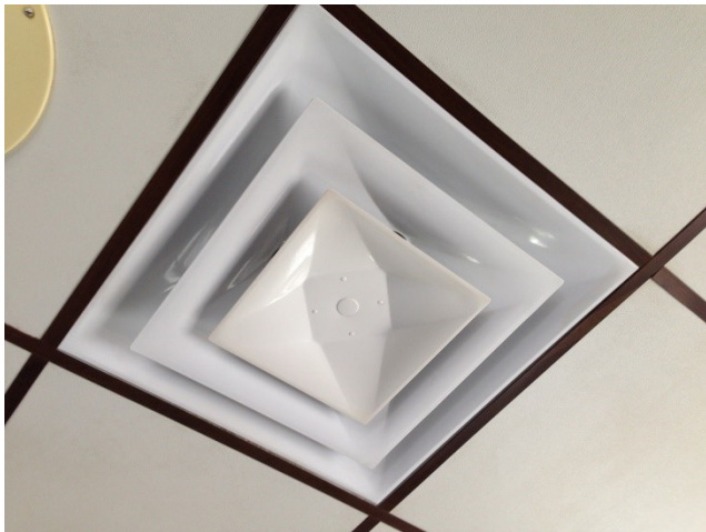
Supply grille (typical)
