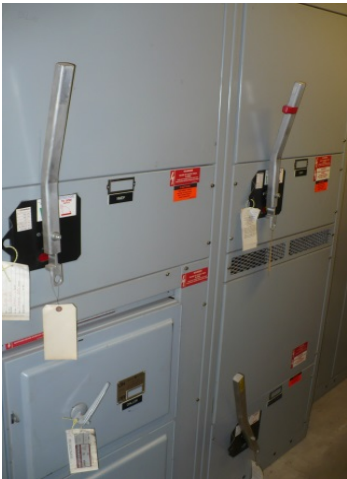
Main fused switchboard
