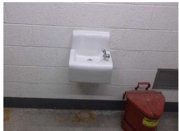
Drinking fountain - basement
