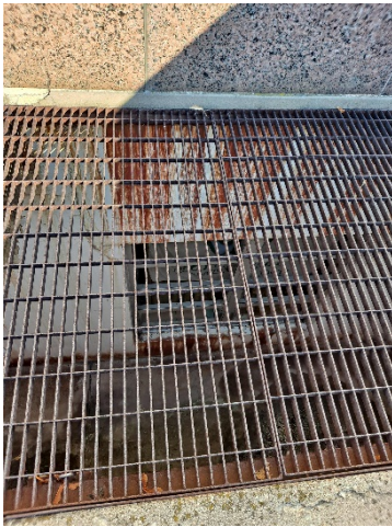
Rust on window well walls
