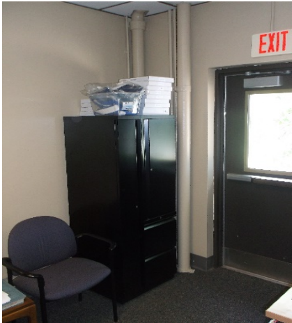
Storm piping, sanitary vent
