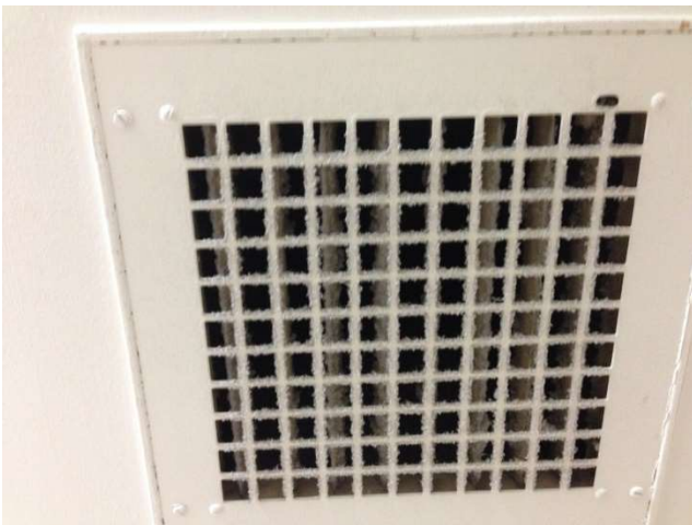
Exhaust grille (typical)
