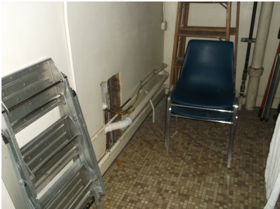
PEX piping to kitchen sink
