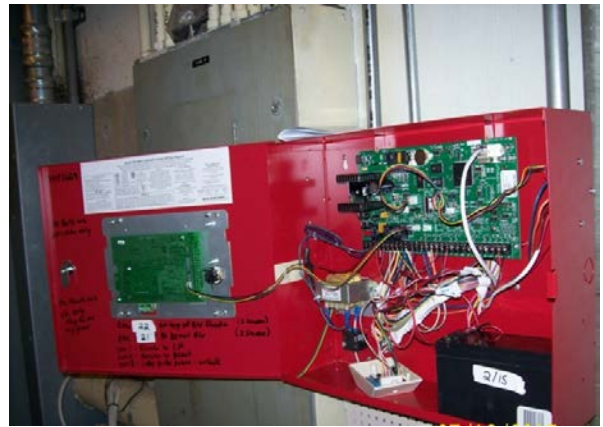
Fire alarm panel
