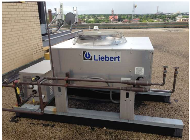
IT department condenser
