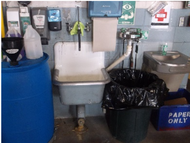
Sink, EWC & eyewash in garage
