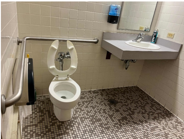
Toilet with grab bars, but lacking clear floor space
