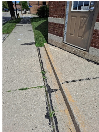
Egress door not at level of egress
