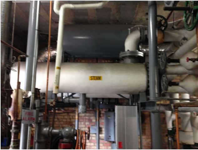
Building steam to water converters
