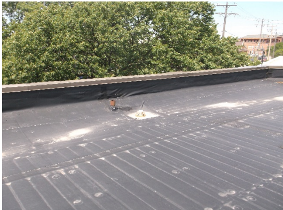
Sanitary vent & roof drain
