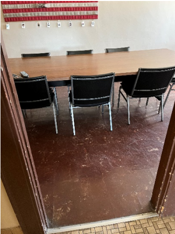
Chipped paint at wood door frame
