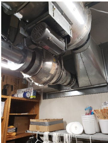
Interior exhaust fans (noisy)
