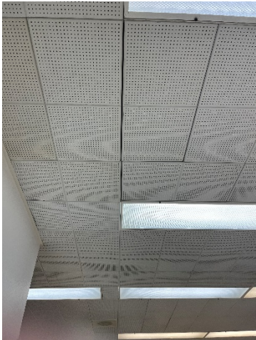
Typical spline ceiling issues
