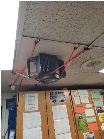
Makeshift room ventilation unit
