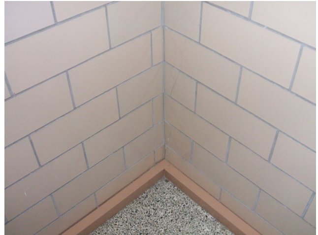
Settlement cracks in glazed tile walls of stairs (Note S2)
