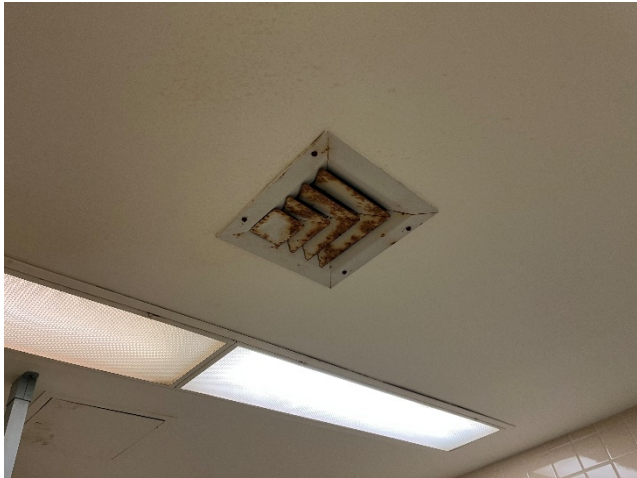
Rusted ceiling diffuser at basement toilet room
