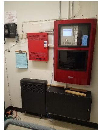
Fire alarm panel
