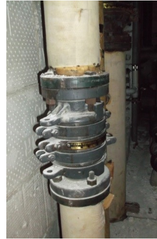
Expansion joint (4th floor) toilet chase
