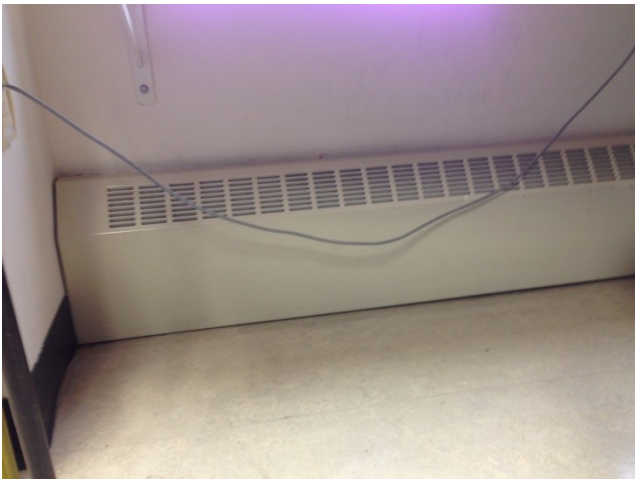
Fin tube (installed at floor)
