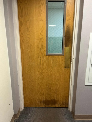
Damaged wood veneer & missing kick plate
