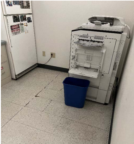
Chipped floor tiles
