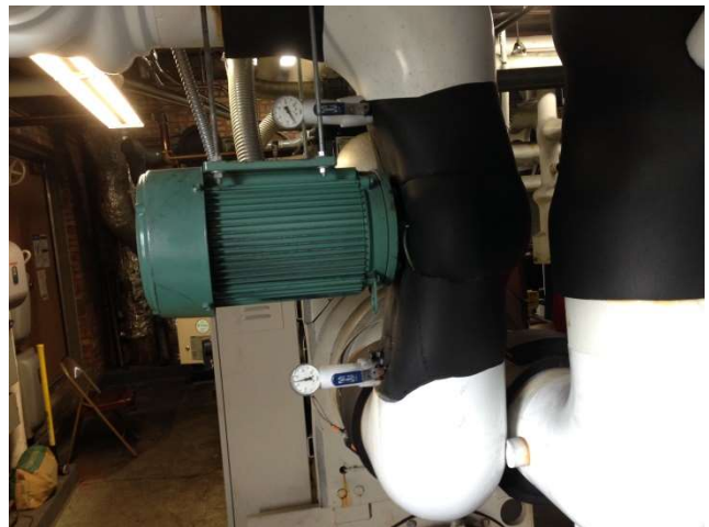
Chilled water pump
