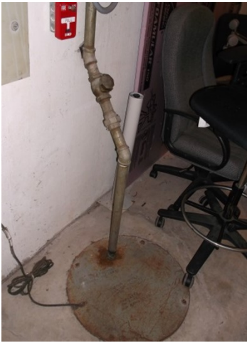
Drain tile sump/pump
