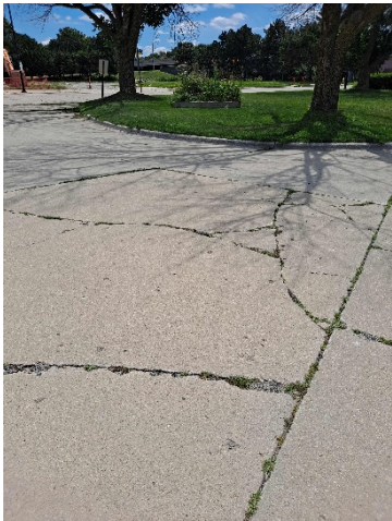
Cracked driveway apron
