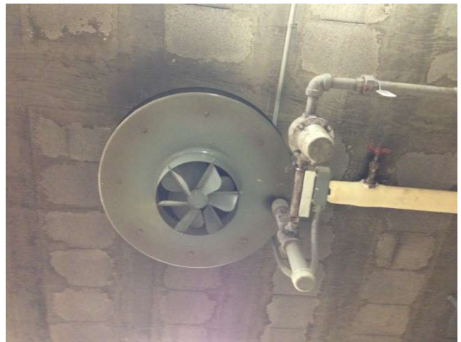
Typical unit heater
