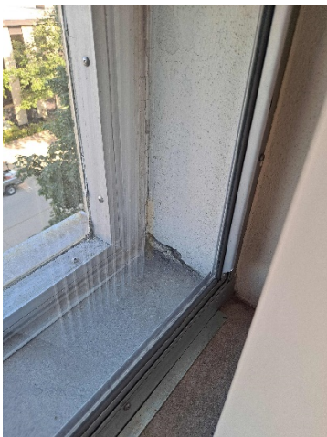
Rust on window well walls
