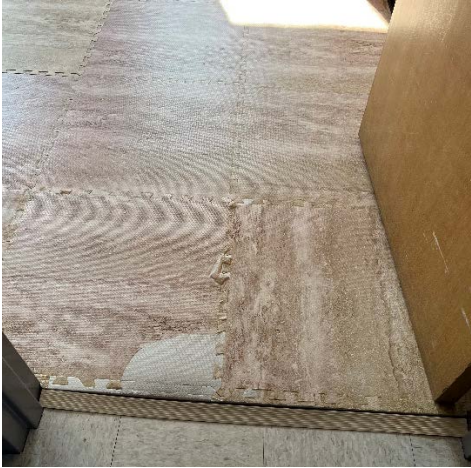
De-laminated interlocking floor tiles
