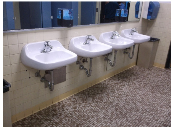
Men's toilet room lavatories
