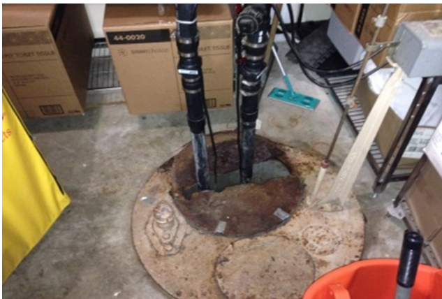
Sump, duplex pumps
