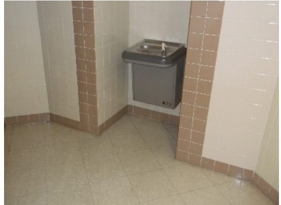
Electric water cooler
