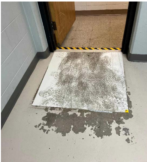
Chipped paint at shooting gallery entry
