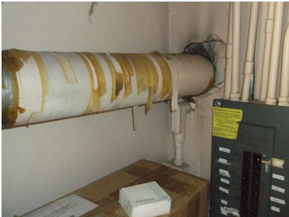
Water piping thru electrical closet
