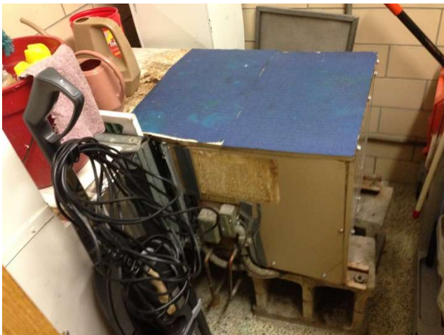
Water cooled blower coil (AHU-5)
