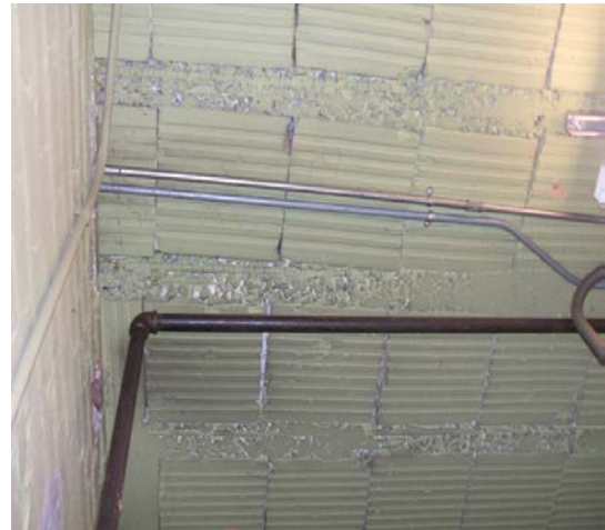
Exposed reinforcing in joists above generator (Note S2)
