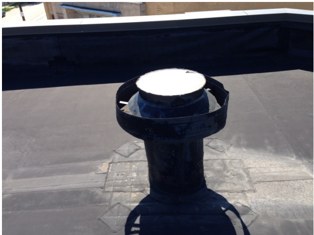
Roof exhaust hood
