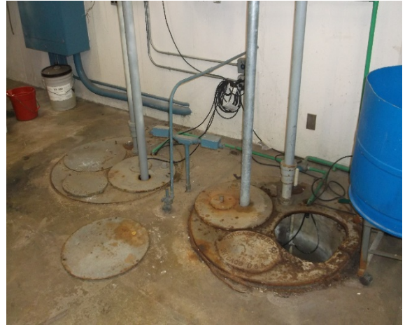
Drain tile, sanitary sump/pump
