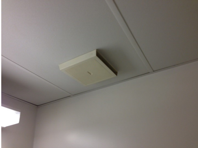
Typical ceiling exhaust fan
