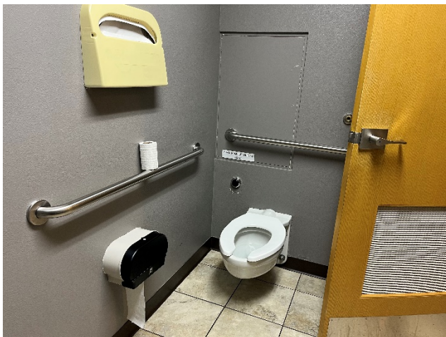
3 rd floor: grab bar mounted on panel
