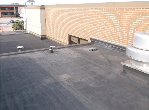
Roof Drain, Sanitary Vent
