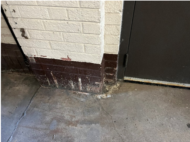
Spalling brick due to moisture exposure
