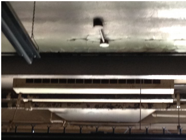
Unit ventilator (steam)
