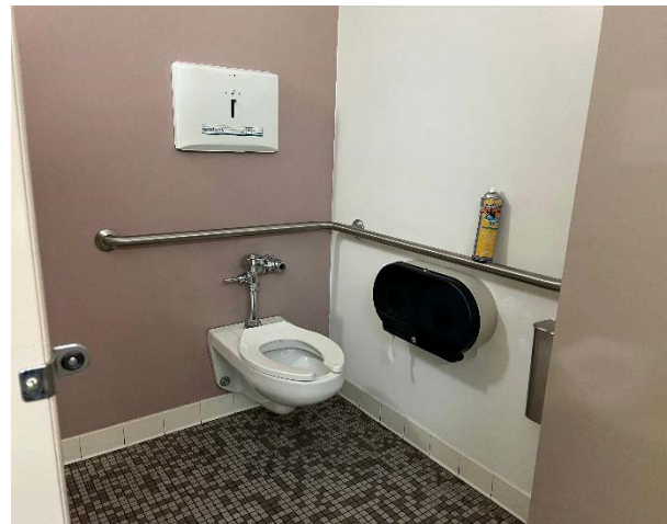
Toilet stall accessible, but room is not (See photo above)
