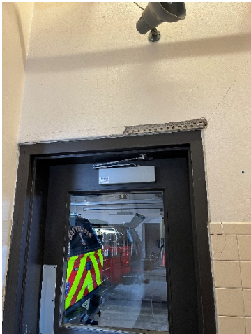
Cracked/missing plaster over door
