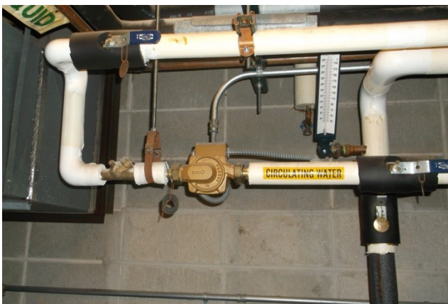
Hot water recirculating pump
