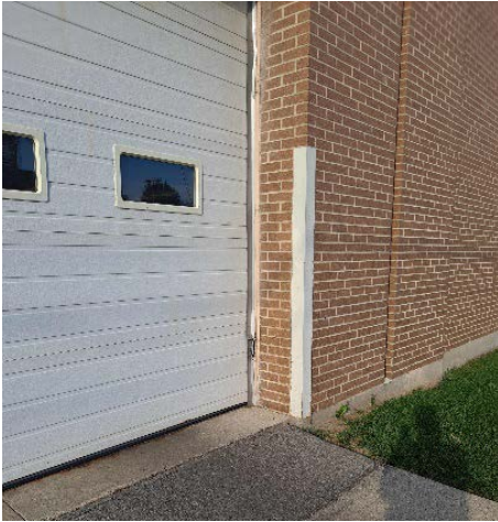
Damaged door jamb and door track
