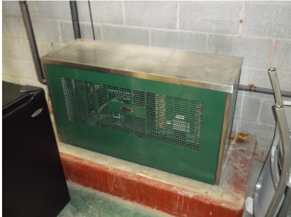
Chiller for drinking fountain(s)
