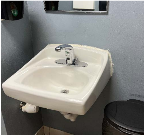
Excessive sealant at lavatory
