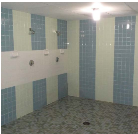
No accessible shower – men's
