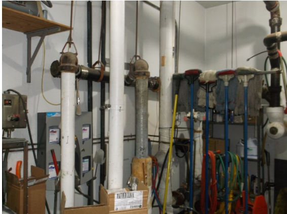
Pump discharge – sanitary piping
