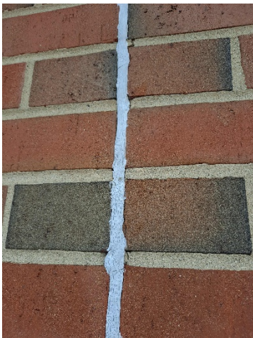
Dried and cracking expansion joint material
