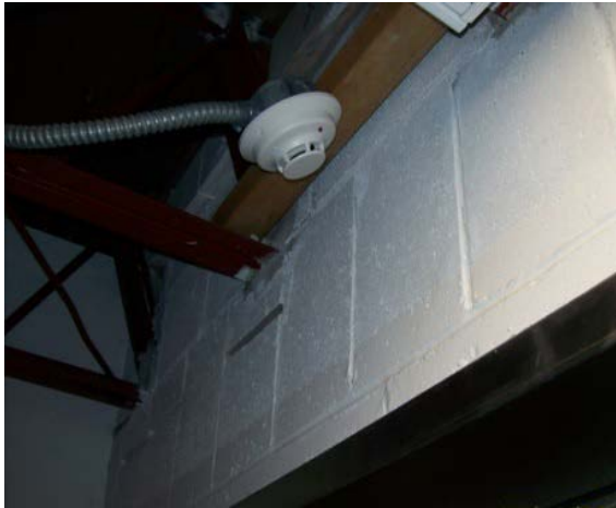
Detector not installed properly
