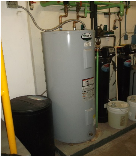
Electric water heater
