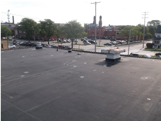
Roof drain(s), sanitary vent
