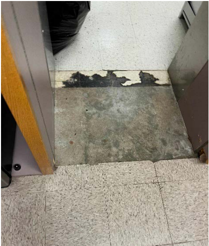
Missing VCT at basement
