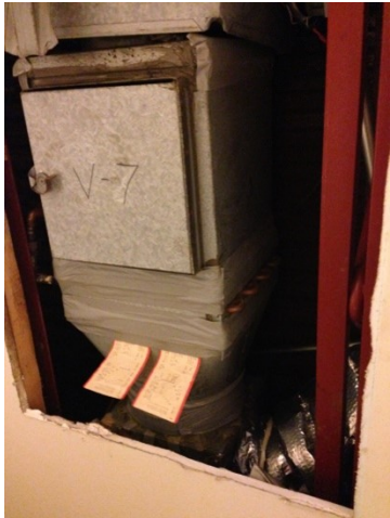
Older VAV terminal
