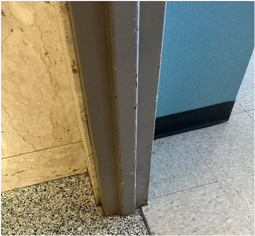
Chipped paint at HM frames
