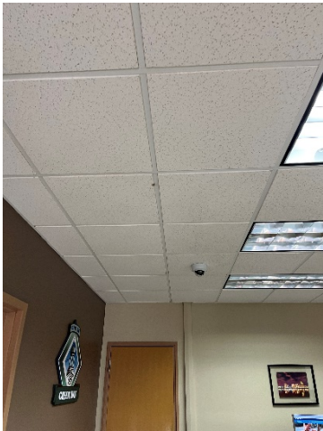
Small chip in ceiling panel
