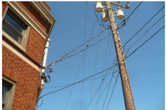
Electrical utility service entrance
