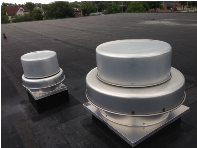
Power roof ventilators (typical)
