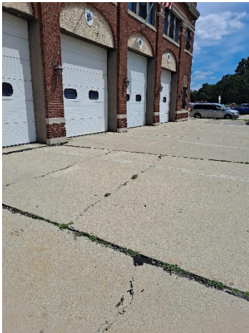
Cracked driveway apron
