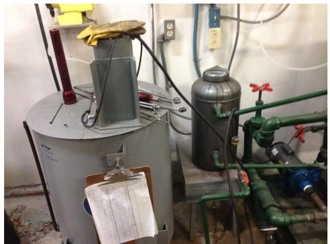
Boiler chemical feeder
