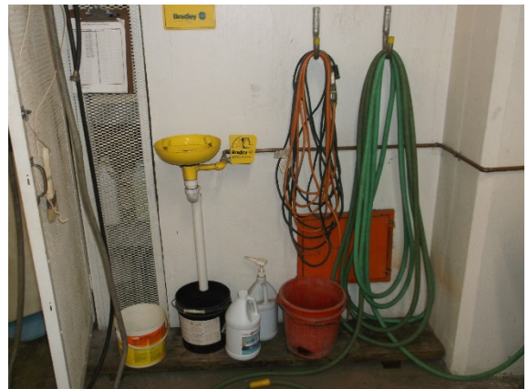
Eyewash – boiler room
