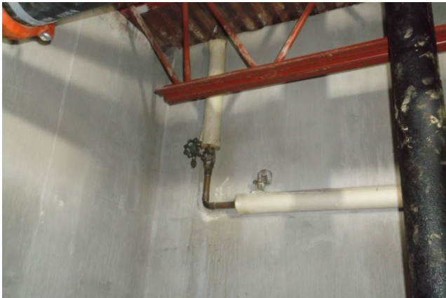
Water piping, Gate valve
