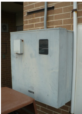
Main electrical service meter
