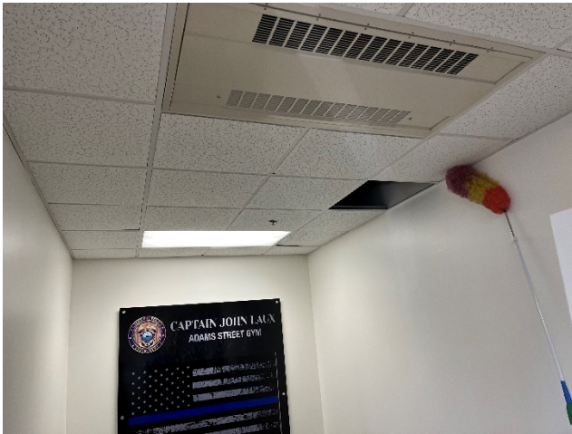
Missing ceiling tile at back stair shaft
