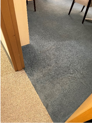
Ripped carpet seam
