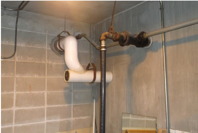
Storm piping, drain tile pump discharge
