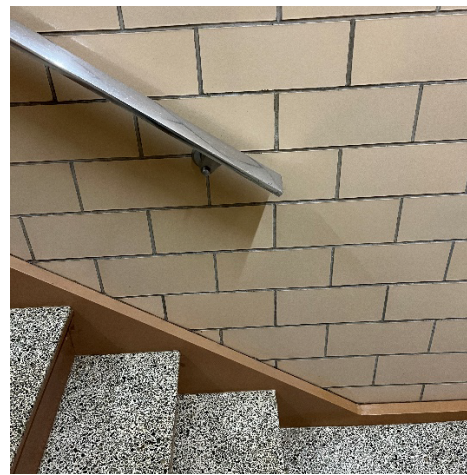
Lack of handrail extension past lowest tread
