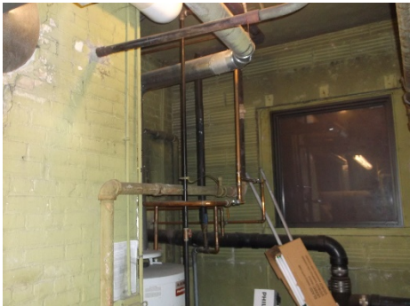
Sanitary/water piping – boiler room
