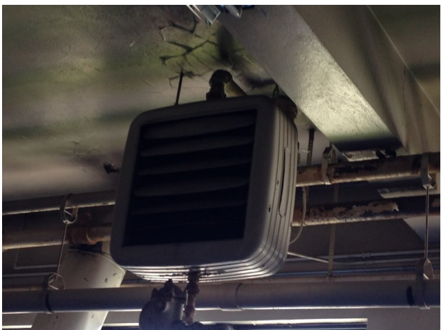
Steam unit heater (bare piping)
