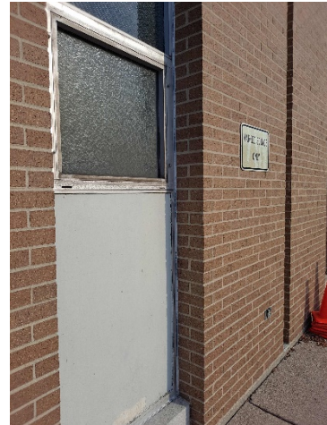
Faded window infill panels
