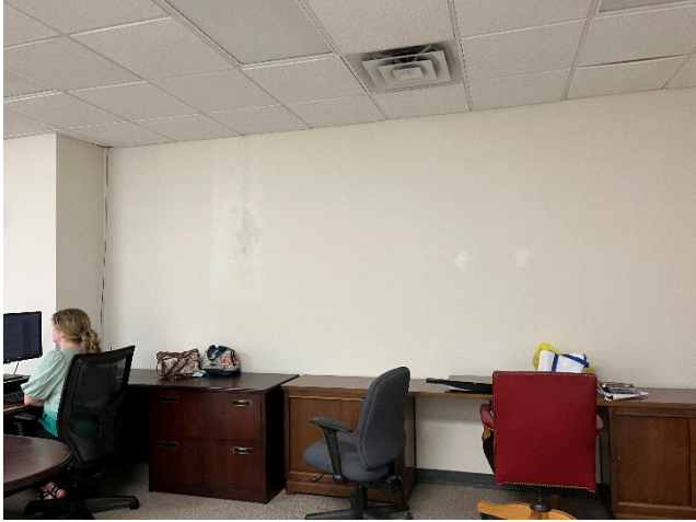
Visible wall patches
