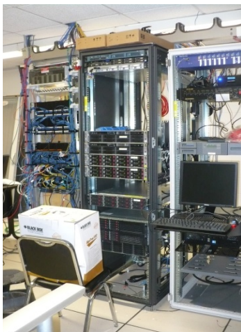
Basement data rack
