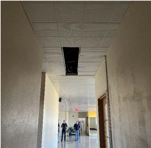
Missing light fixture
