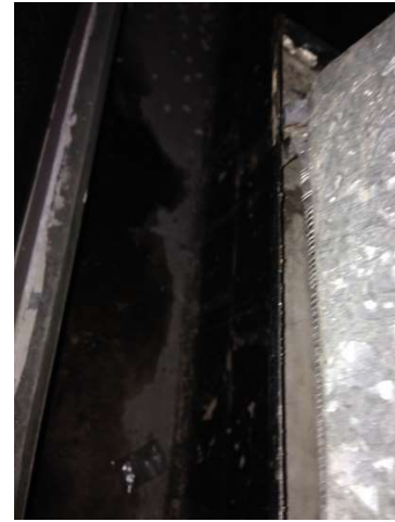
Condensation below induction unit (in wall)
