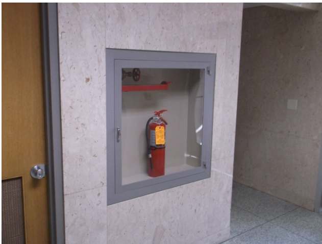
Hose valve cabinet
