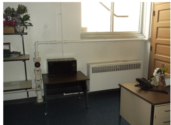
Sanitary vent piping
