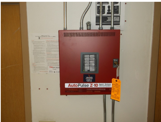
Halon control panel – IT room
