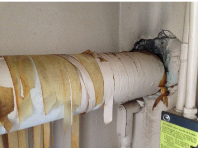
Poor insulation condition
