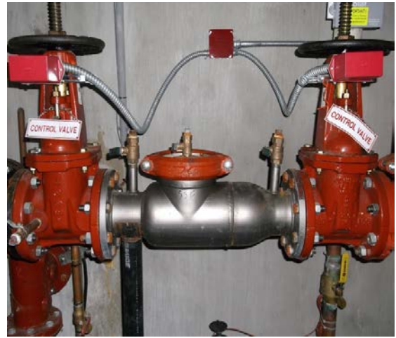
4" double check backflow preventer
