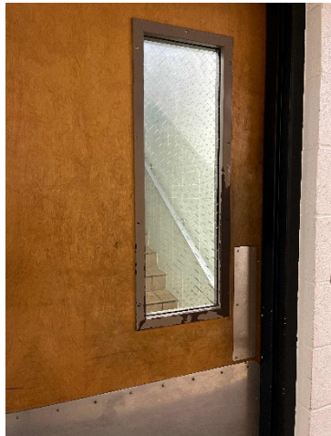
Chipped paint at lite and damaged wood finish
