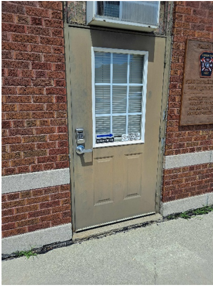
Recommend threshold at entry
