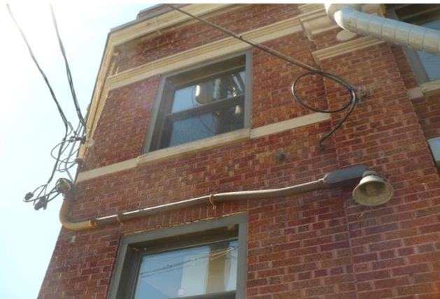
Electrical utility service entrance
