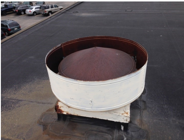
Garage exhaust vent (typical)
