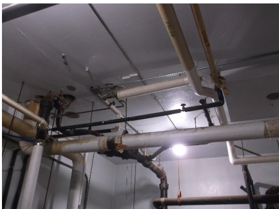
Water & sanitary piping
