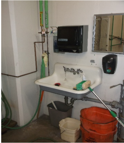
Janitors' sink – boiler room
