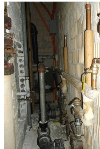
Piping in toilet chase – typical
