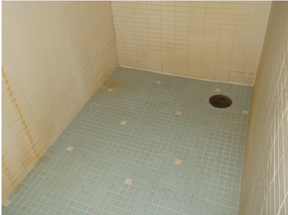
Men's shower room floor drain
