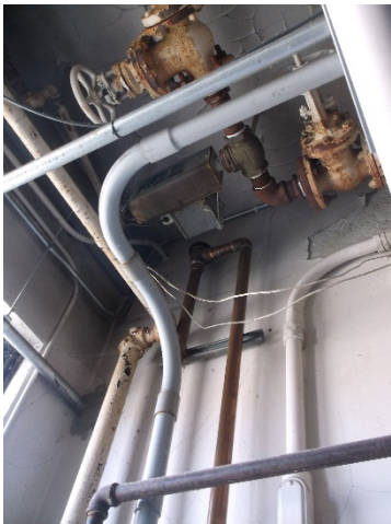
Fill lines backflow preventer
