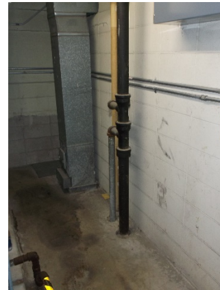
Sanitary vent piping
