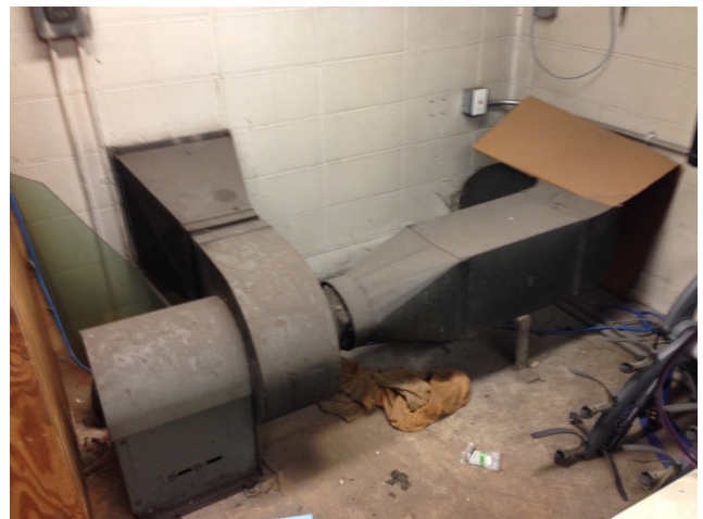
Garage storage exhaust fan (old)
