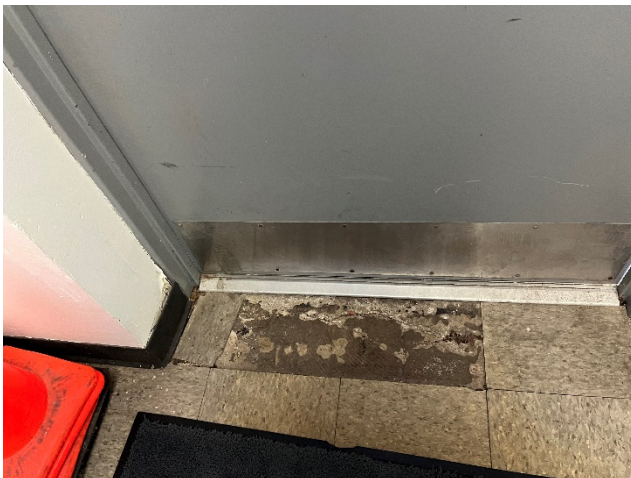
Missing vinyl tile at back door
