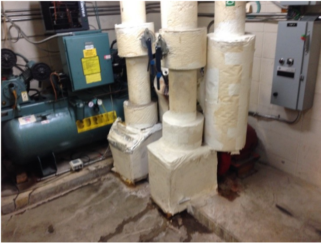
Chilled water pumps
