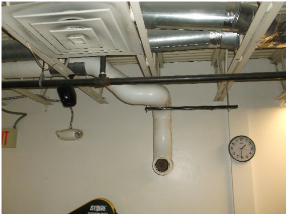
Storm piping - insulated
