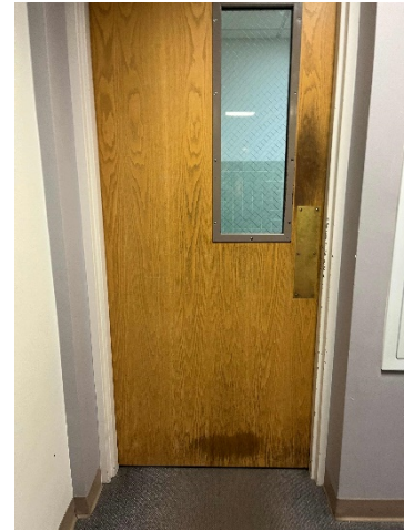
Route into 2 nd floor toilets lacks clear floor space
