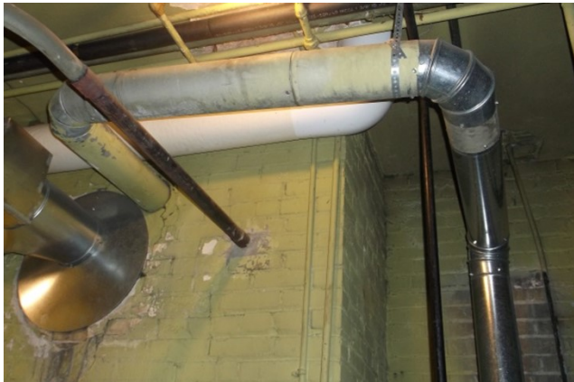
Water heater vent piping
