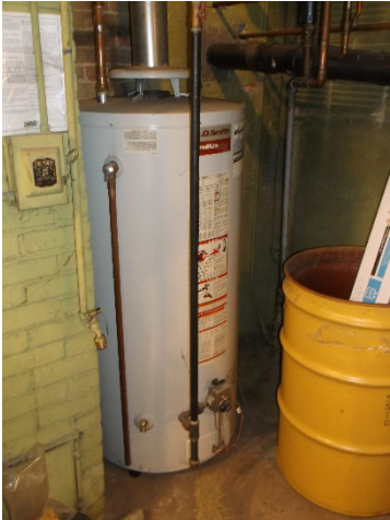
Water heater – gas fired
