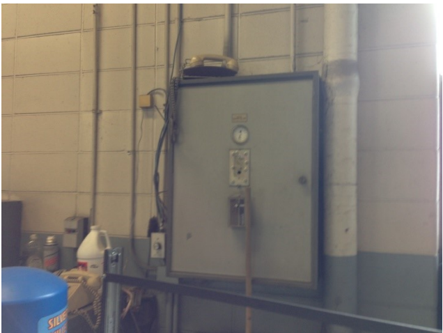
Garage control panel
