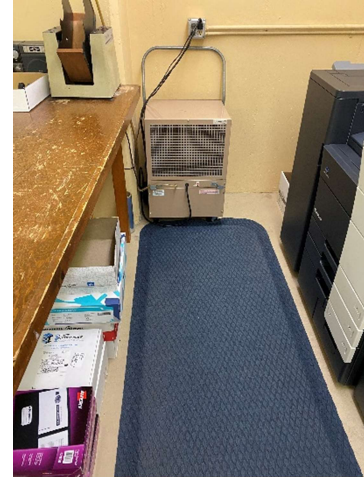
Print room dehumidification (humidity issues)
