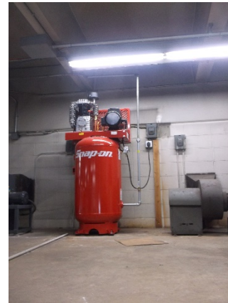
Shop air compressor
