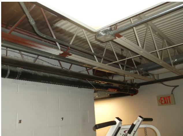
Fire protection main
