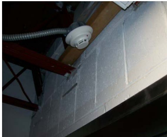
Detector not installed properly
