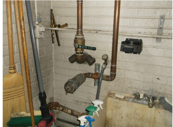
Fill connection(s) in garage
