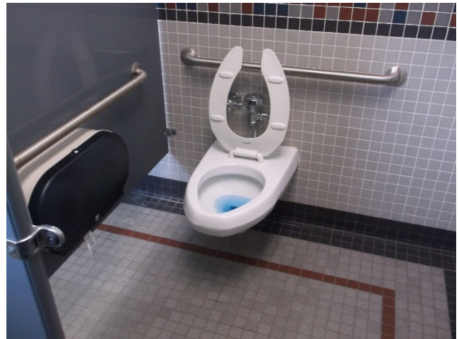
1 st floor Men's – missing vertical grab bar
