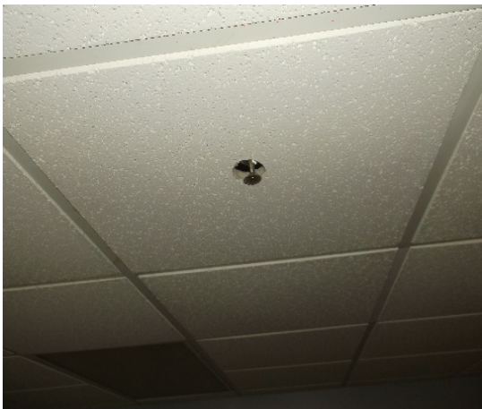
Sprinkler head – missing escutcheon
