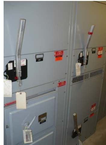
Main fused switchboard
