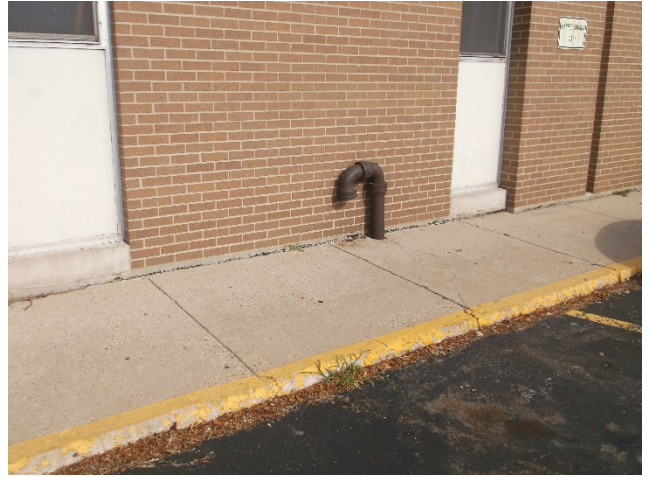
Garage catch basin vent
