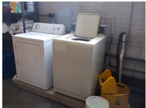
Washer/dryer in garage bay
