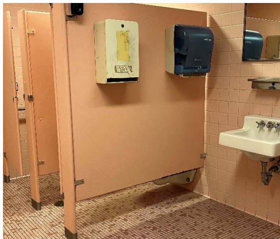
Rusted bottom of women's toilet partitions
