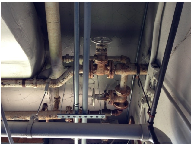
Uninsulated pipe (typical)
