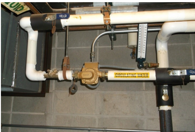
Hot water recirculating pump
