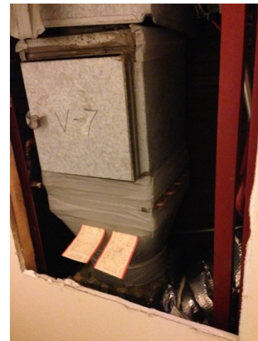
Older VAV terminal
