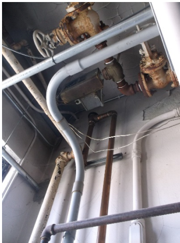
Fill lines backflow preventer
