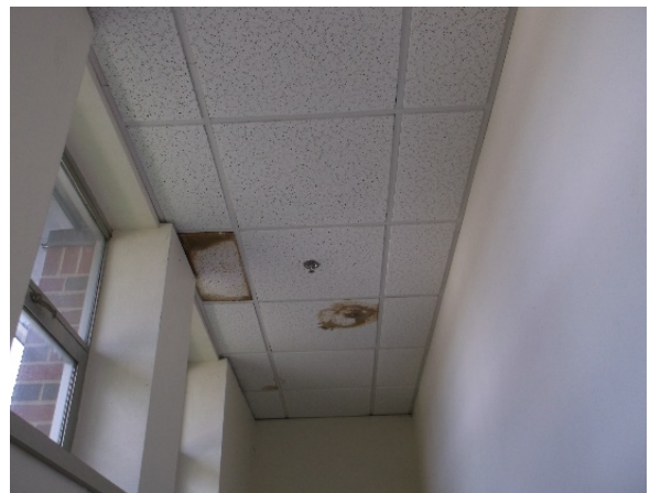
Sprinkler head in stairwell
