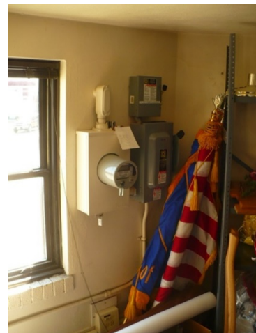
100A service meter and disconnect
