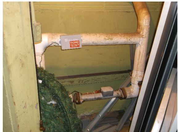
Water service, water meter with by-pass
