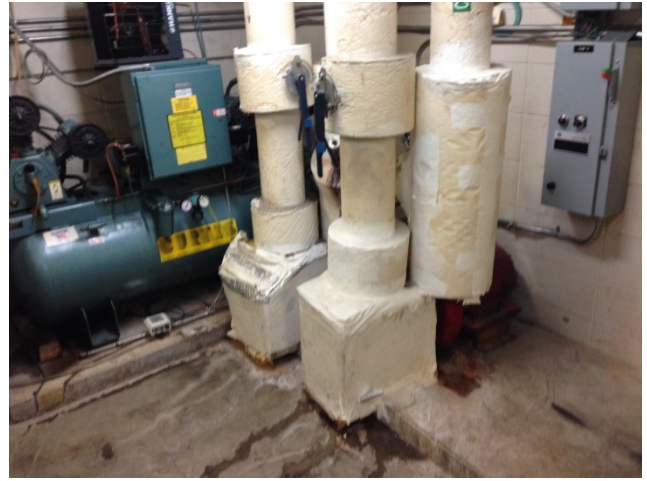
Chilled water pumps
