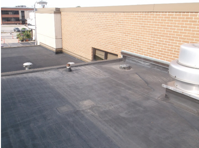
Roof Drain, Sanitary Vent
