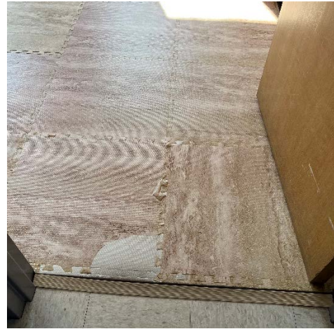
De-laminated interlocking floor tiles
