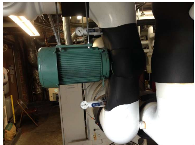
Chilled water pump
