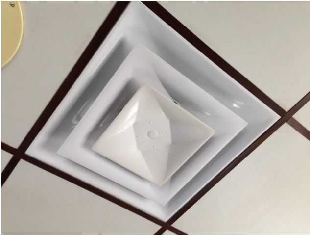
Supply grille (typical)
