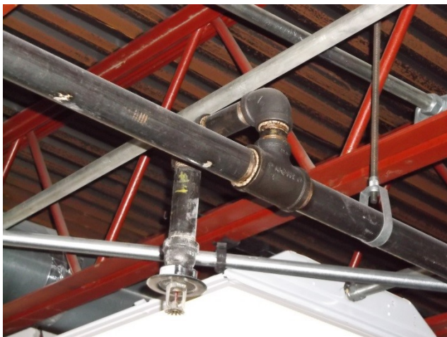
Pendent sprinkler head too far from ceiling
