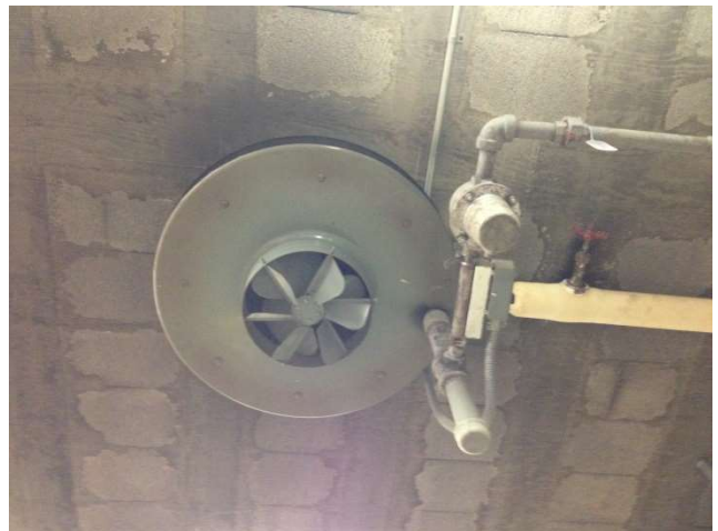
Typical unit heater
