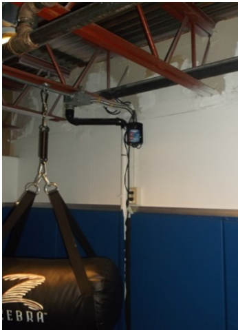
Drain tile sump/pump, alarm
