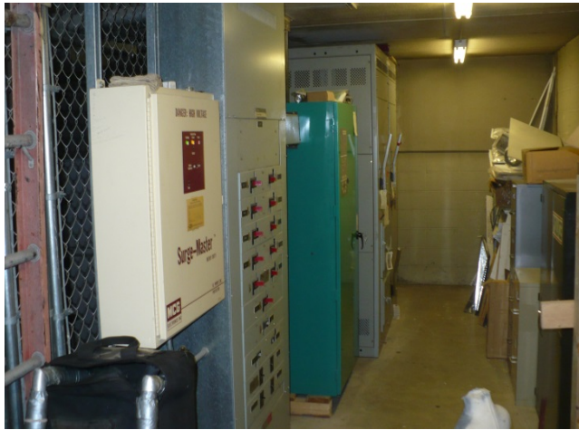
Main electrical equipment
