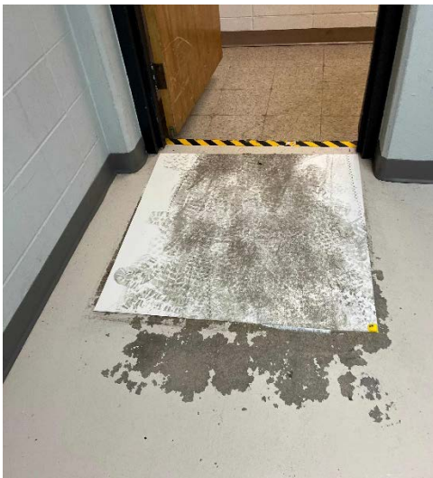
Chipped paint at shooting gallery entry
