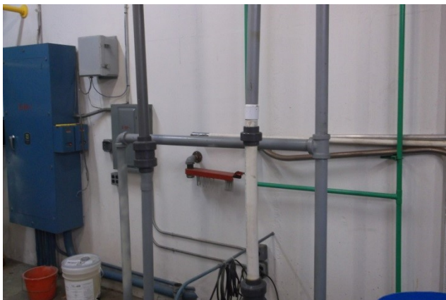
Pump discharge piping
