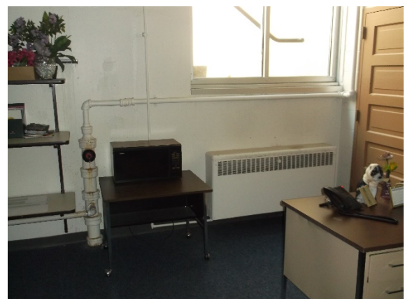
Sanitary vent piping
