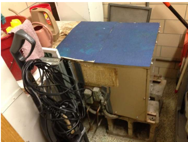
Water cooled blower coil (AHU-5)
