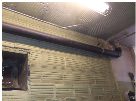
Sanitary piping – boiler room
