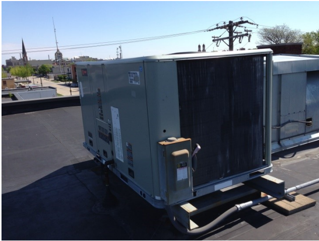
Roof top air unit
