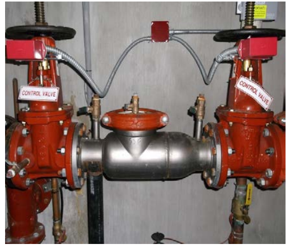
4" double check backflow preventer
