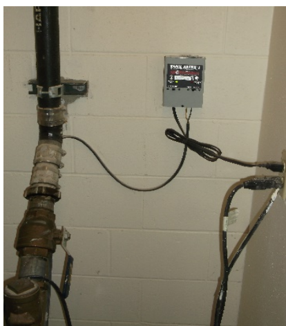
Elevator – high water alarm
