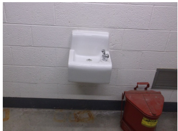
Drinking fountain - basement
