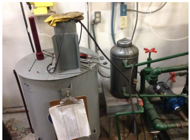
Boiler chemical feeder
