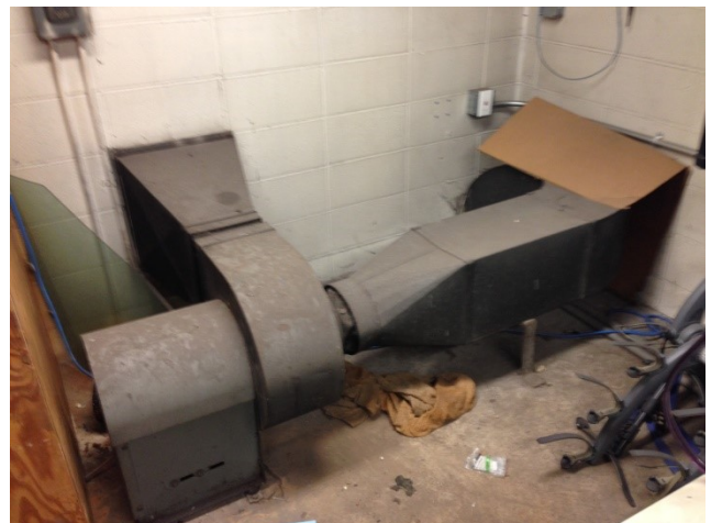
Garage storage exhaust fan (old)
