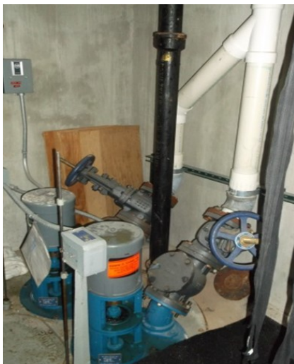
Sanitary ejector – duplex pumps
