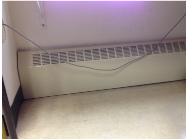
Fin tube (installed at floor)
