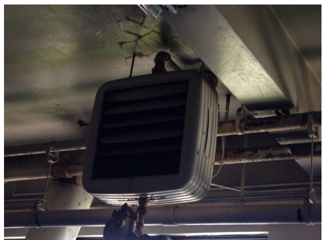
Steam unit heater (bare piping)
