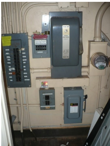
200A service meter and disconnect
