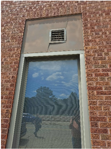
Transom faded and broken
