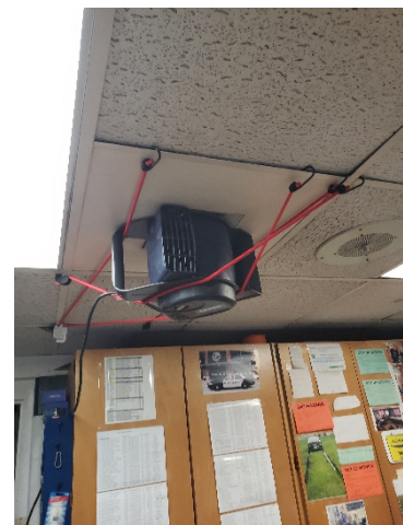
Makeshift room ventilation unit
