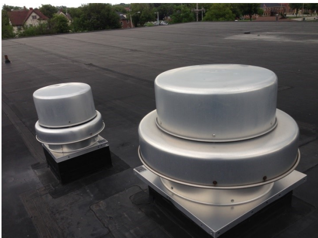
Power roof ventilators (typical)
