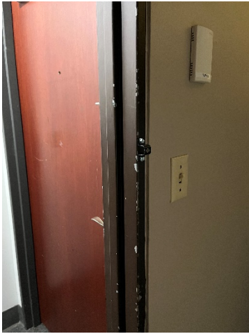
Chipped paint at basement door frames
