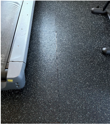
Gap in rubber floor tile
