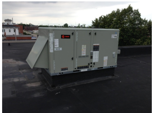
Training room air unit
