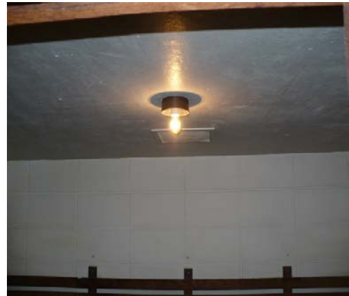
Sauna light missing lens
