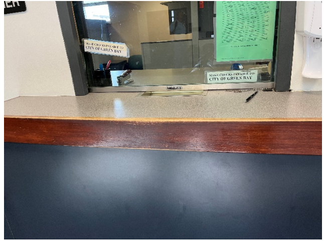
Worn finish at reception counter
