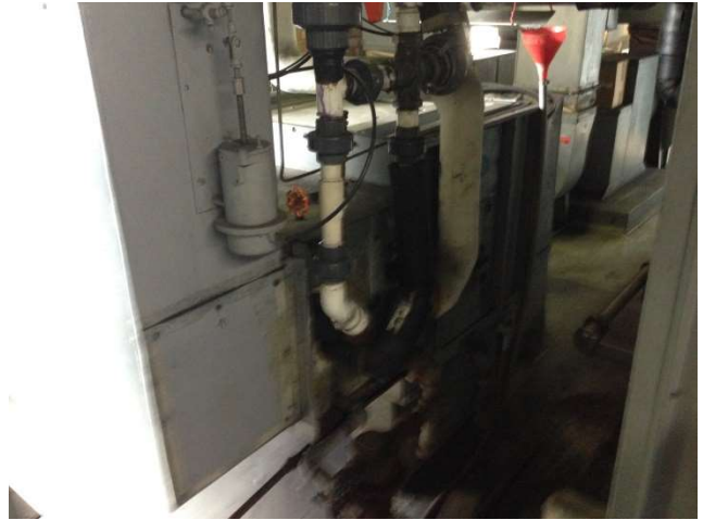
AHU-2 and 3 coils
