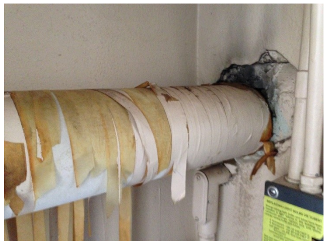
Poor insulation condition
