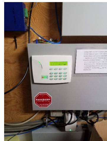
Card access system
