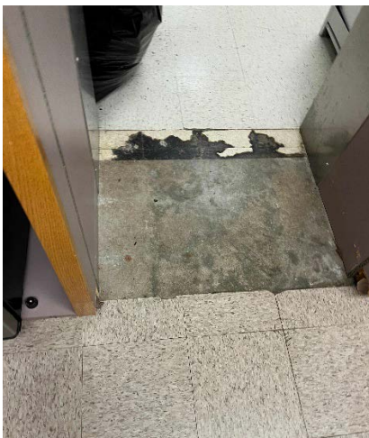
Missing VCT at basement
