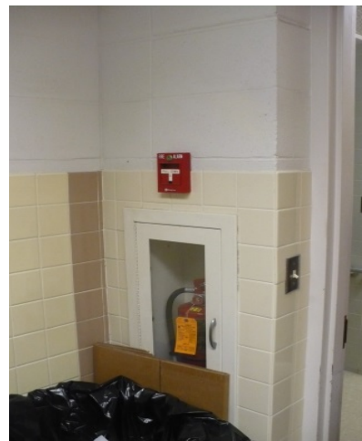
Non-ADA height of pull station
