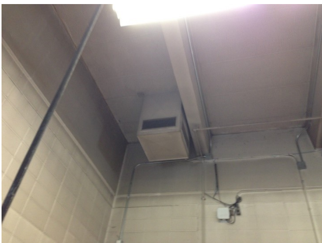
Garage exhaust (near ceiling)
