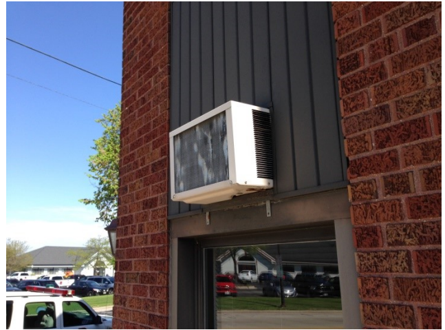
Through wall air conditioner
