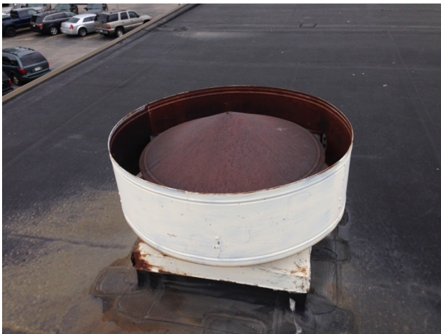
Garage exhaust vent (typical)
