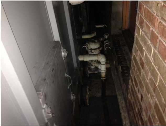
AHU-1 steam coil
