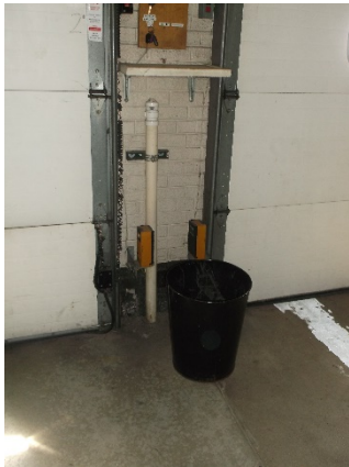
Studor vent - garage
