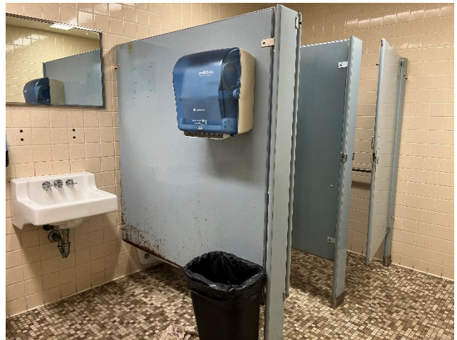
Rusted bottom of men's toilet partitions
