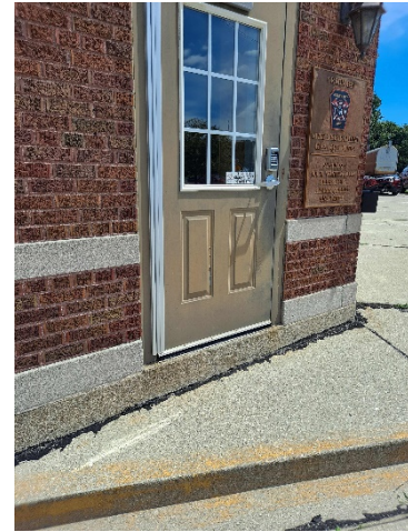
Door not egressing to grade
