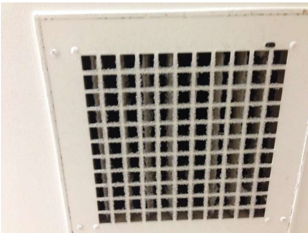
Exhaust grille (typical)
