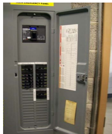
Main emergency panel
