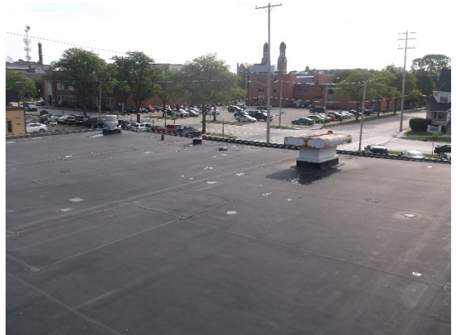
Roof drain(s), sanitary vent
