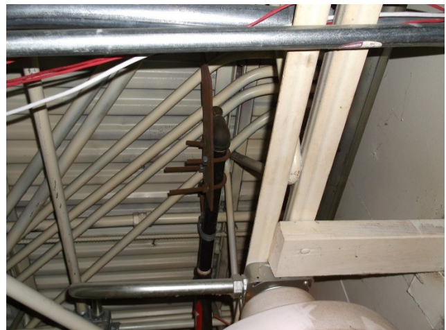
Sprinkler head with baffle in electrical room
