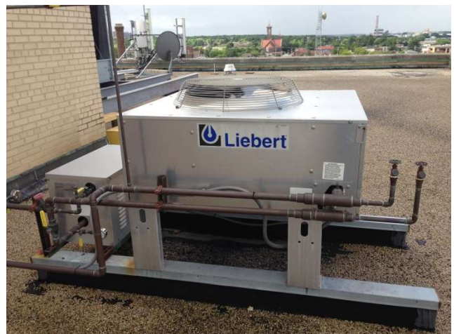
IT department condenser
