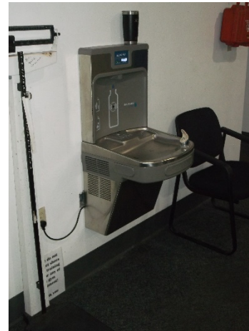
Electric water cooler – basement
