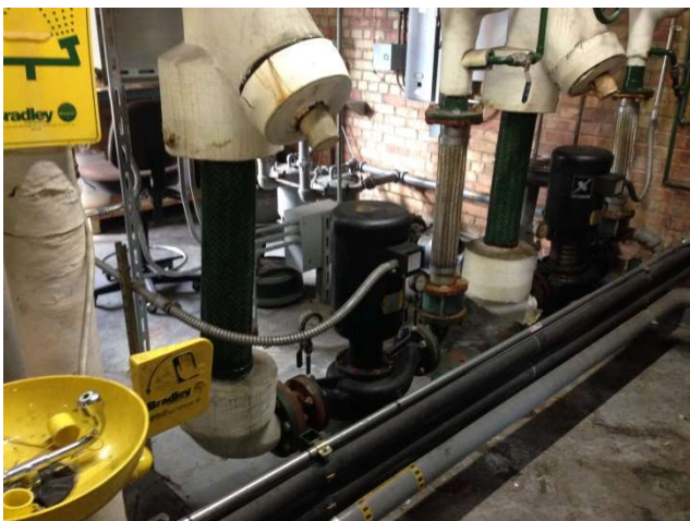
Induction unit water pumps
