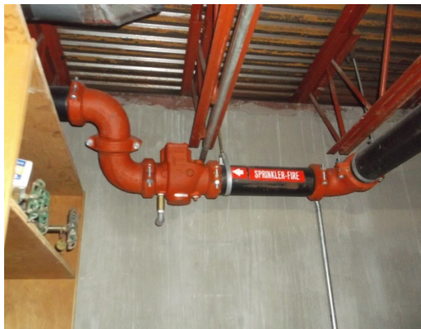
Flow direction points the wrong direction
