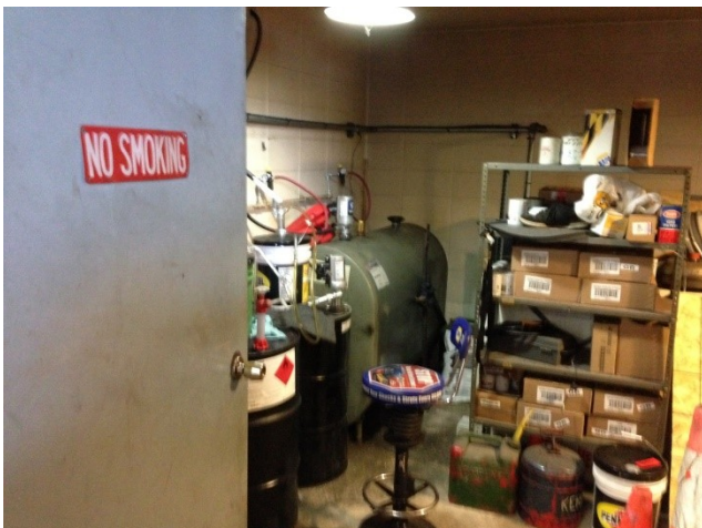
Hazardous storage room (vented tanks)
