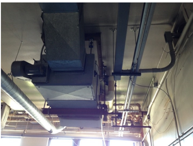
Make-up air unit
