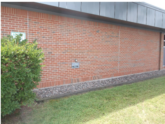
Fire department connection
