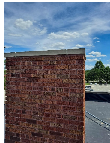
Tuck pointing needed at chimney
