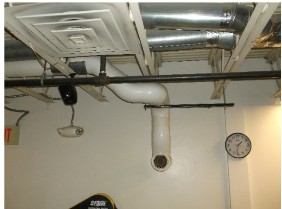
Storm piping - insulated
