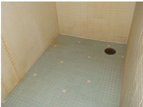
Men's shower room floor drain
