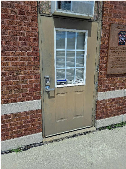
Recommend threshold at entry
