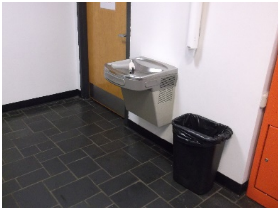
Electric water cooler – lobby
