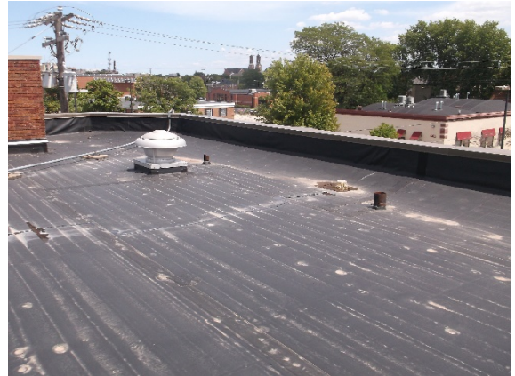
Sanitary vent & roof drain
