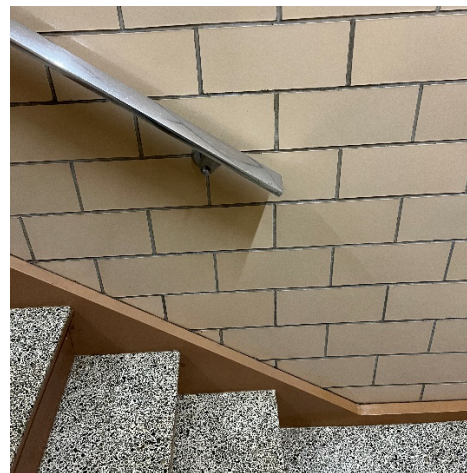
Lack of handrail extension past lowest tread
