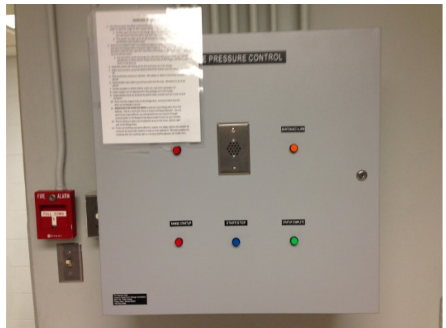
Firing range control panel
