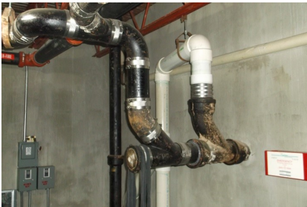
Sanitary piping (cast iron & PVC)
