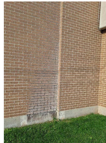
Efflorescence on brick
