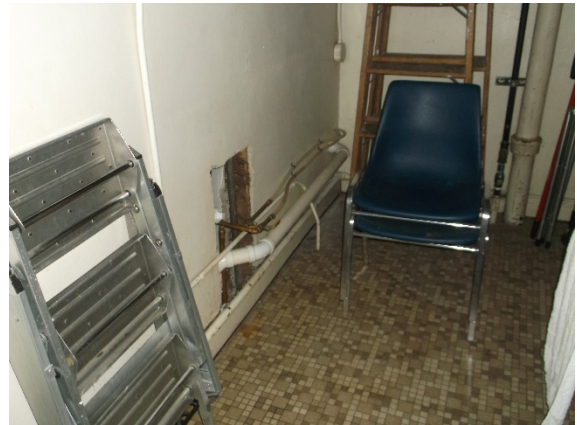
PEX piping to kitchen sink
