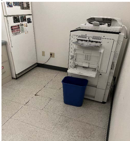
Chipped floor tiles
