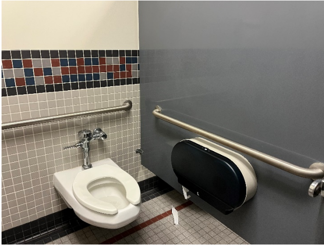
1 st floor Women's – missing vertical grab bar
