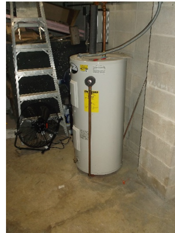
Electric water heater
