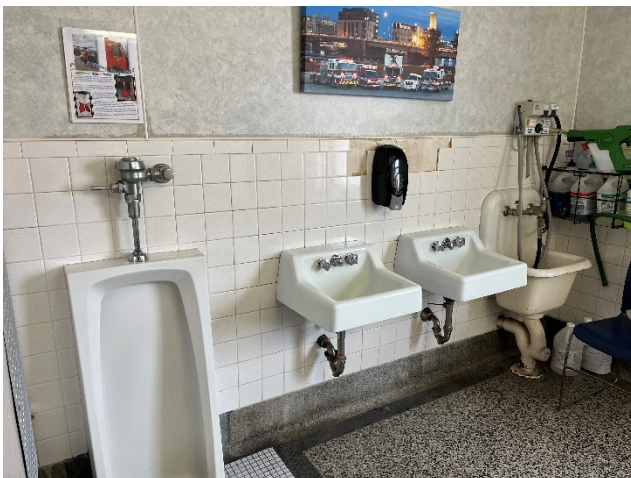
Missing wall tile at plumbing wall
