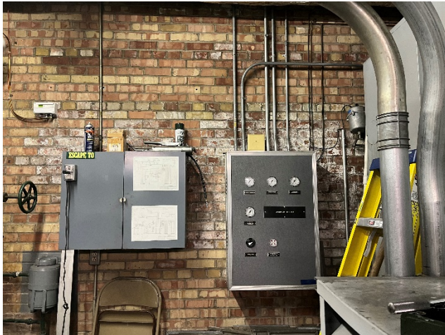
Effervescence on west wall
