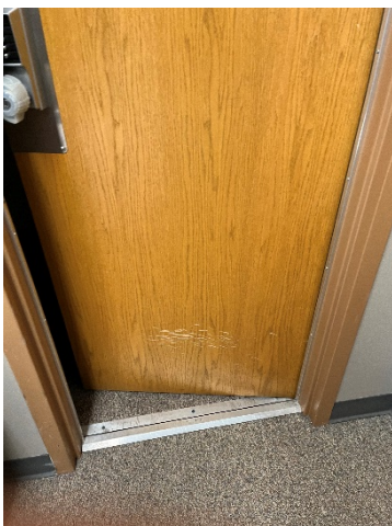
Scratched wood door
