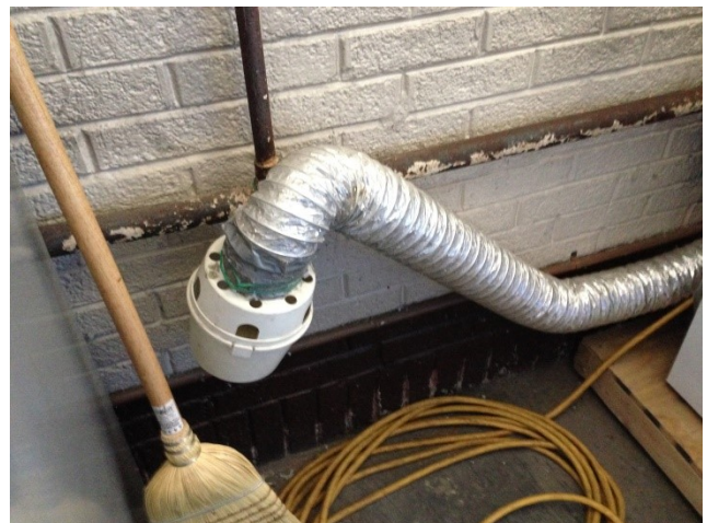
Dryer vent (indoors)
