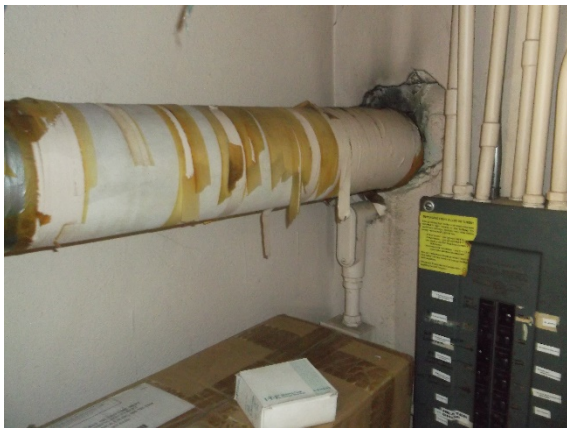
Water piping thru electrical closet
