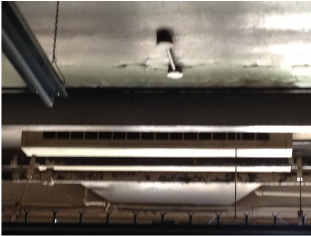
Unit ventilator (steam)
