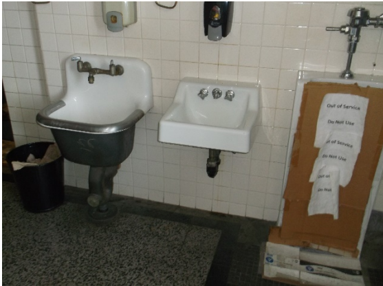
Sink, lavatory, urinal – women's
