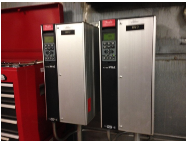
Air unit VFD's (boiler units similar)
