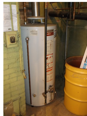
Water heater – gas fired
