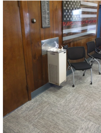
Electric water cooler- meeting room
