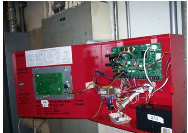
Fire alarm panel
