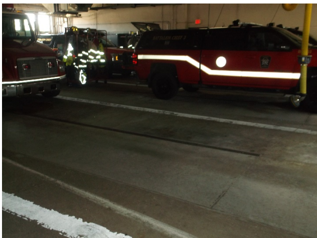
Garage trench drain
