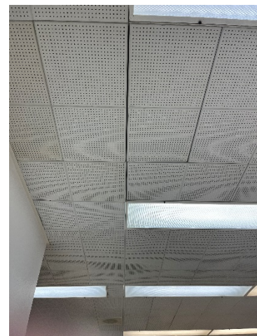
Typical spline ceiling issues
