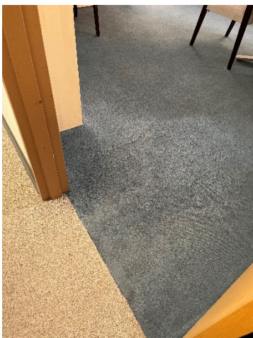
Ripped carpet seam
