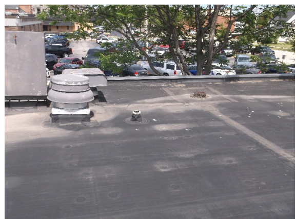
Sanitary vent & roof drain
