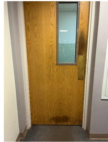
Damaged wood veneer & missing kick plate
