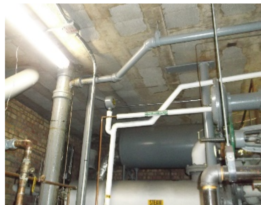
Cast iron vent piping
