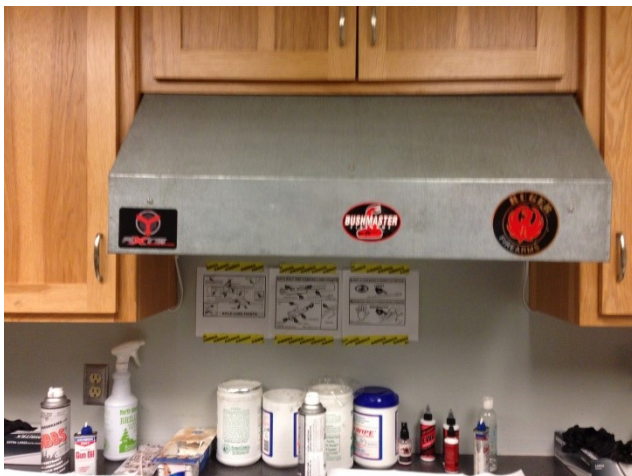
Firearm cleaning exhaust hood
