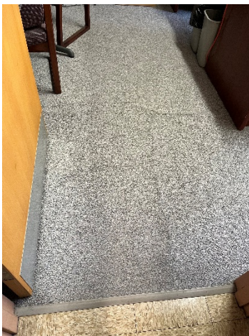
Bubbled carpet at NE office
