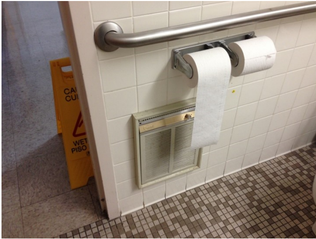
Electric heat at stairs and toilets
