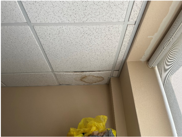
Damaged ceiling tile – adjacent to IT room
