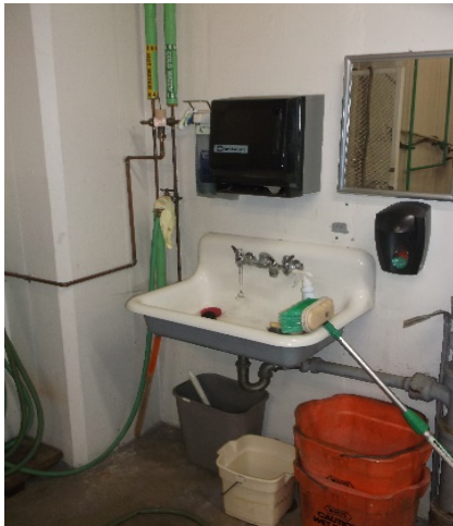
Janitors' sink – boiler room
