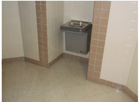
Electric water cooler
