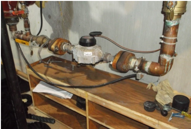
Water meter with by-pass
