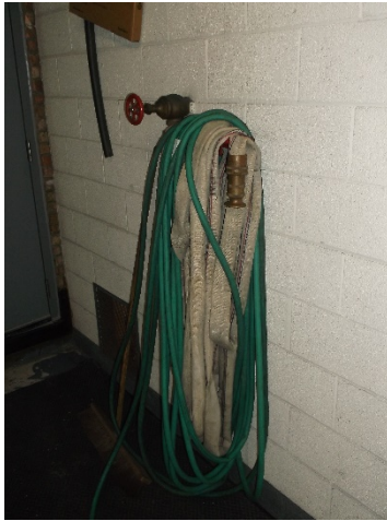
Hose valve – penthouse
