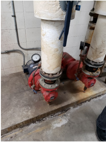
Hot water pumps
