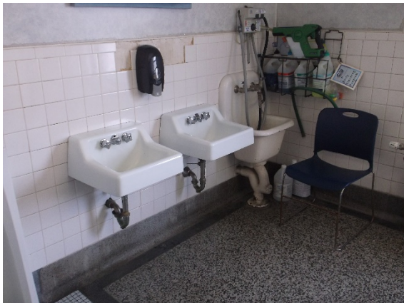
Lavatory sink – men's
