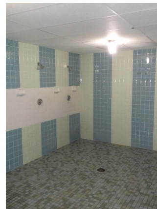
Men's shower room
