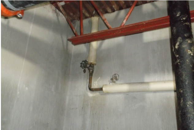
Water piping, Gate valve
