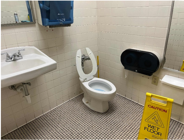
1 st Floor: not accessible toilet room
