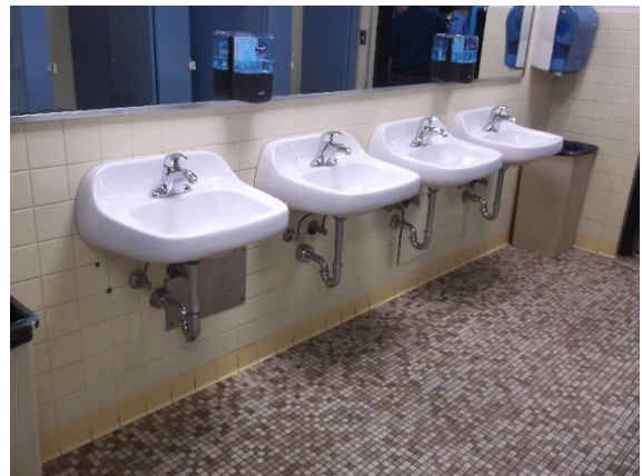
Men's toilet room lavatories
