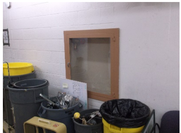
Valve cabinet - basement
