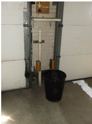
Studor vent - garage
