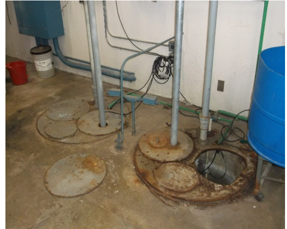
Drain tile, sanitary sump/pump
