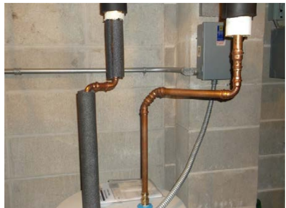
Water piping at water heater, pro-press piping
