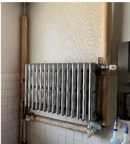
Friable insulation on piping
