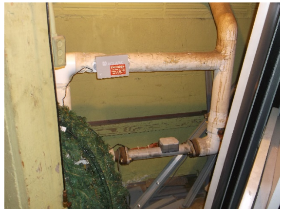
Water service, water meter with by-pass
