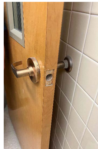
Missing latch at north stair door
