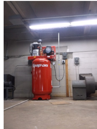
Shop air compressor
