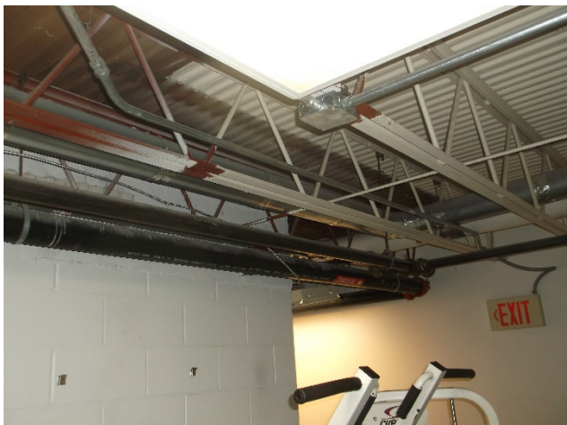
Fire protection main
