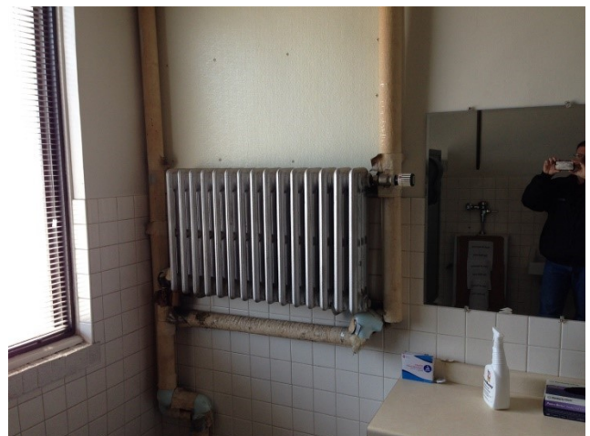
Radiator at women's toilet
