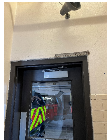
Cracked/missing plaster over door
