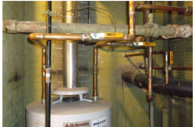
Hot/cold water piping at water heater
