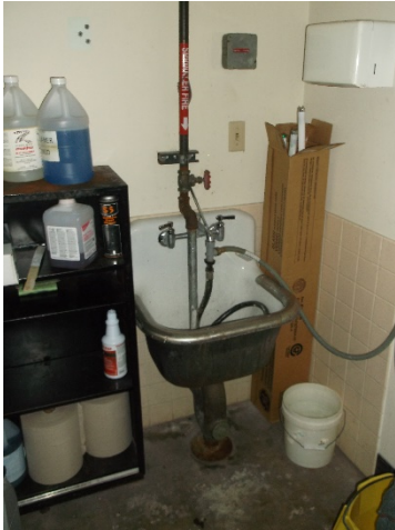
Inspector's test drain discharging in sink
