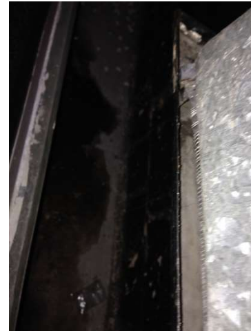
Condensation below induction unit (in wall)
