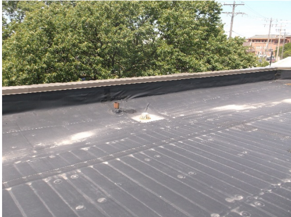
Sanitary vent & roof drain
