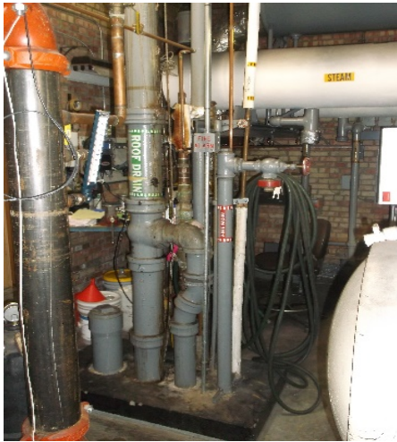
Vent, water piping in penthouse
