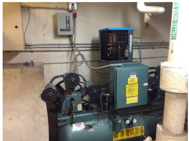
Temperature control air compressor
