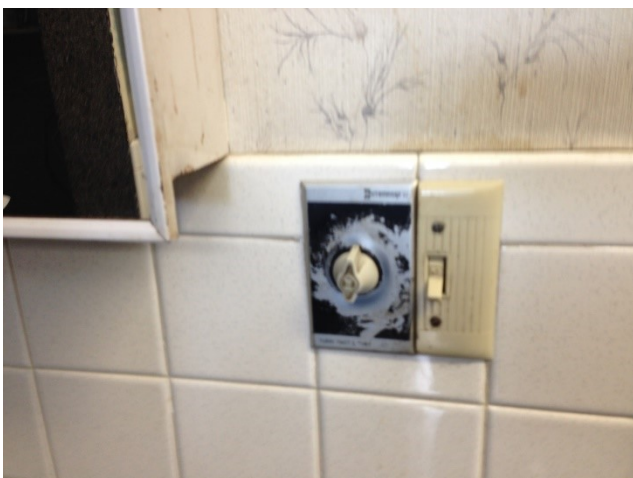
Exhaust fan manual switch (typical)
