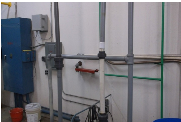
Pump discharge piping
