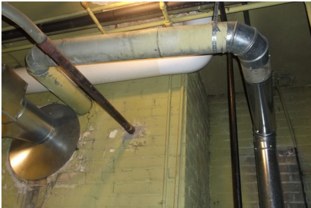
Water heater vent piping
