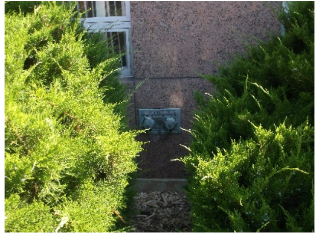
Fire dept. connection
