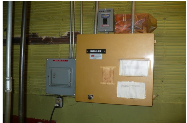
50A transfer switch
