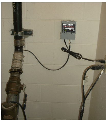
Elevator – high water alarm
