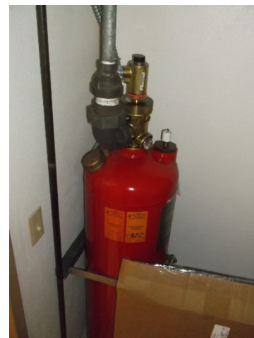
Ansul Halon 1301 – IT room
