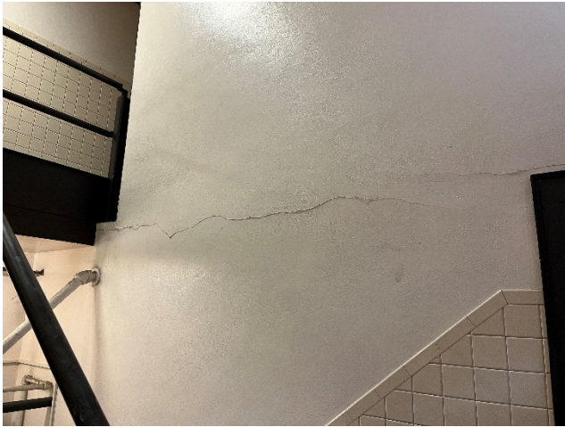
Cracked plaster at stair
