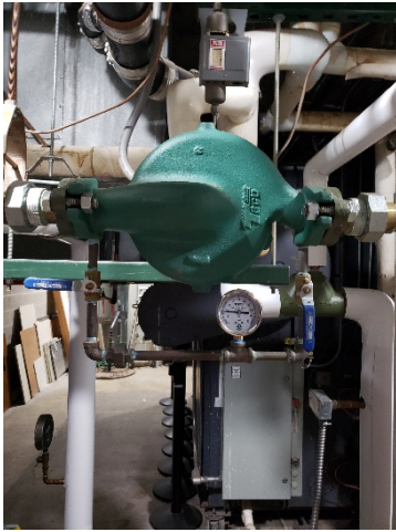
Hot water pumps
