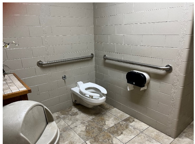
5 th floor: Typical missing vertical grab bar
