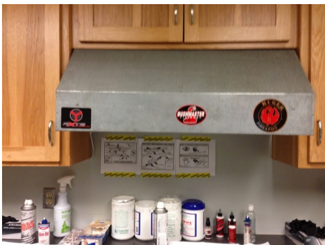
Firearm cleaning exhaust hood
