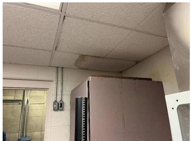
Typical stained ceiling tile
