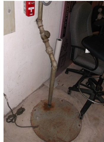
Drain tile sump/pump
