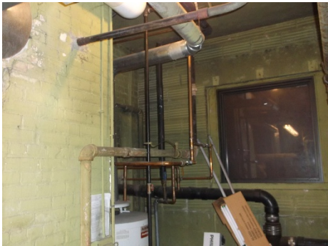
Sanitary/water piping – boiler room
