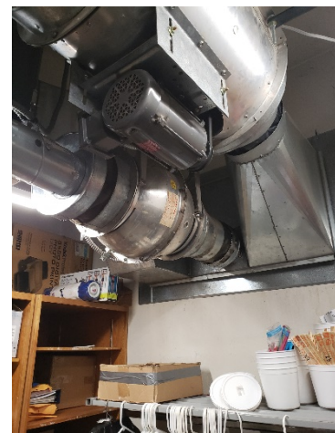
Interior exhaust fans (noisy)
