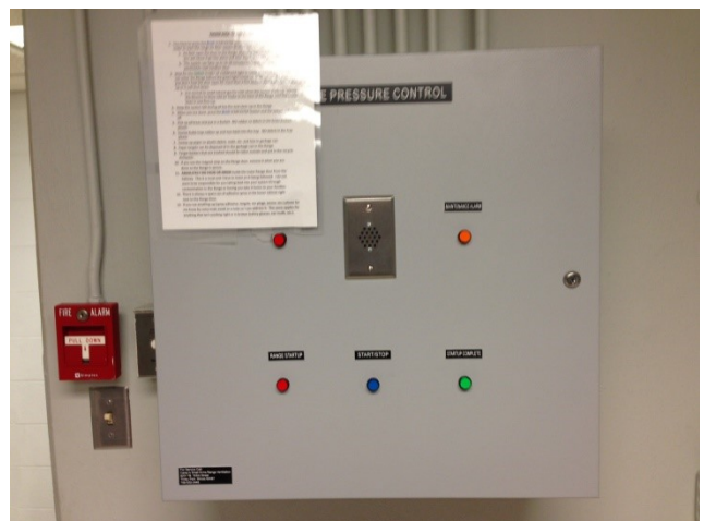
Firing range control panel
