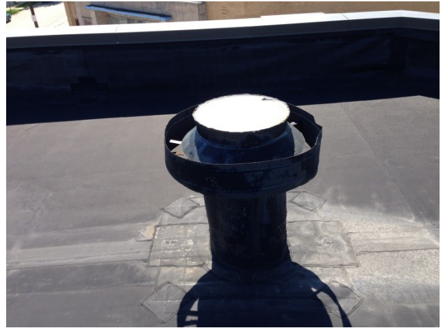
Roof exhaust hood
