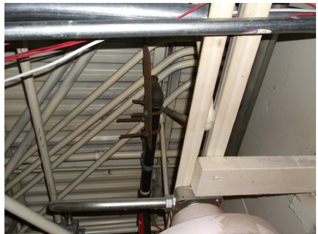
Sprinkler head with baffle in electrical room
