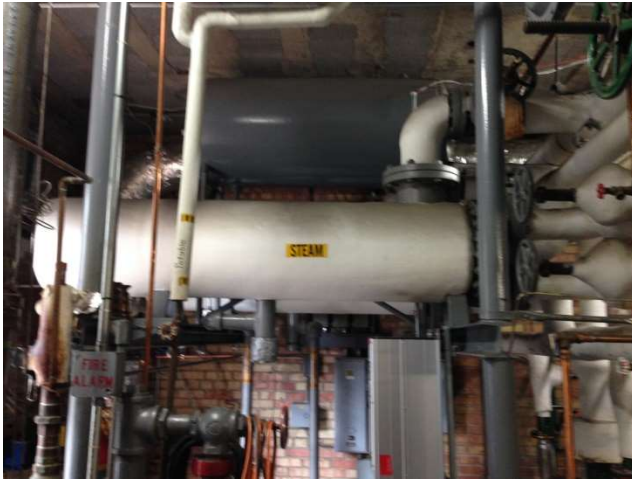
Building steam to water converters
