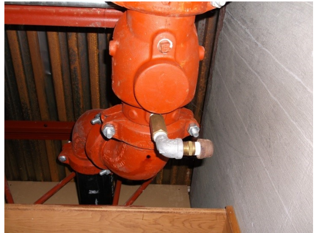
Automatic ball drip capped
