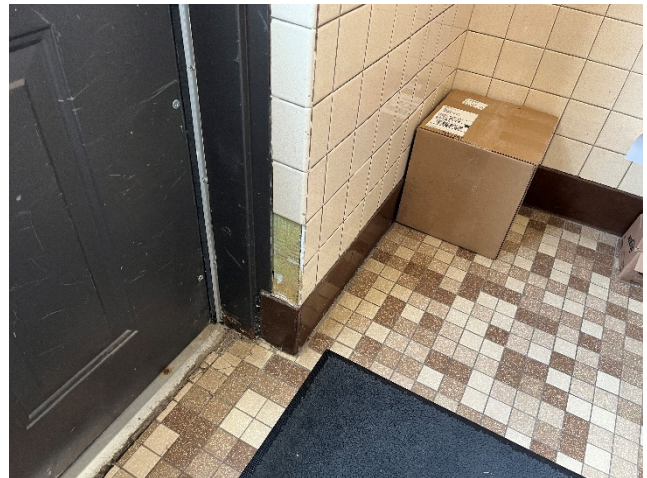
Missing wall tile
