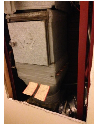
Older VAV terminal
