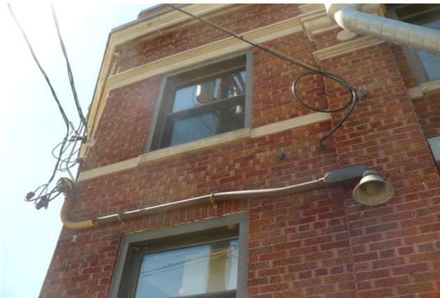
Electrical utility service entrance
