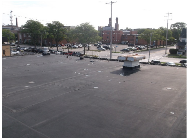
Roof drain(s), sanitary vent
