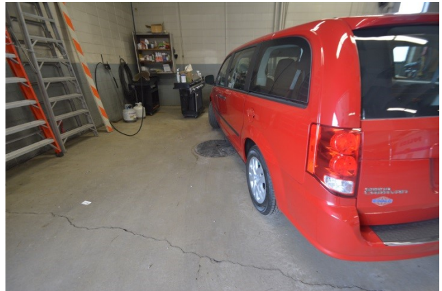
Cracked slab at garage (Note S1)
