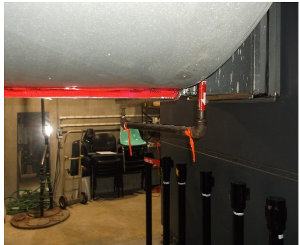
Sprinkler head under duct
