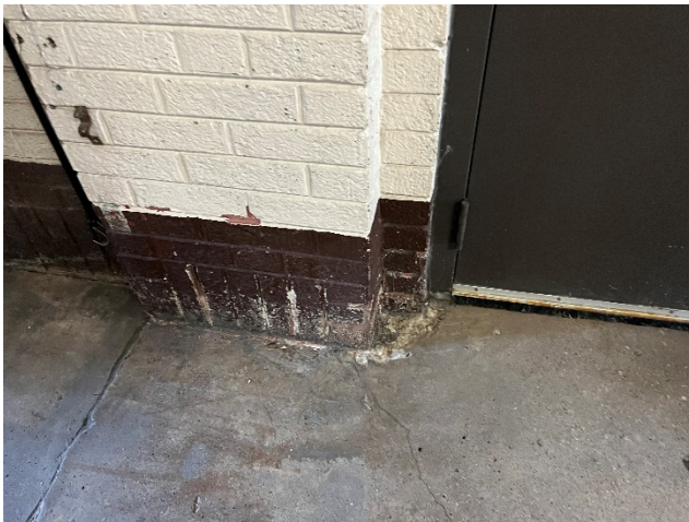
Spalling brick due to moisture exposure
