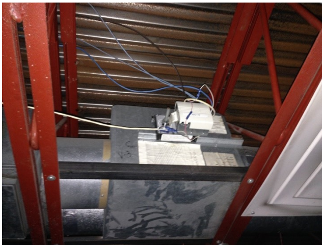
VAV terminal (no reheat)
