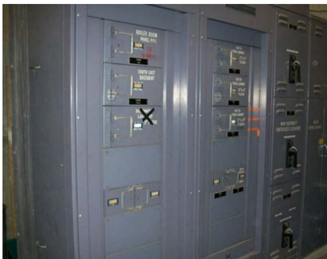
MSB main switchboard
