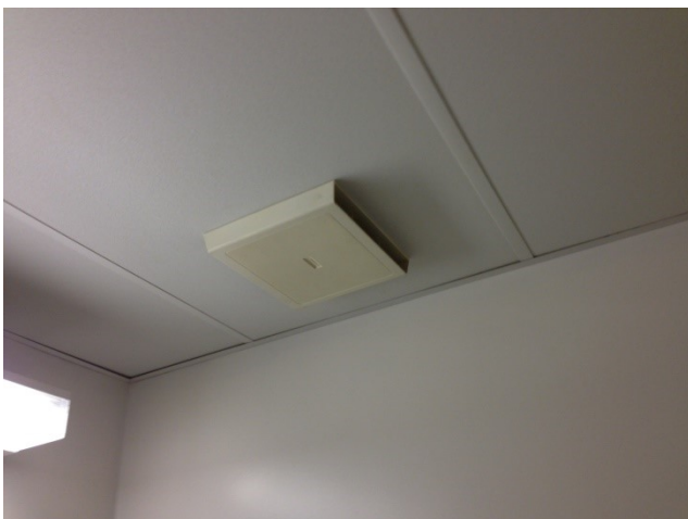
Typical ceiling exhaust fan
