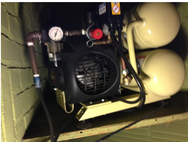
Temperature control air compressor
