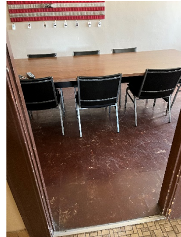
Chipped paint at wood door frame
