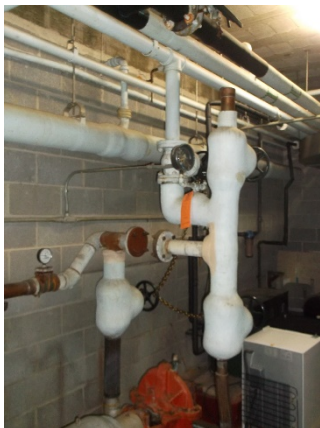
Storm and water piping
