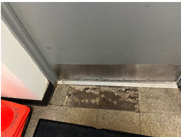
Missing vinyl tile at back door
