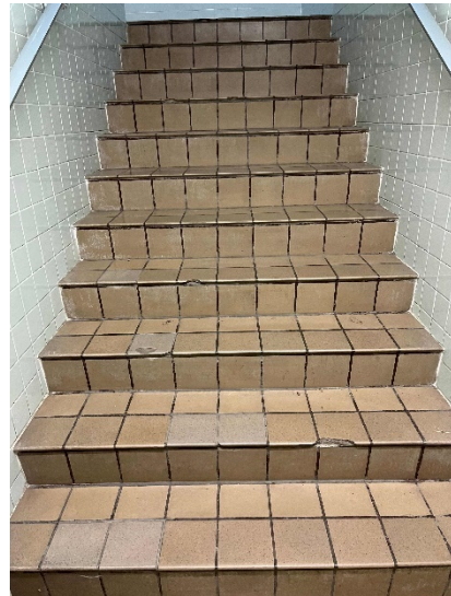
Chipped tiles at south stair
