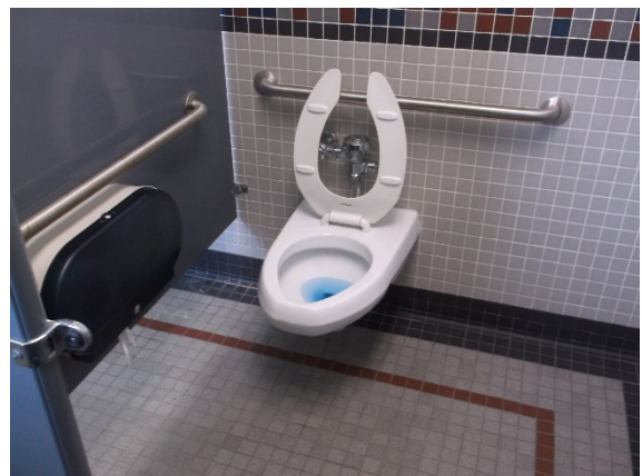
Water closet – 1 st floor public men's
