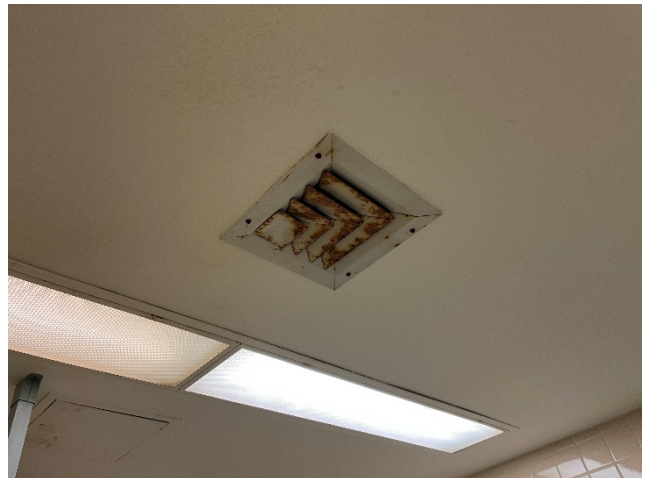
Rusted ceiling diffuser at basement toilet room
