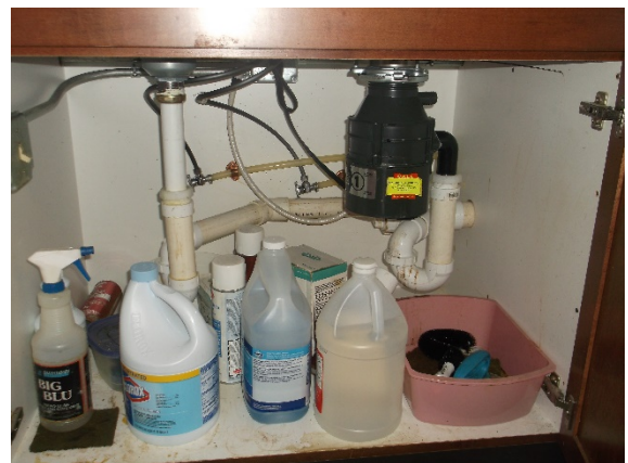
Kitchen sink – garbage disposal
