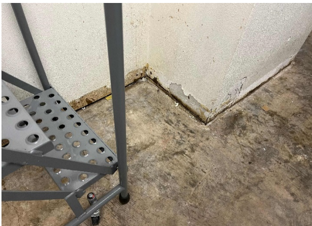
Deteriorated base at high-density storage
