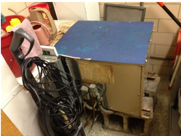
Water cooled blower coil (AHU-5)
