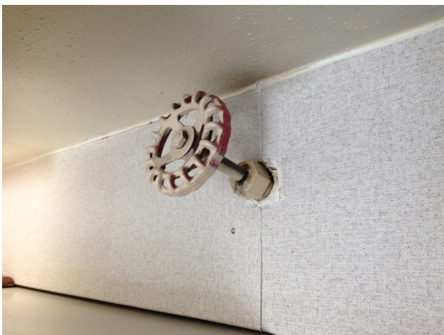
Wall built over valve
