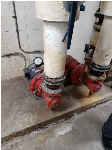
Hot water pumps
