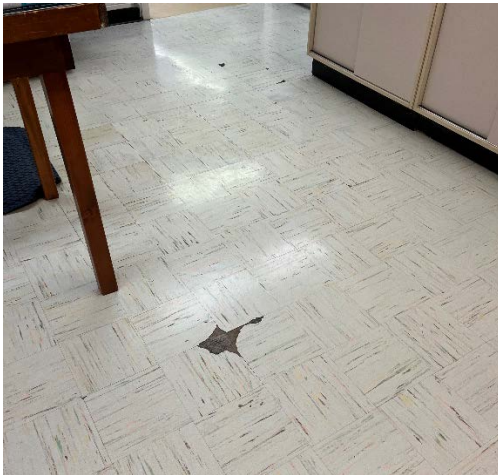
Chipped floor tile
