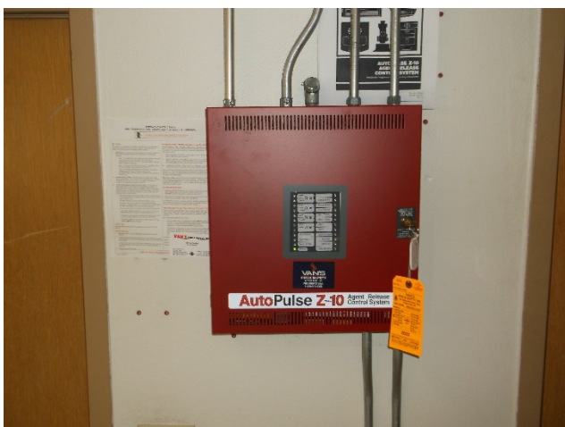
Halon control panel – IT room
