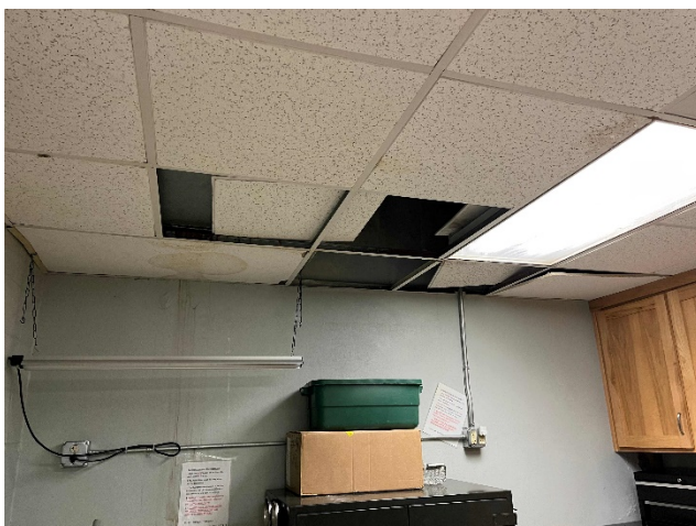
Missing and misplaced ceiling tiles
