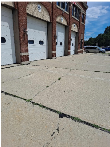
Cracked driveway apron
