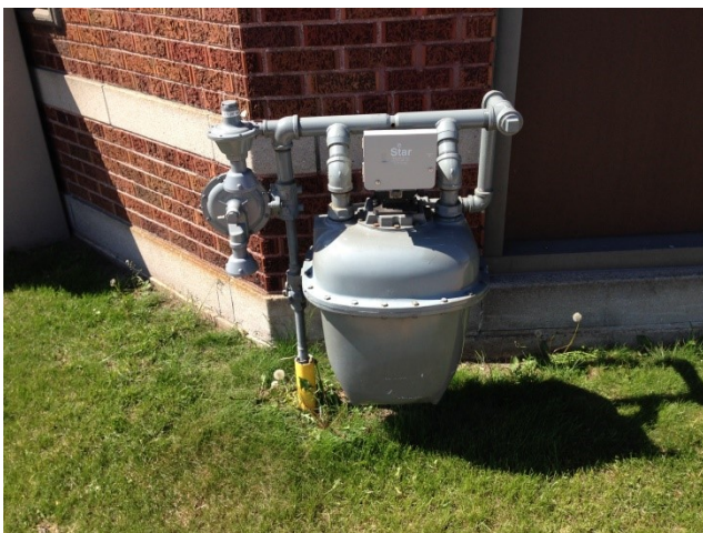
Gas meter (intake louver out of frame)
