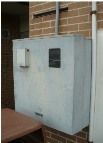
Main electrical service meter
