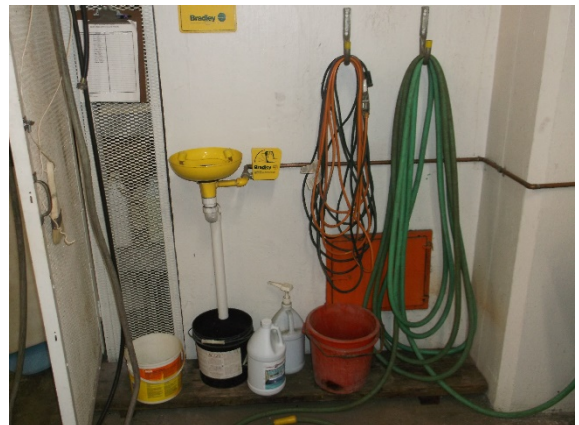
Eyewash – boiler room
