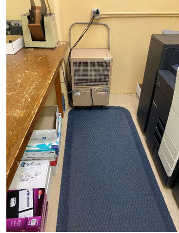
Print room dehumidification (humidity issues)
