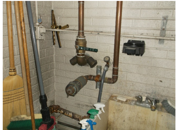
Fill connection(s) in garage
