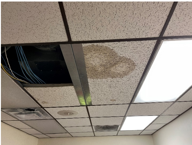
Missing and stained ceiling tile
