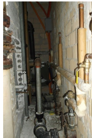
Piping in toilet chase – typical
