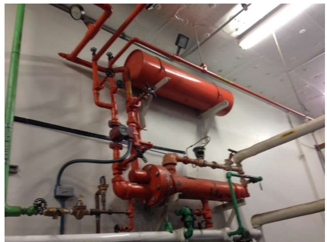
Basement hot water system
