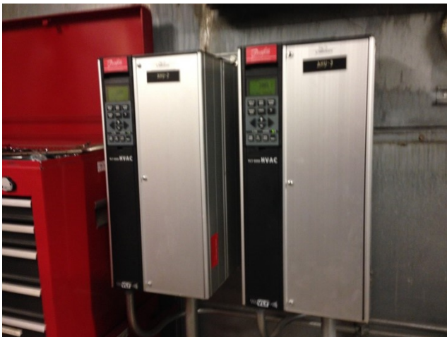
Air unit VFD's (boiler units similar)
