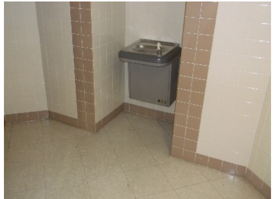
Electric water cooler
