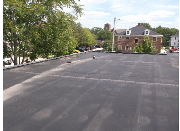
Sanitary vent & roof drain
