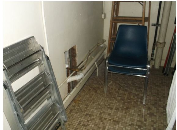
PEX piping to kitchen sink
