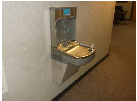
Electric water cooler
