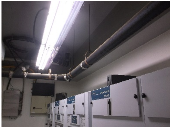
Sanitary piping over evidence dryers
