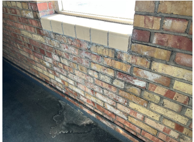
Effervescence on east wall
