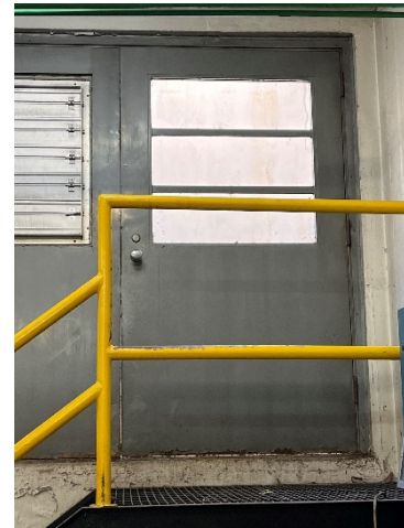
Missing weatherstripping at rusted door
