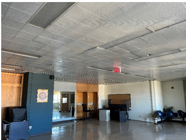
Typical spline ceiling issues
