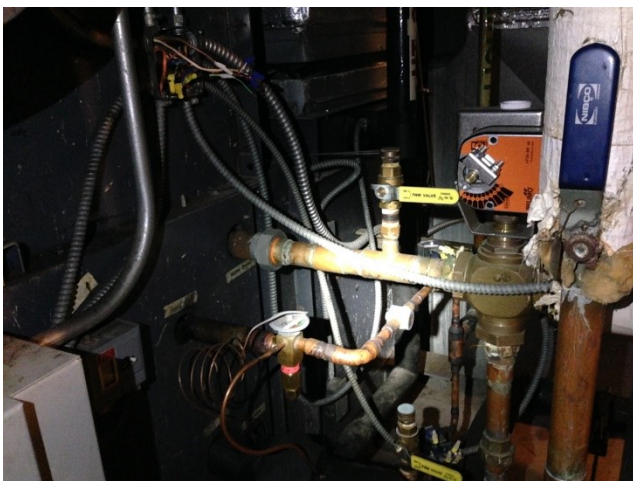
Air unit coils
