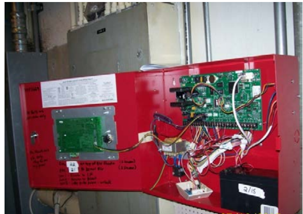
Fire alarm panel
