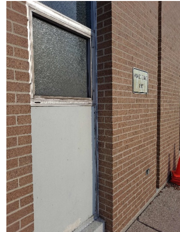
Faded window infill panels
