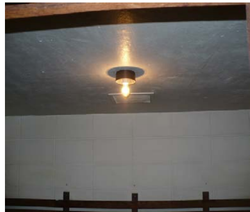
Sauna light missing lens
