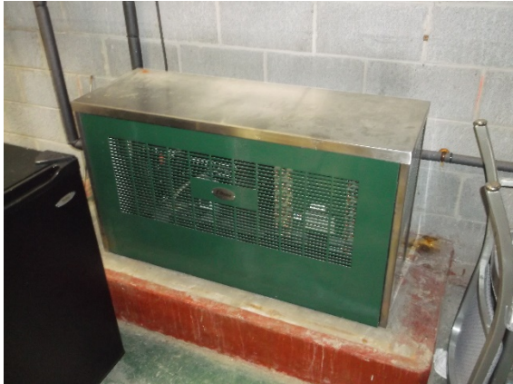
Chiller for drinking fountain(s)
