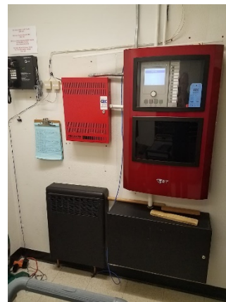
Fire alarm panel
