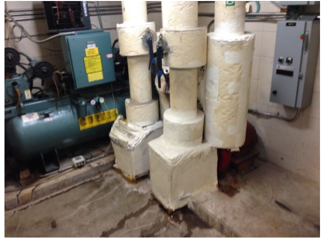
Chilled water pumps
