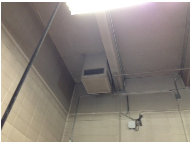
Garage exhaust (near ceiling)
