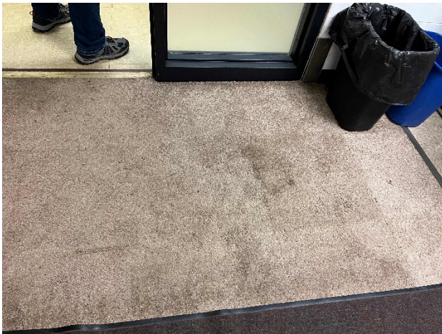
Worn, stained cut-pile carpet
