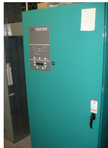
Automatic transfer switch
