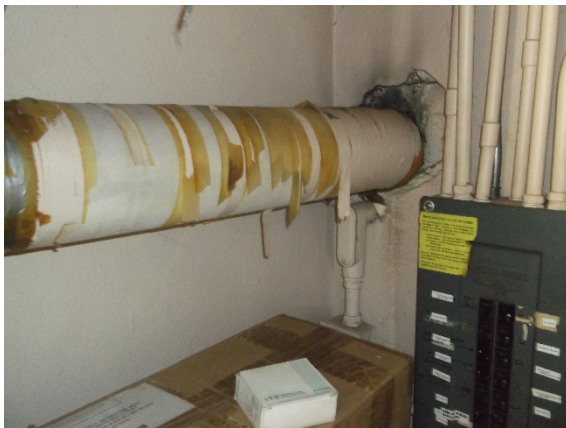
Water piping thru electrical closet
