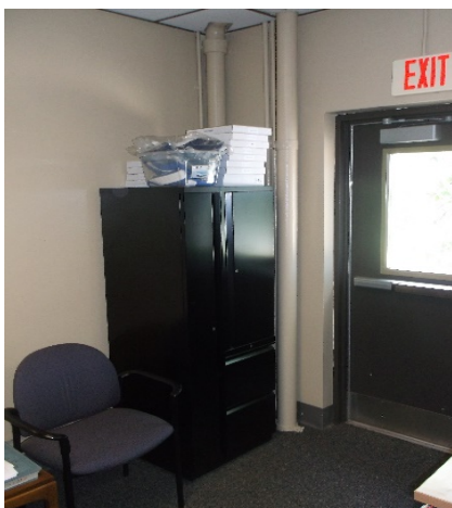
Storm piping, sanitary vent
