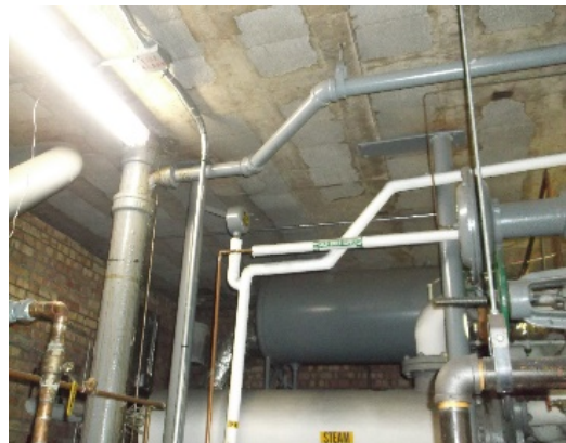
Cast iron vent piping
