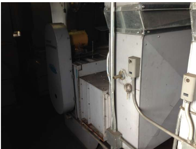
AHU-2 and AHU-3
