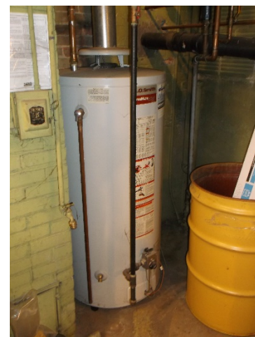
Water heater – gas fired
