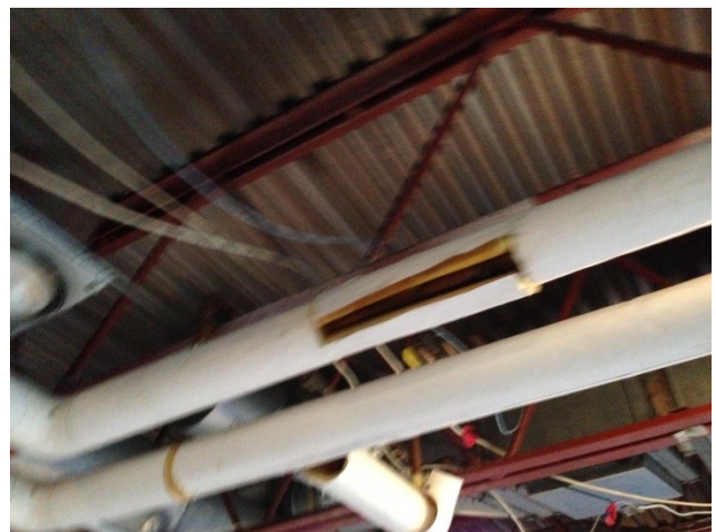
Poor insulation (typical)
