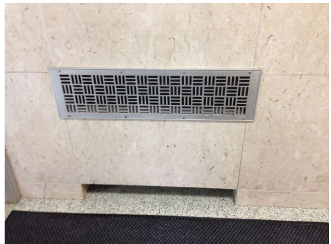
Vestibule heater (typical)
