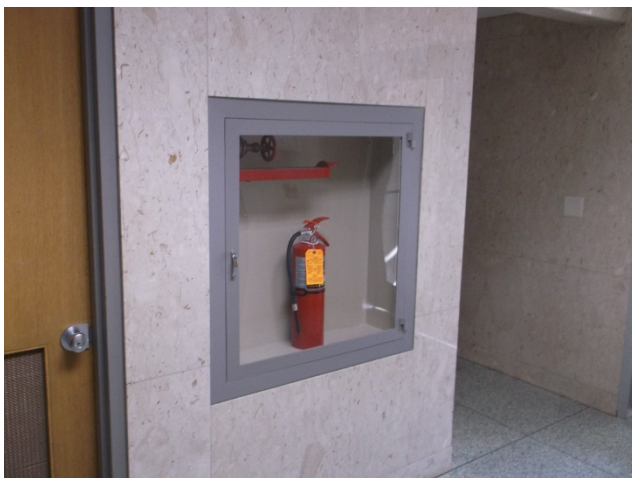
Hose valve cabinet
