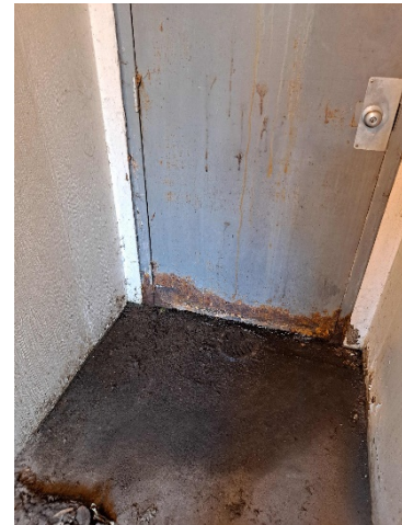
Rusted door to window well
