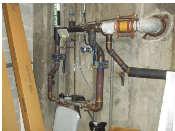
2" water meter, 4" water main
