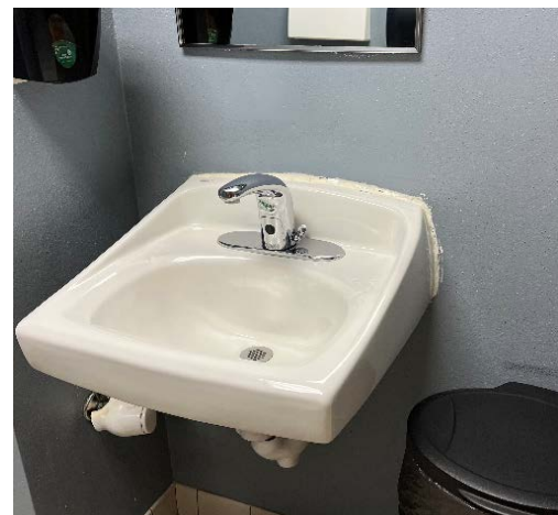
Excessive sealant at lavatory
