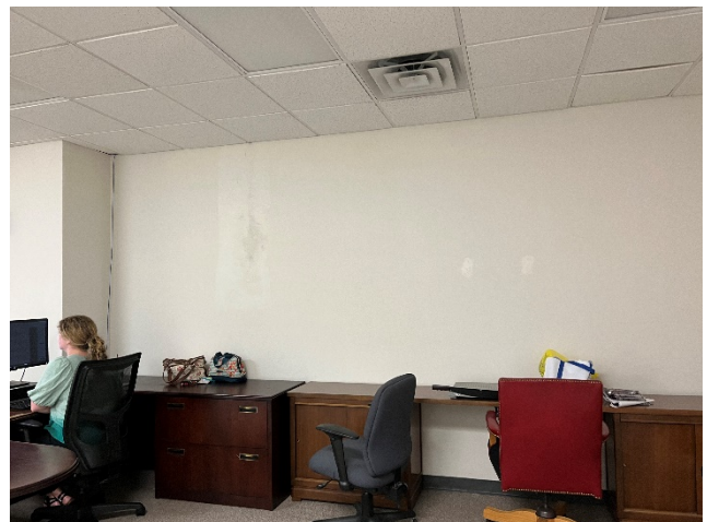
Visible wall patches
