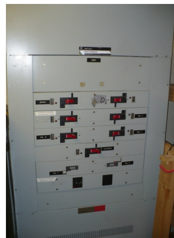
Normal main distribution panel
