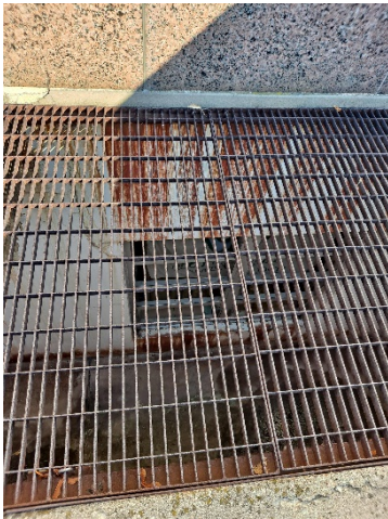
Rust on window well walls
