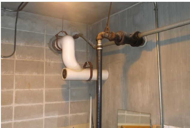
Storm piping, drain tile pump discharge
