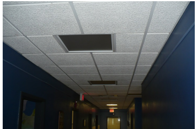
1 st floor corridor lighting
