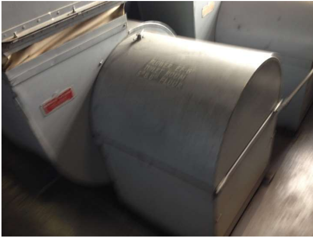
Typical exhaust fan
