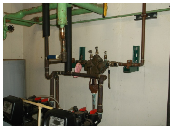
RPZ backflow preventer
