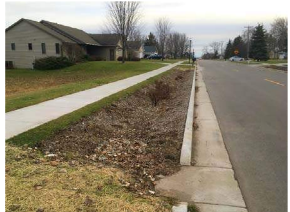
Biofilters located in the terrace
