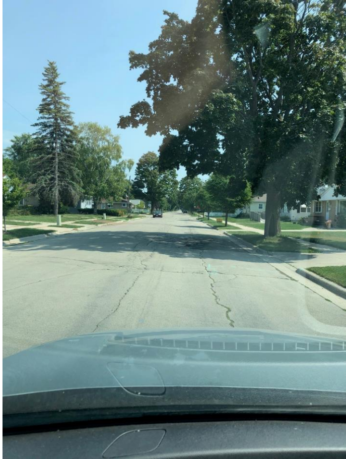
Eastbound Bond at approaching Wilson No Stop Advance sign. At time Stop condition was visible since that time forestry has planted crab apple trees in terrace
