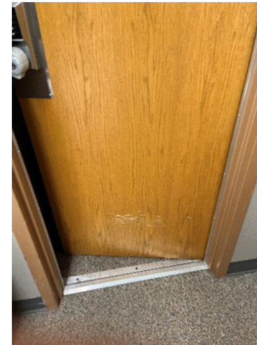
Scratched wood door
