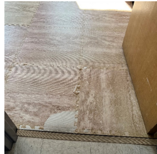
De-laminated interlocking floor tiles
