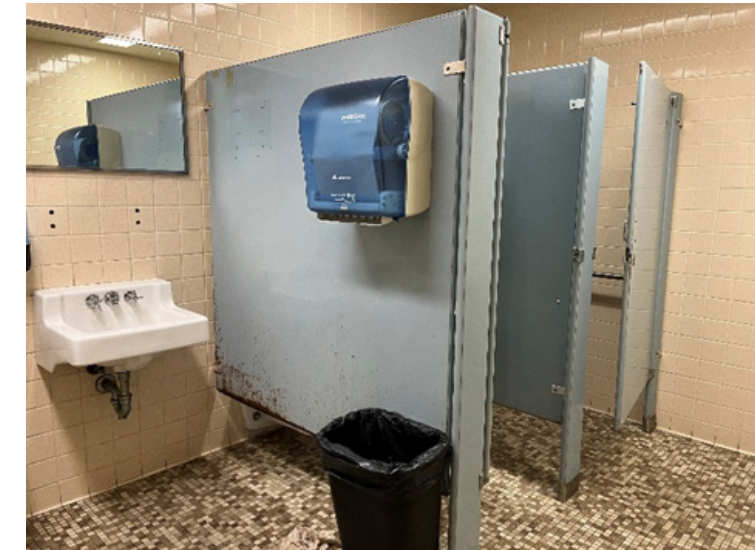
Rusted bottom of men's toilet partitions
