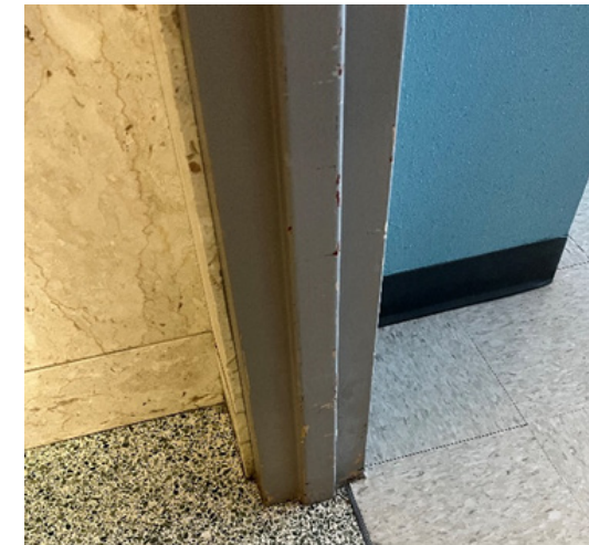
Chipped paint at HM frames
