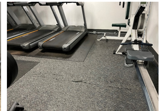
Ripped carpet at cardio room
