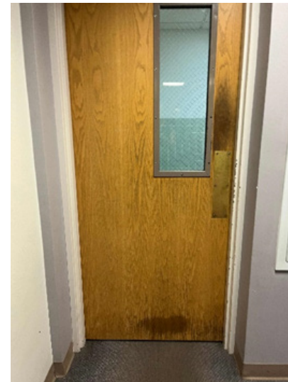
Damaged wood veneer & missing kick plate
