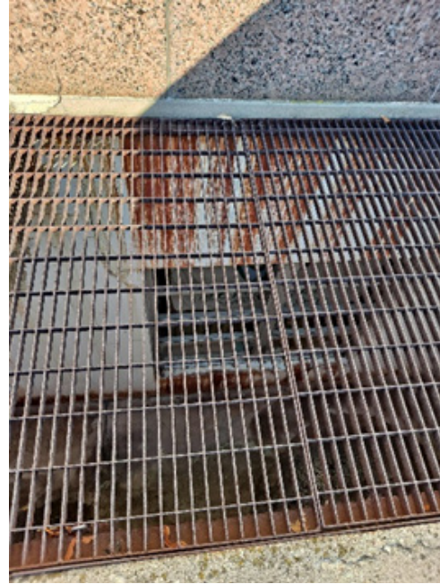
Rust on window well walls
