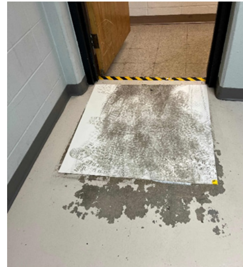
Chipped paint at shooting gallery entry
