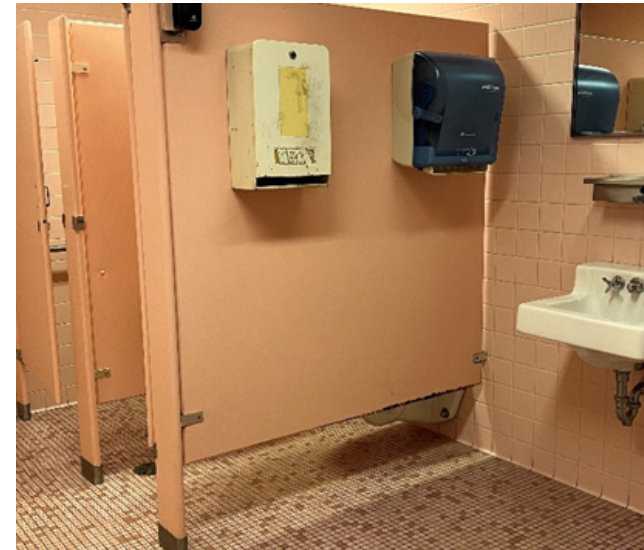
Rusted bottom of women's toilet partitions
