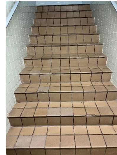
Chipped tiles at south stair
