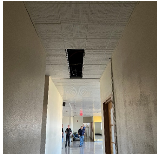
Missing light fixture
