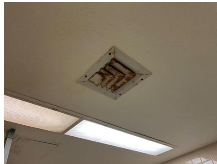
Rusted ceiling diffuser at basement toilet room
