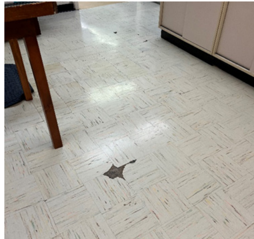
Chipped floor tile
