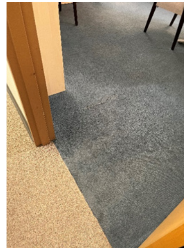
Ripped carpet seam
