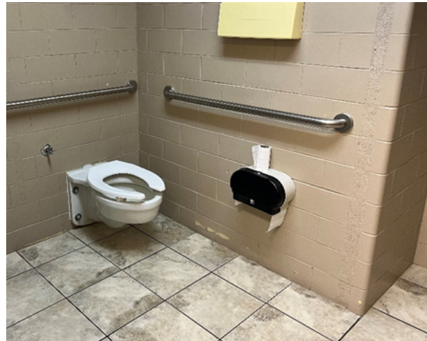
Peeling paint from glazed block
