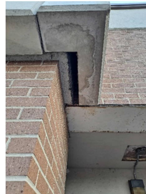
Gaps under precast concrete panels
