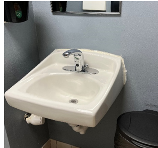
Excessive sealant at lavatory
