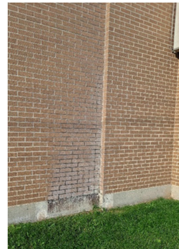
Efflorescence on brick
