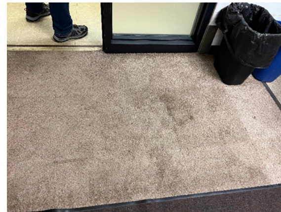
Worn, stained cut-pile carpet
