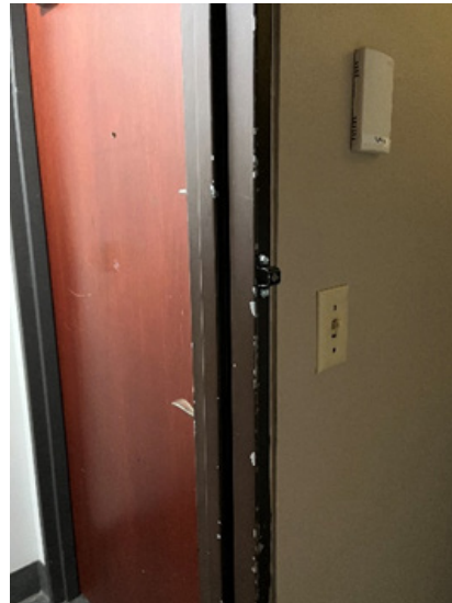
Chipped paint at basement door frames
