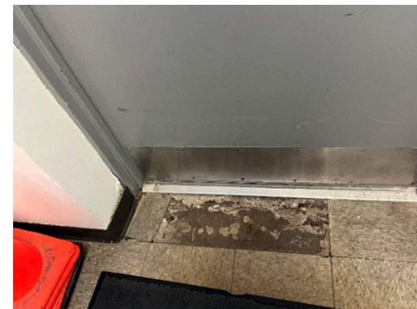
Missing vinyl tile at back door
