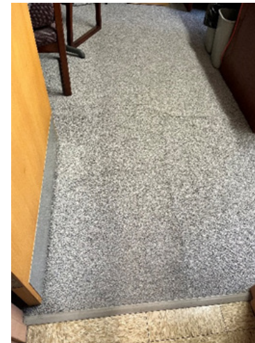
Bubbled carpet at NE office
