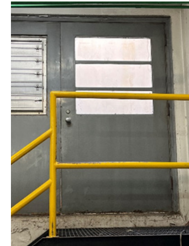
Missing weatherstripping at rusted door
