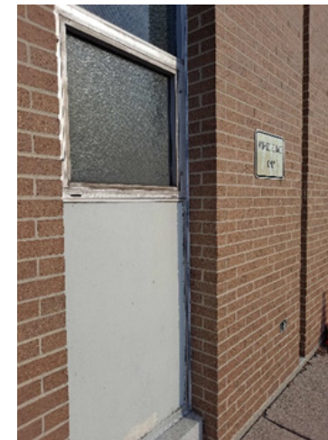
Faded window infill panels
