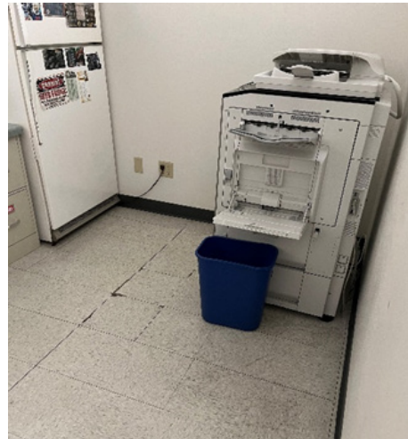
Chipped floor tile
