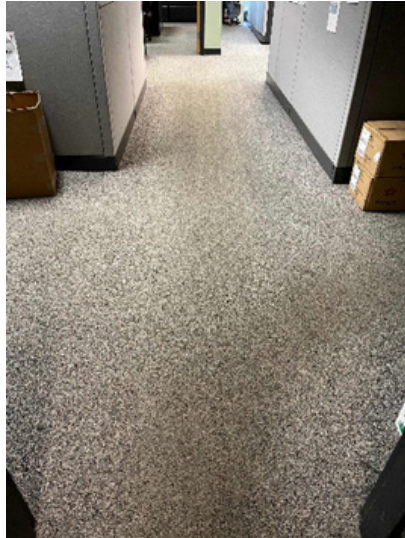
Worn carpet at office area
