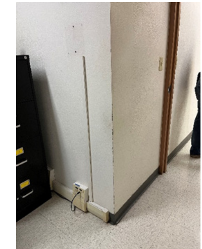
2nd & 3rd floors: typical chipped paint at exterior corner
