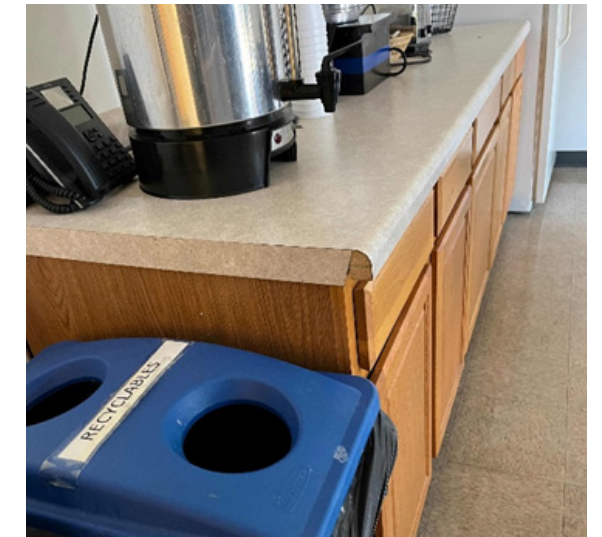
Chipped plastic laminate
