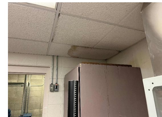
Typical stained ceiling tile
