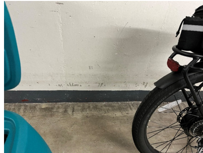
Chipped paint at wall
