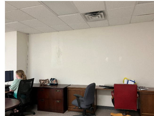
Visible wall patches
