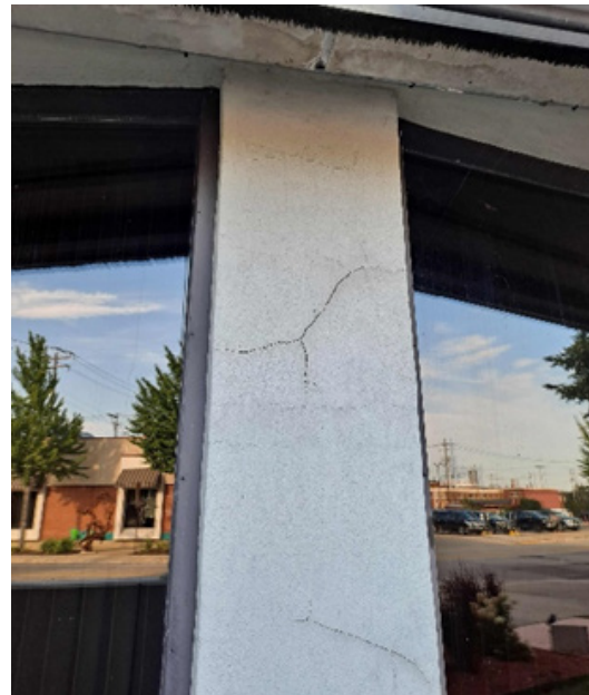
Cracked concrete between windows
