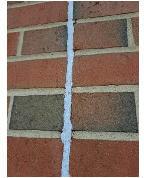
Dried and cracking expansion joint material
