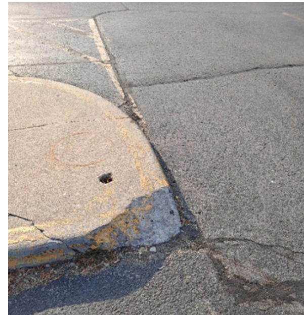
Damaged concrete curb
