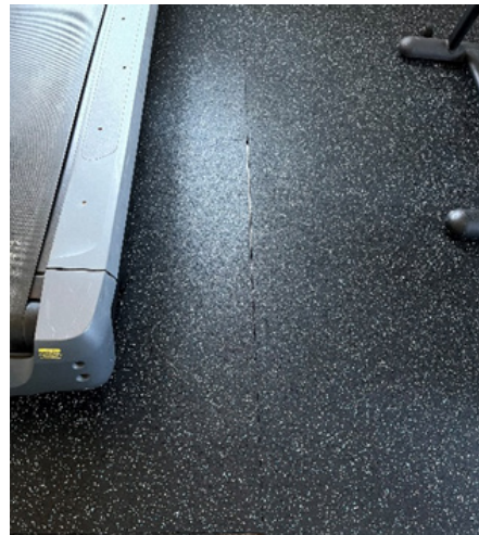
Gap in rubber floor tile
