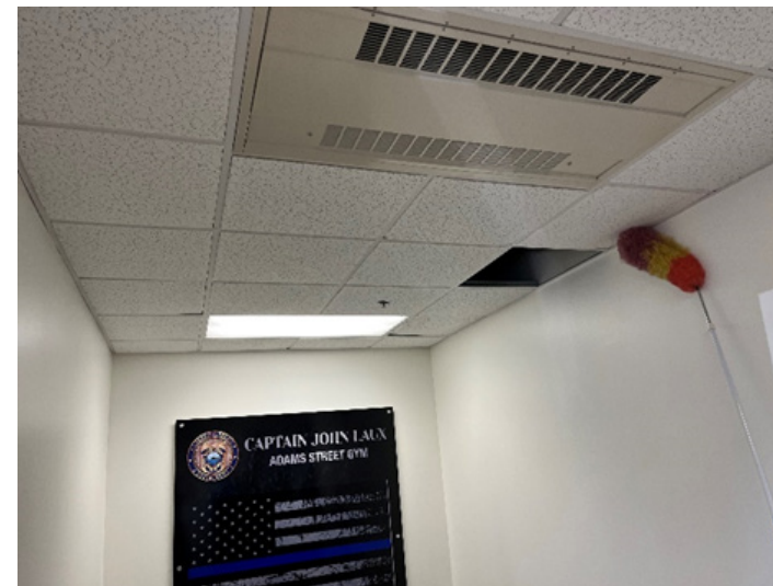
Missing ceiling tile at back stair shaft
