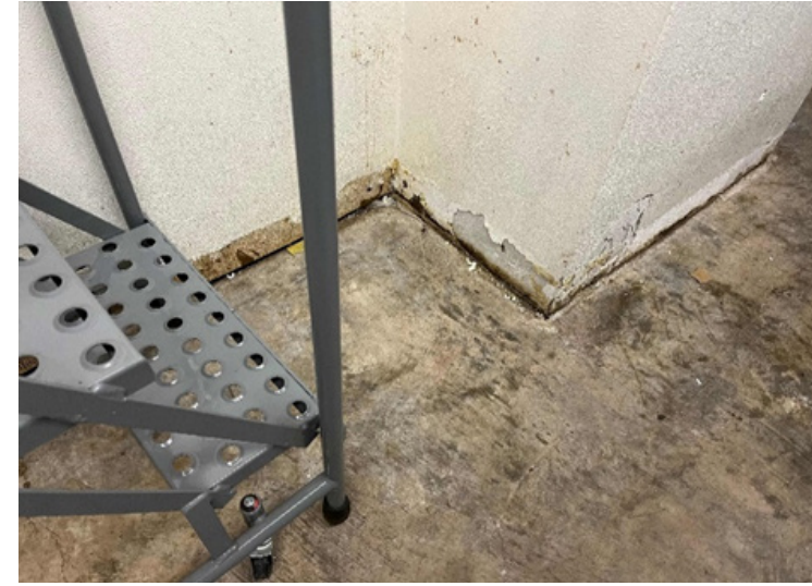
Deteriorated base at high-density storage
