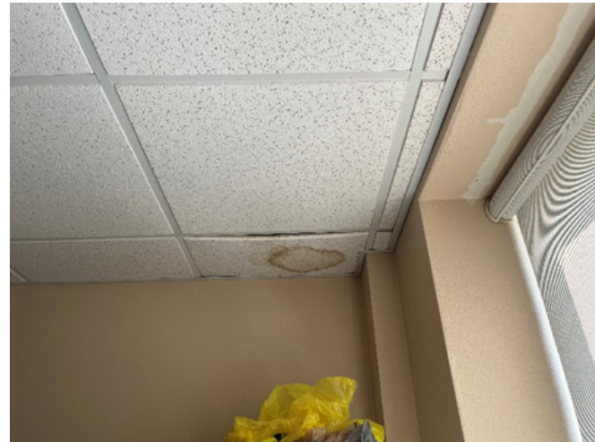
Damaged ceiling tile – adjacent to IT room
