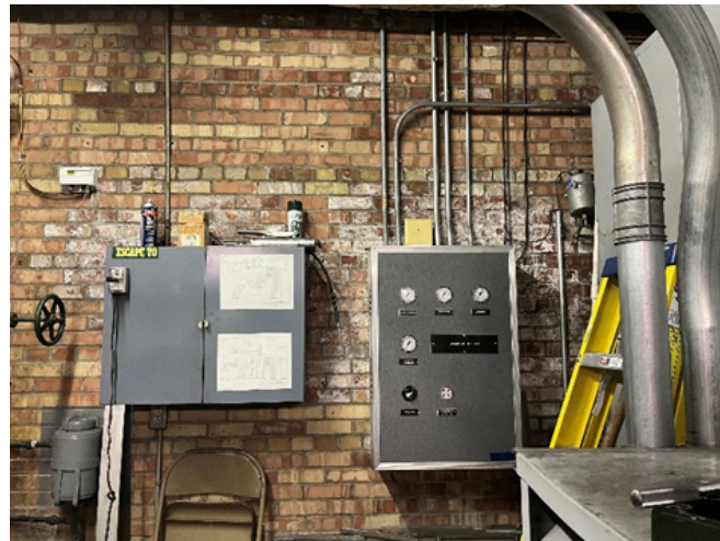
Efflorescence on west wall
