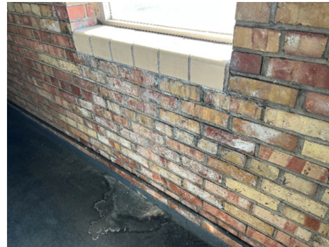
Efflorescence on east wall
