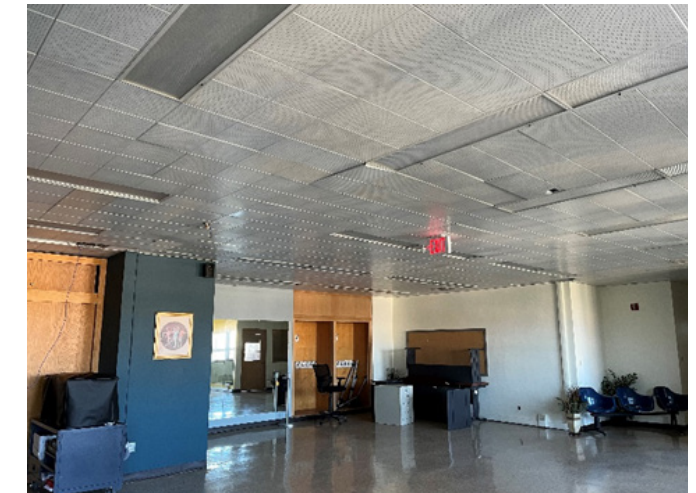
Typical spline ceiling issues
