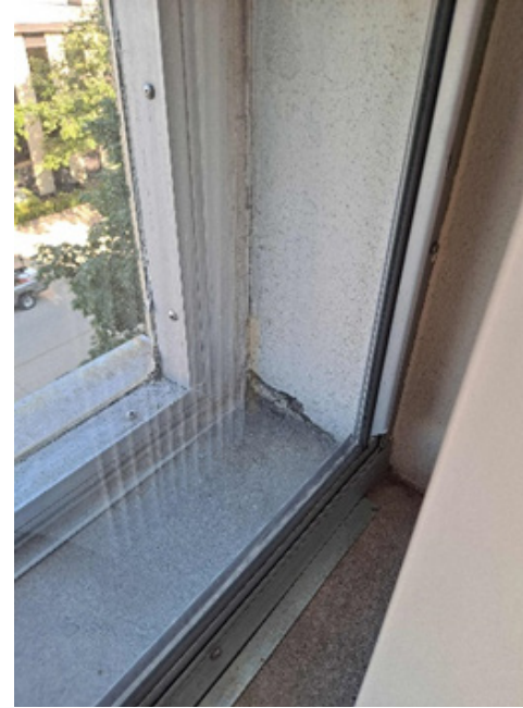
Rust on window well walls
