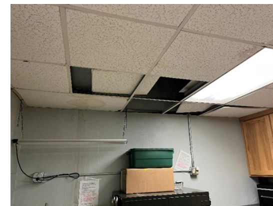
Missing and misplaced ceiling tiles
