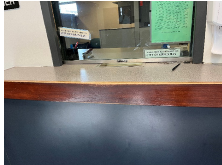
Worn finish at reception counter
