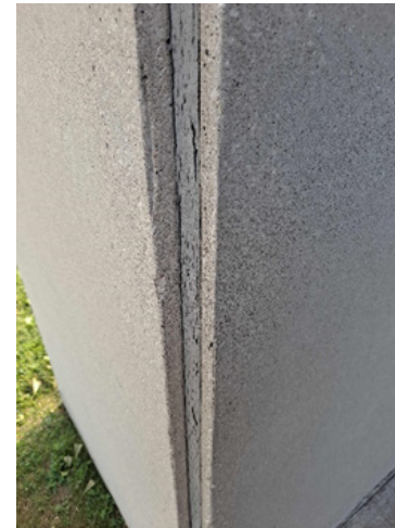
Caulking dried and brittle
