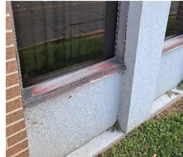
Faded metal window trim
