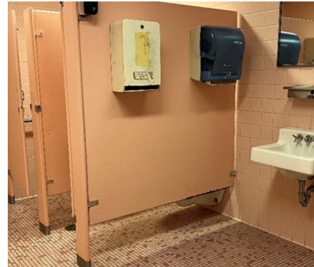
Rusted bottom of women's toilet partitions
