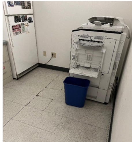
Chipped floor tile
