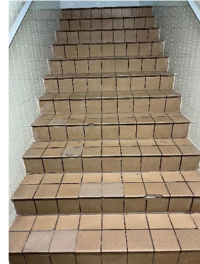
Chipped tiles at south stair
