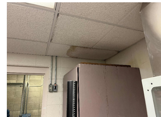
Typical stained ceiling tile
