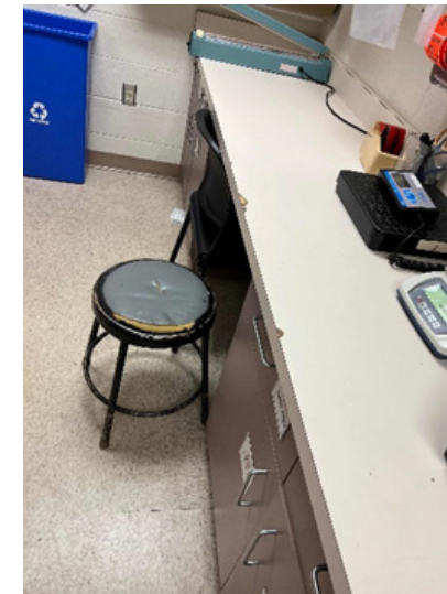
Plastic laminate casework condition
