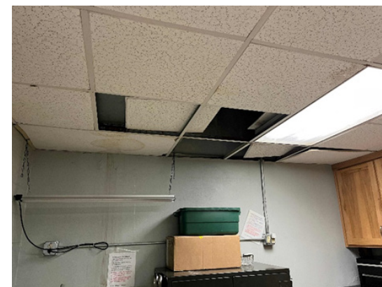
Missing and misplaced ceiling tiles
