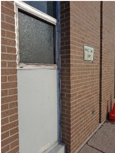
Faded window infill panels
