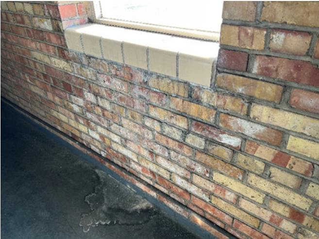
Efflorescence on east wall
