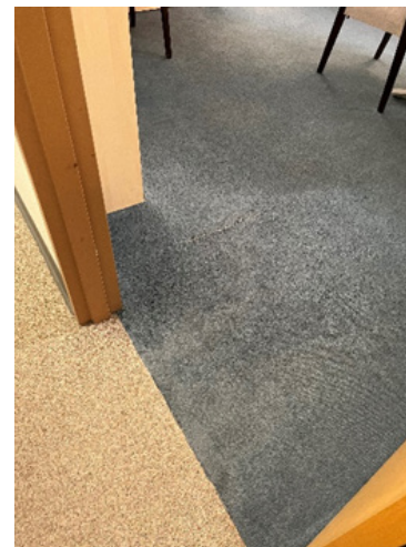
Ripped carpet seam
