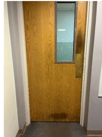
Damaged wood veneer & missing kick plate
