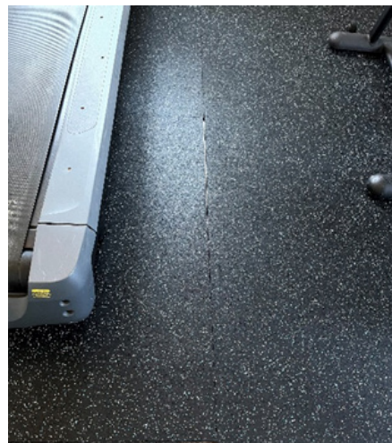
Gap in rubber floor tile
