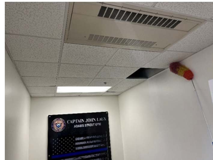
Missing ceiling tile at back stair shaft
