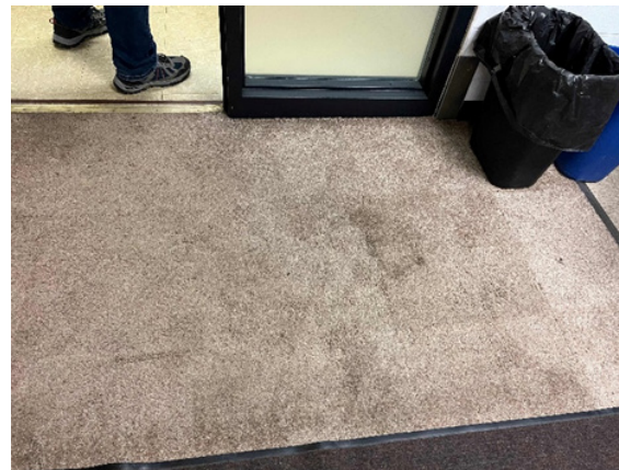
Worn, stained cut-pile carpet
