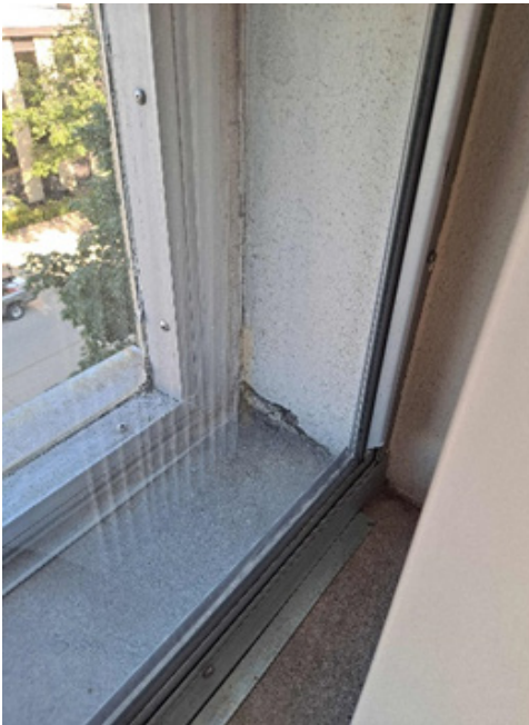
Rust on window well walls
