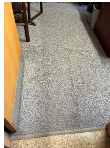
Bubbled carpet at NE office
