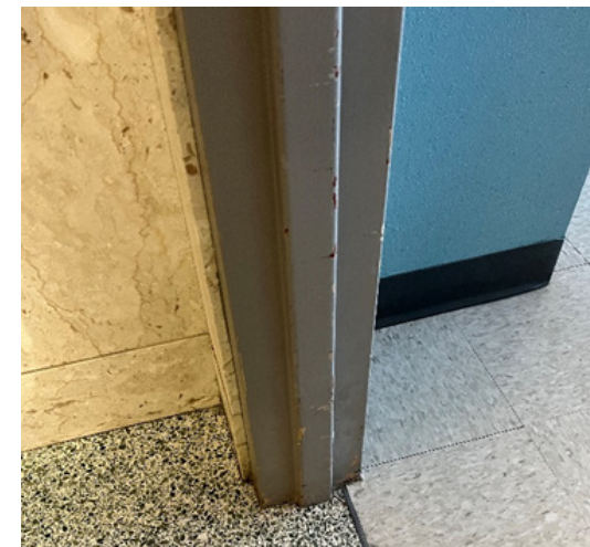
Chipped paint at HM frames
