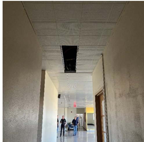
Missing light fixture
