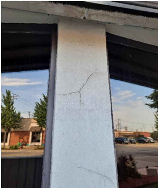
Cracked concrete between windows
