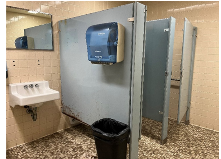
Rusted bottom of men's toilet partitions
