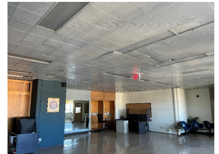
Typical spline ceiling issues
