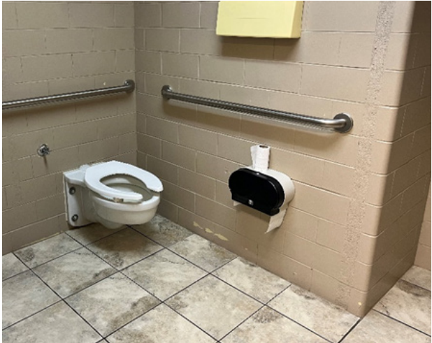
Peeling paint from glazed block
