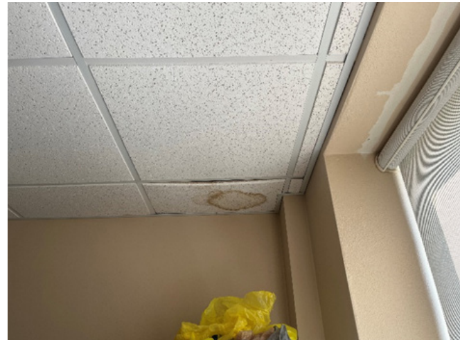
Damaged ceiling tile – adjacent to IT room
