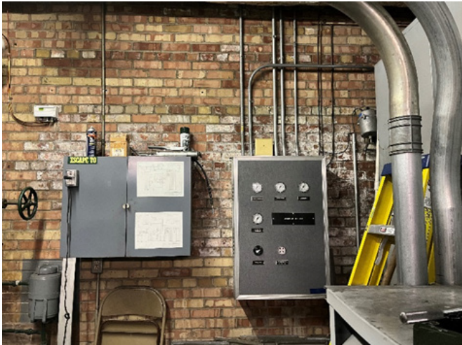
Efflorescence on west wall
