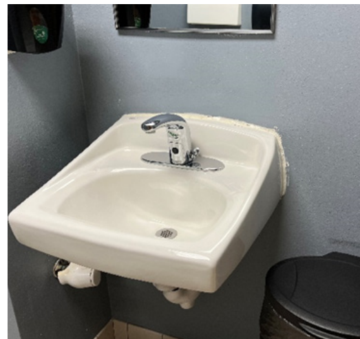
Excessive sealant at lavatory
