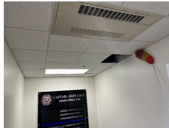
Missing ceiling tile at back stair shaft
