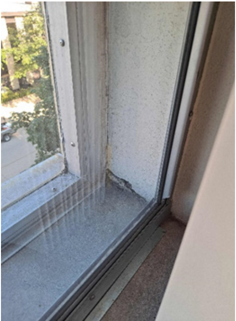
Rust on window well walls
