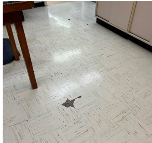
Chipped floor tile
