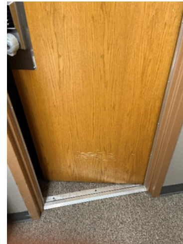
Scratched wood door
