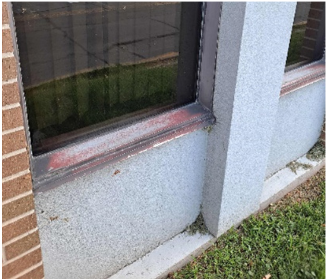
Faded metal window trim
