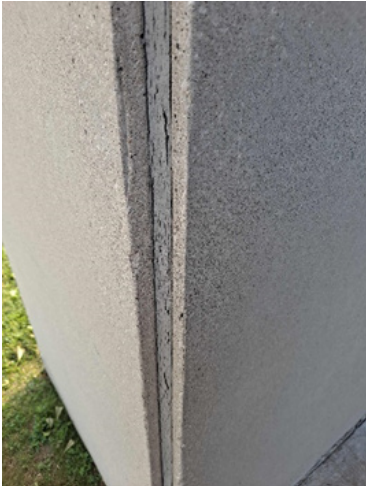
Caulking dried and brittle
