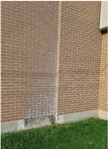
Efflorescence on brick
