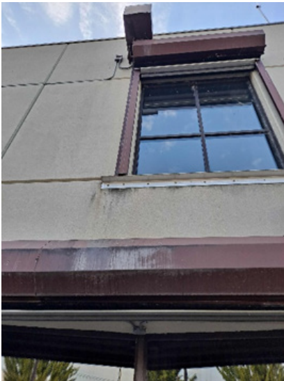
Window housing faded and rusting
