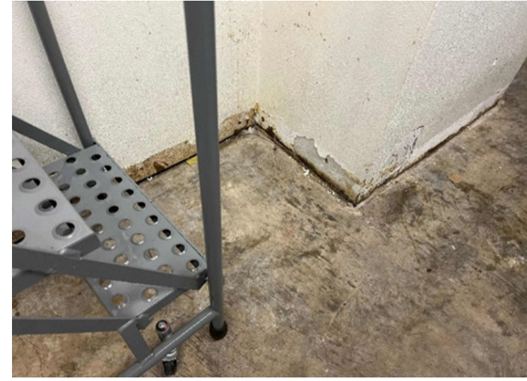
Deteriorated base at high-density storage
