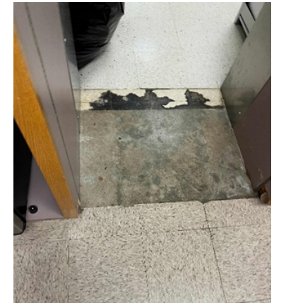
Missing VCT at basement
