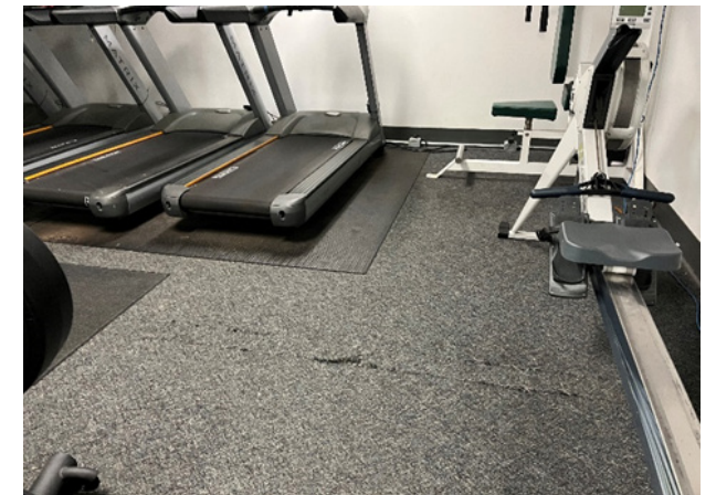
Ripped carpet at cardio room
