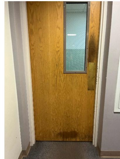
Damaged wood veneer & missing kick plate
