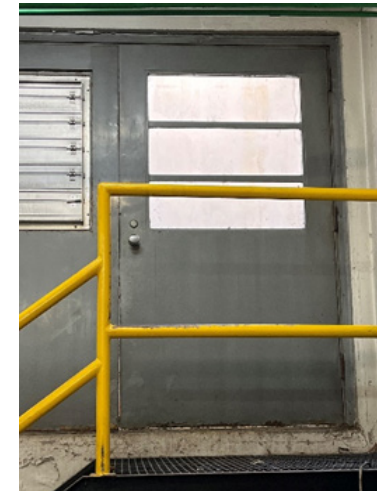
Missing weatherstripping at rusted door
