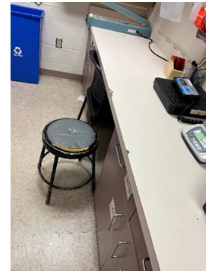
Plastic laminate casework condition
