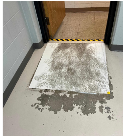
Chipped paint at shooting gallery entry
