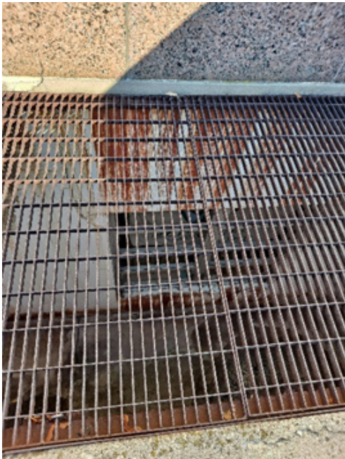
Rust on window well walls
