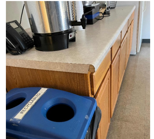
Chipped plastic laminate
