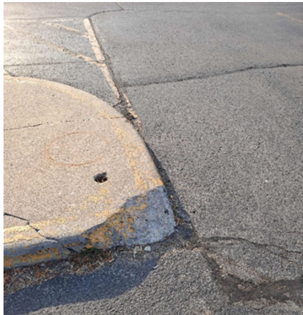
Damaged concrete curb
