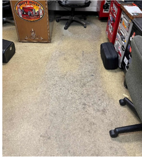
Worn VCT at shop office
