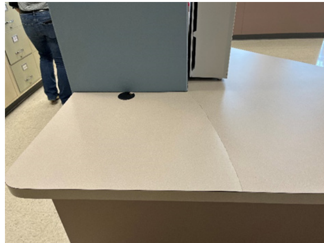
Cracked, damaged plastic laminate
