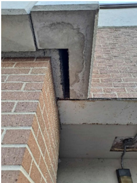
Gaps under precast concrete panels
