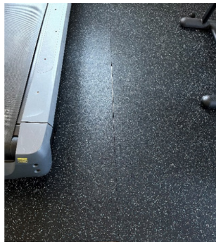
Gap in rubber floor tile
