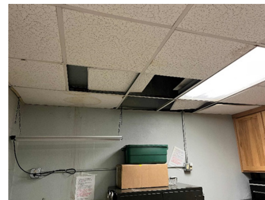
Missing and misplaced ceiling tiles
