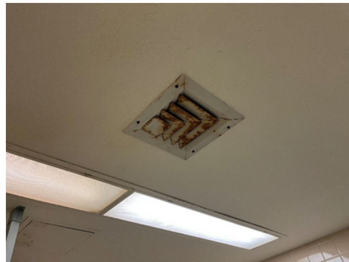
Rusted ceiling diffuser at basement toilet room
