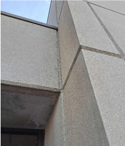
Caulking dried and brittle
