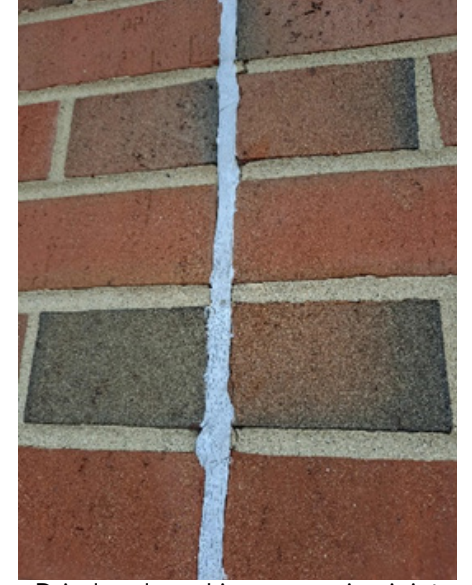
Dried and cracking expansion joint material
