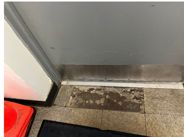
Missing vinyl tile at back door
