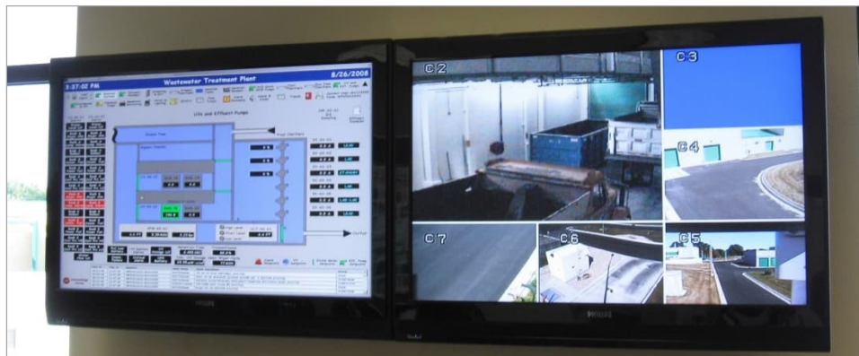
Fond du Lac WPCF SCADA and Security 47-inch LCD monitors.
