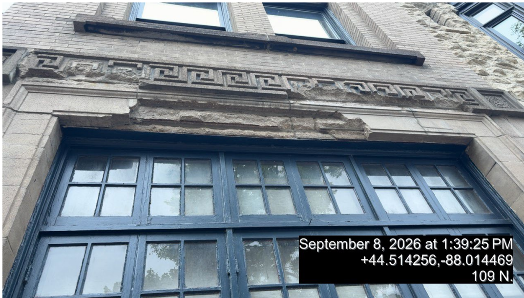
Existing condition detail - deterioration at decorative band above window opening.
