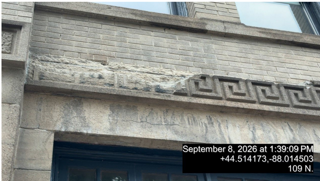
Existing condition detail - localized loss at decorative Greek-key band.
