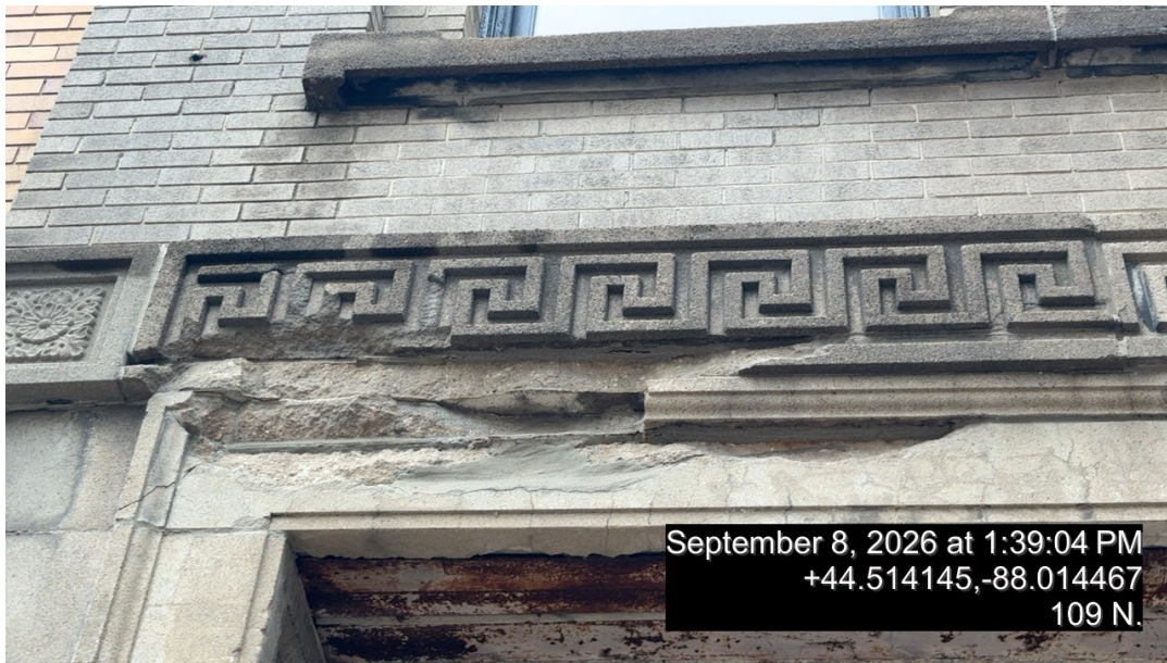
Existing condition detail - localized deterioration at decorative facade band.
