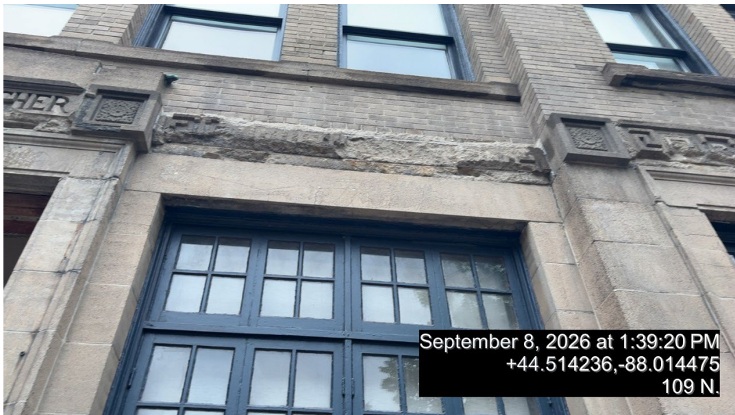
Existing condition detail - deterioration above window opening.
