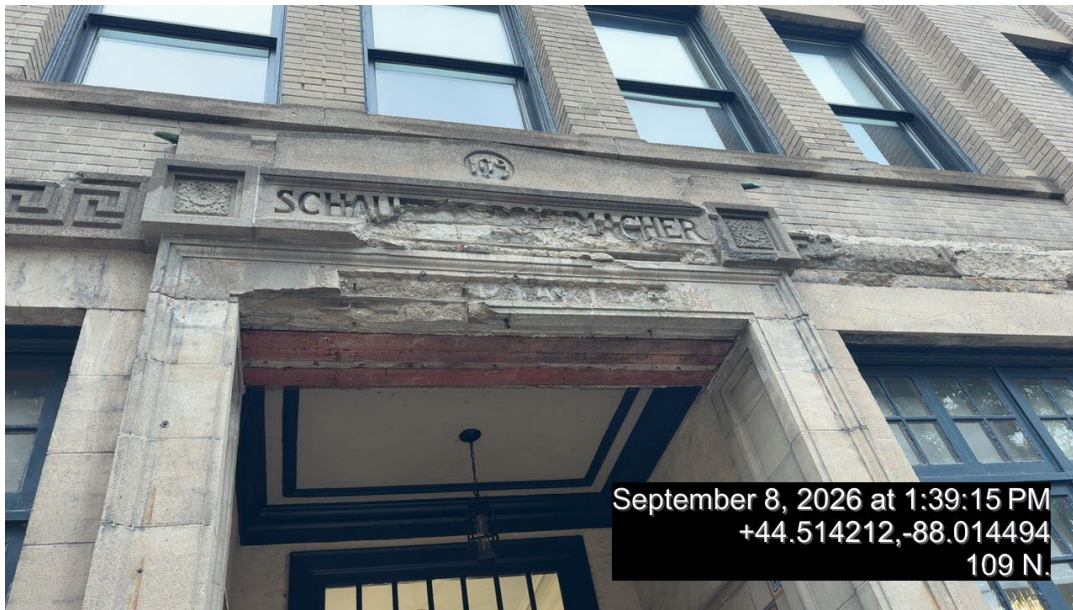
Existing condition detail - deterioration at central entrance surround and adjacent facade band.
