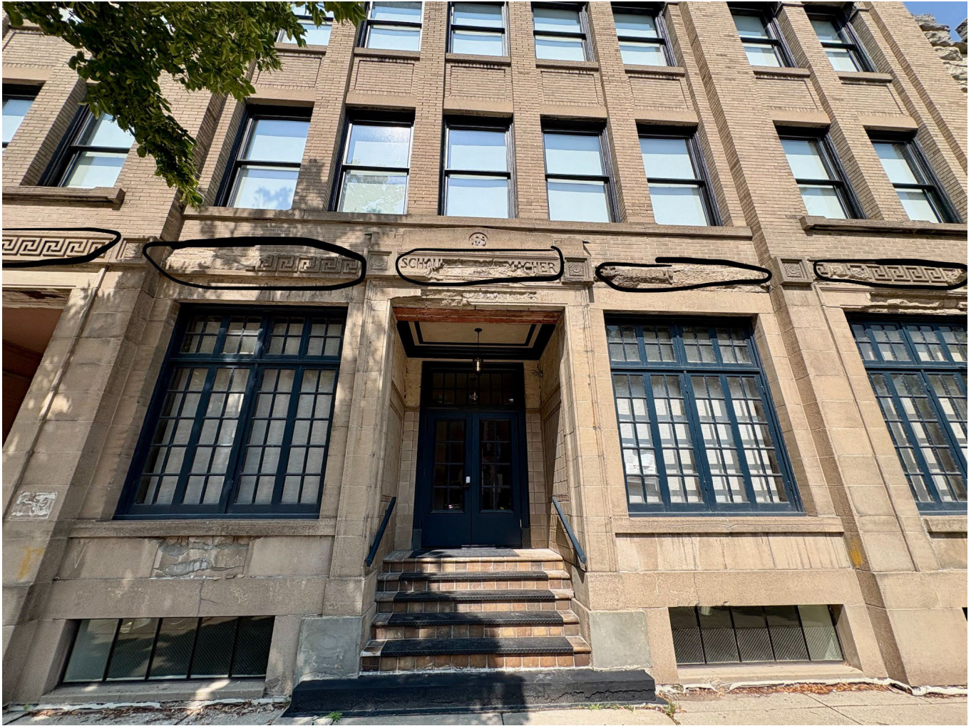
Existing facade - front elevation with areas of deterioration identified.
